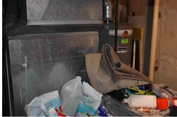
FURNACE / WATER HEATER
