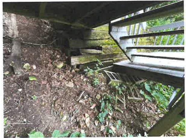
Photo 6 – Retaining Wall 1, East Corner Deterioration
