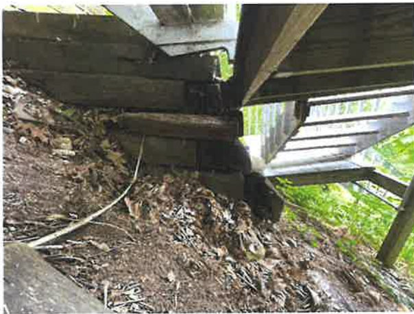
Photo 5 – Retaining Wall 1, East Corner Deterioration
