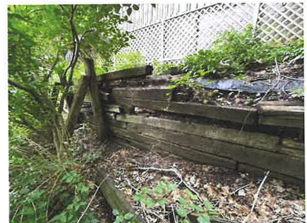
Photo 15 – Retaining Wall 2, Deterioration at West End
