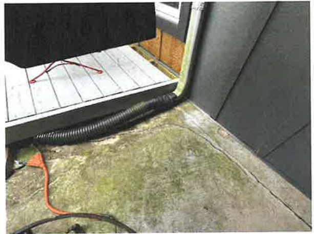
Photo 18 – Condition D, Southeast Corner of Patio
