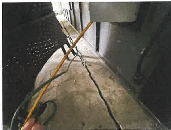
Photo 19 – Condition D, Along South End of Patio
