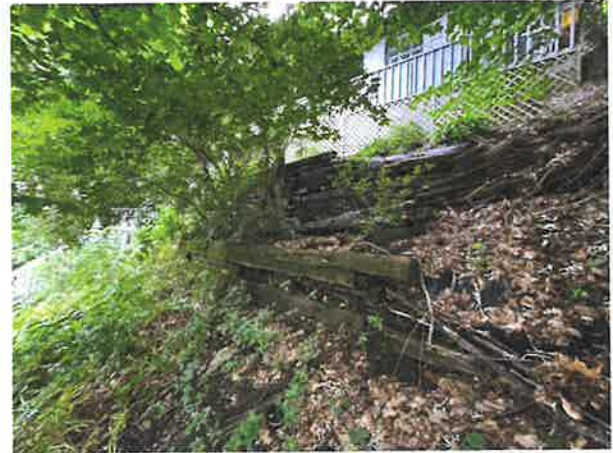
Photo 8 – Retaining Wall 1, West End Deterioration
