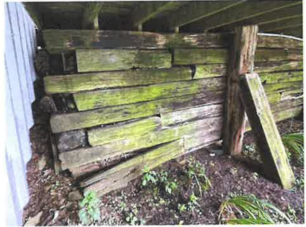
Photo 11 – Retaining Wall 2, East Corner Deterioration
