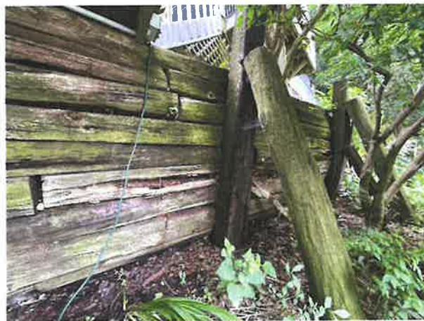
Photo 12 – Retaining Wall 2, Deterioration and Leaning Support
