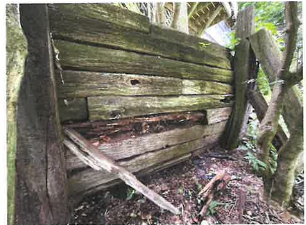
Photo 13 – Retaining Wall 2, Deterioration and Bowed Support
