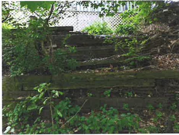
Photo 7 – Retaining Wall 1, West End Deterioration
