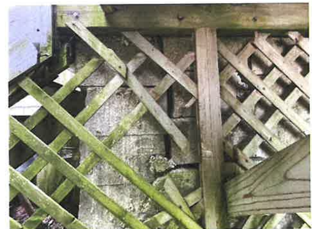
Photo 22 – Condition G, One Example
