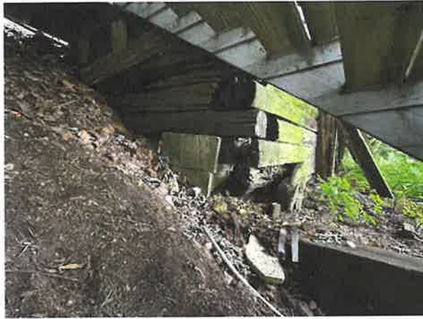
Photo 10 – Retaining Wall 2, East Corner Deterioration
