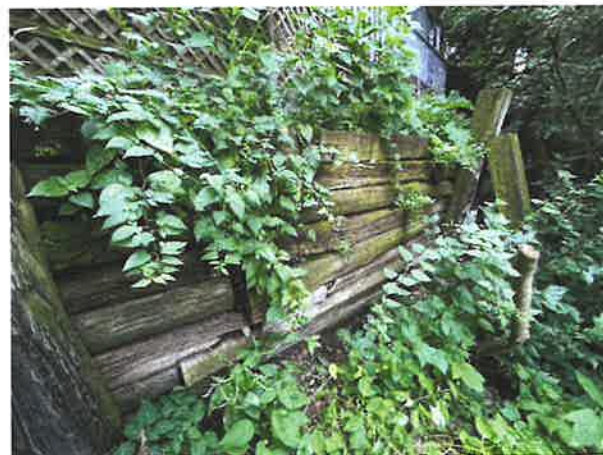
Photo 14 – Retaining Wall 2, Deterioration and Leaning Support
