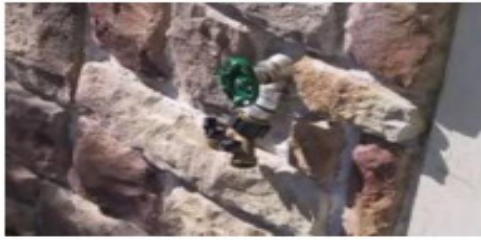
Outside Tap located near patio
