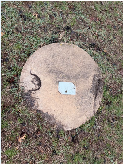
Missing locking device
