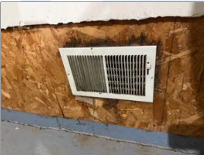
Heat register improperly terminated through the fire separation
