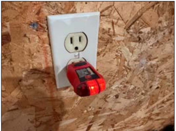
Missing GFCI protection for the garage
