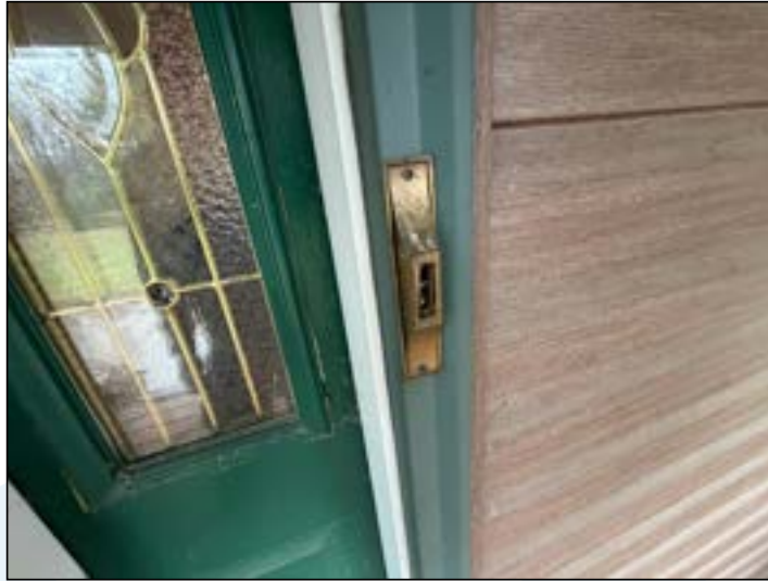
Broken doorbell button
