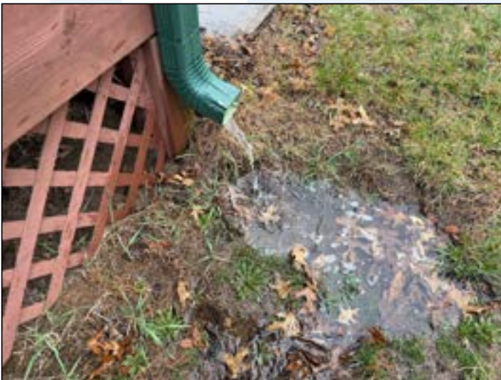
Missing down spout extensions
