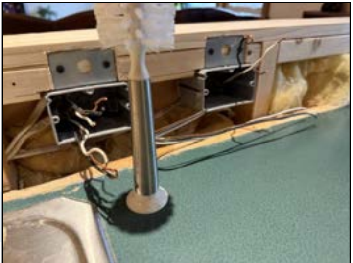
missing receptacles on the kitchen countertop from remodel
