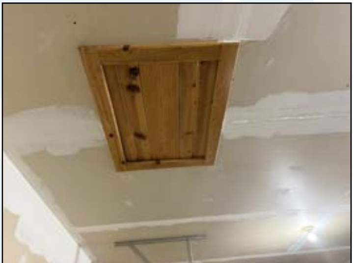
Access to the attic was not fire rated
