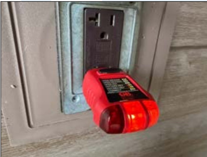
GFCI function would not trip
