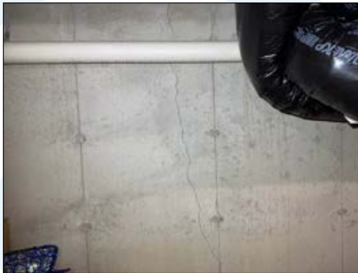
Shrinkage cracking observed
