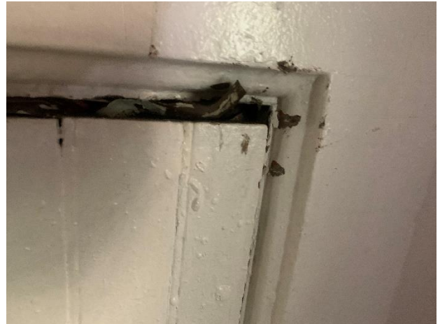
Door, Door Casing Back Entry Side B-Hatch
