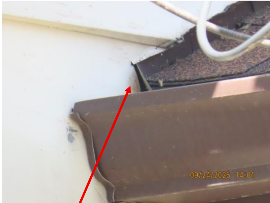
Kick out flashings were observed
