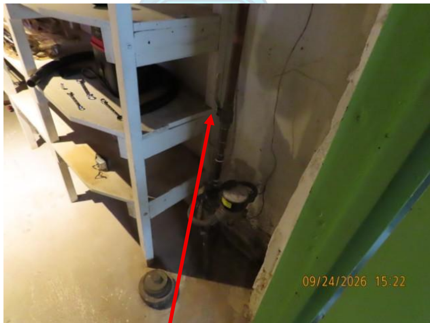
Main water shutoff
