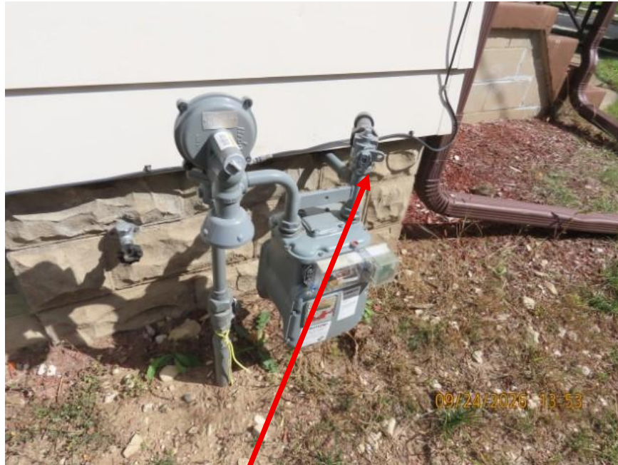
Main gas shutoff
