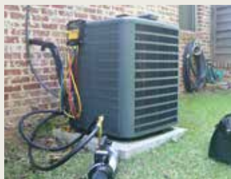
Pre-season HVAC tune ups
