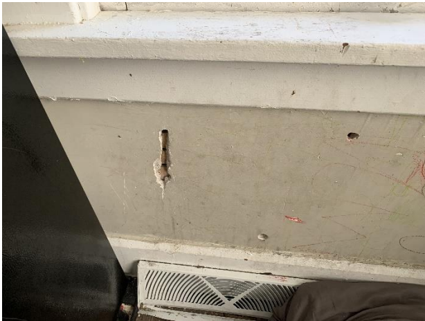
Wall Kitchen Side C
