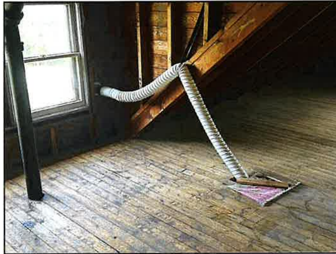
89. Not insulated in unconditioned space
