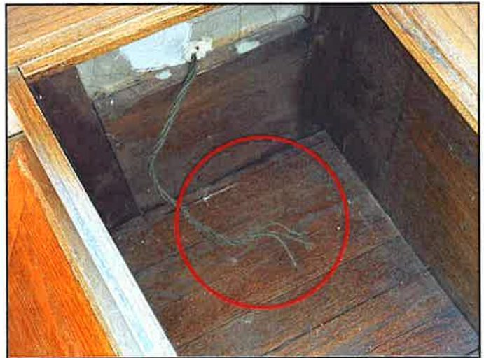
49. Exposed wires should be installed inside
