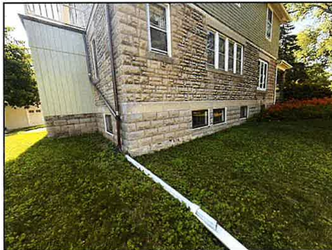
31. Improper slope or drainage
