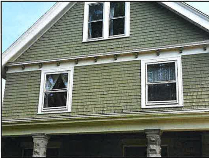
22. Peeling paint and wood rot
