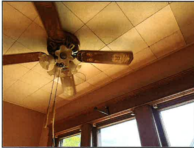
78. Moisture staining, appears to be old. Wa
