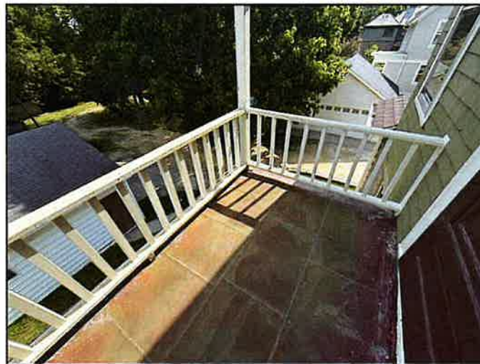
28. Guardrail is not to today's standard
