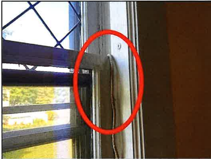
84. Broken sash cord/spring
