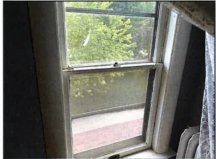
85. Broken sash cord/spring
