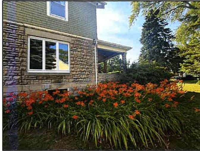
30. Trees or shrubs too close to building
