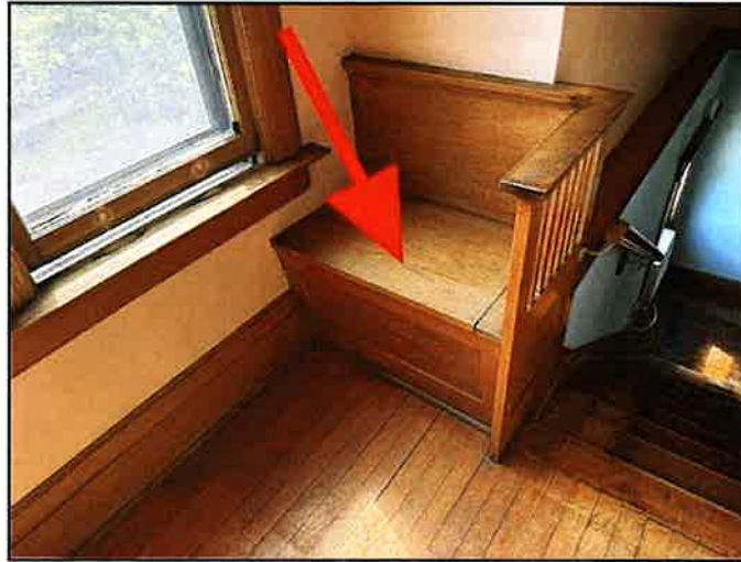
50. Exposed wires should be installed inside
