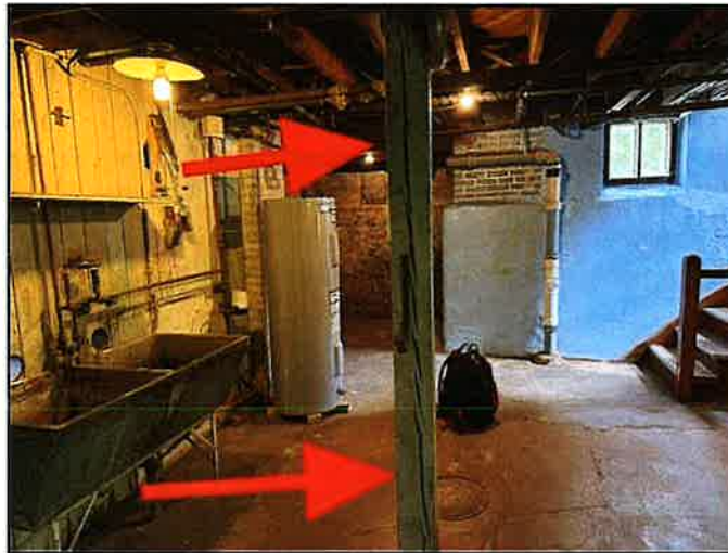
34. Cracks on wood columns. These are normal
