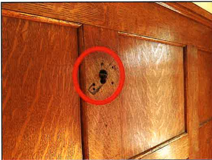
48. Exposed wires should be installed inside
