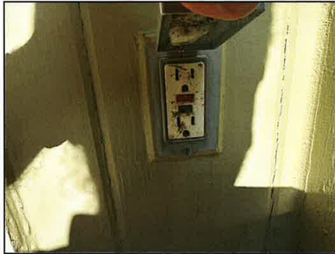
57. Test faulty on GFCI/GFI (Ground Fault Ci
