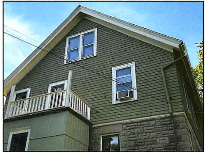
23. Peeling paint and wood rot
