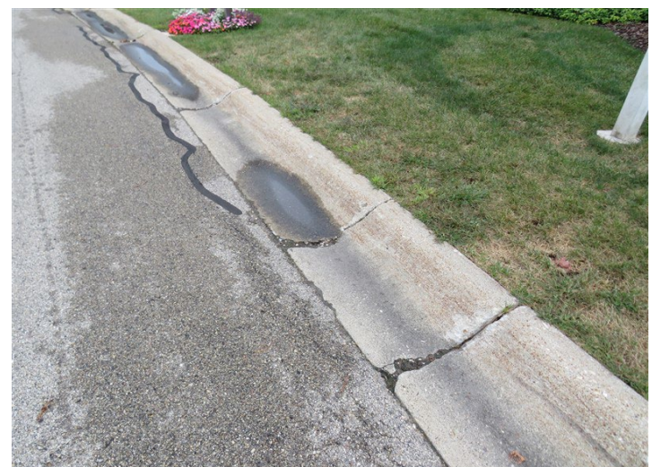
cracks and concrete deterioration
