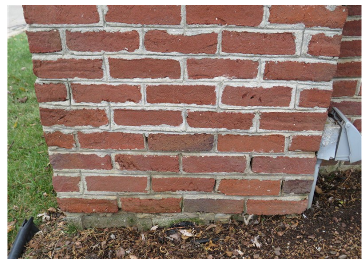
mortar deterioration and prior repairs
