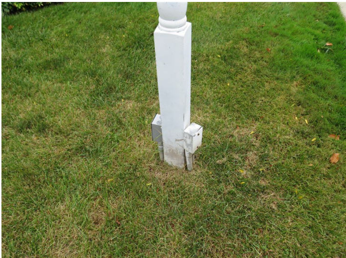
wear at base of pole from lawn care equipment
