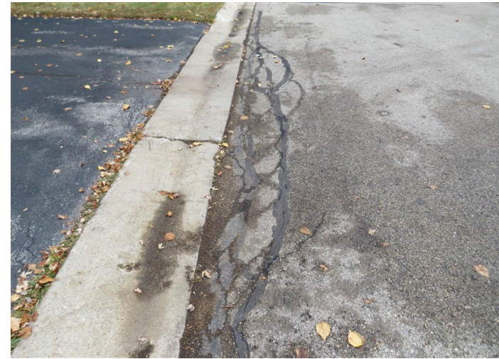
repaired and unrepaired cracks
