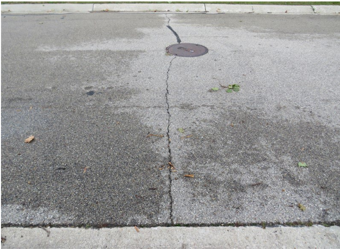
crack at street
