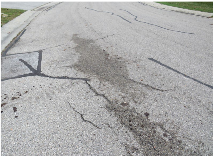
repaired and unrepaired cracks
