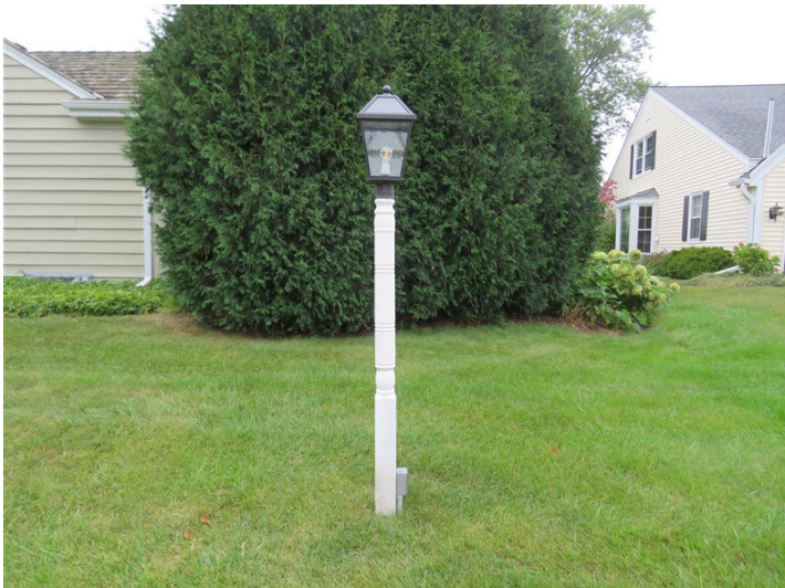
composite light pole with metal light fixture
