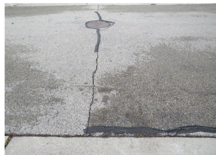
crack at pavement
