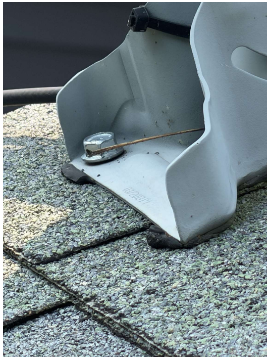
Photo 10. Roof-mounted satellite attachment and surrounding shingles.
