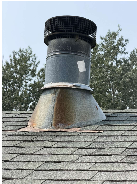
Photo 1. Metal roof vent/chimney assembly showing visible rust and corrosion.
