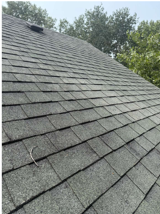
Photo 8. Shingle field showing general surface wear and weathering.
