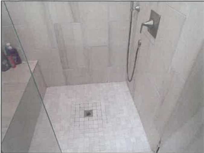
223. Grout loose, missing or deteriorated
