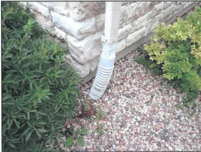
67. Discharge below grade
