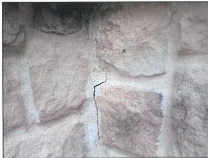
89. Missing, ineffective weep holes or flashings
