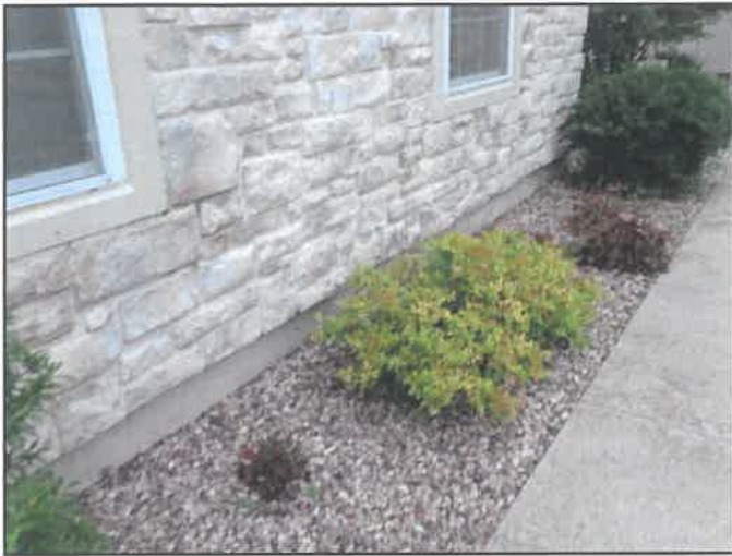
83. Missing, ineffective weep holes or flashings
