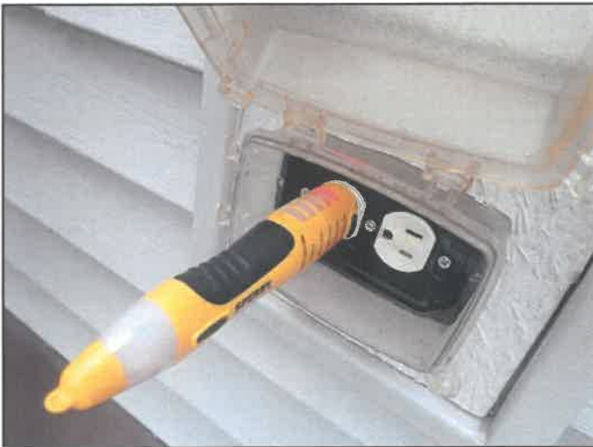
123. Test faulty on GFCI/GFI (Ground Fault...
