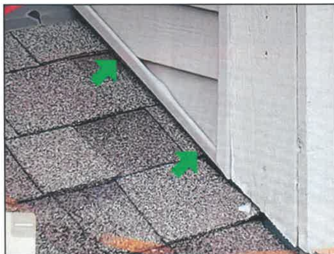
51. Siding not cut back
