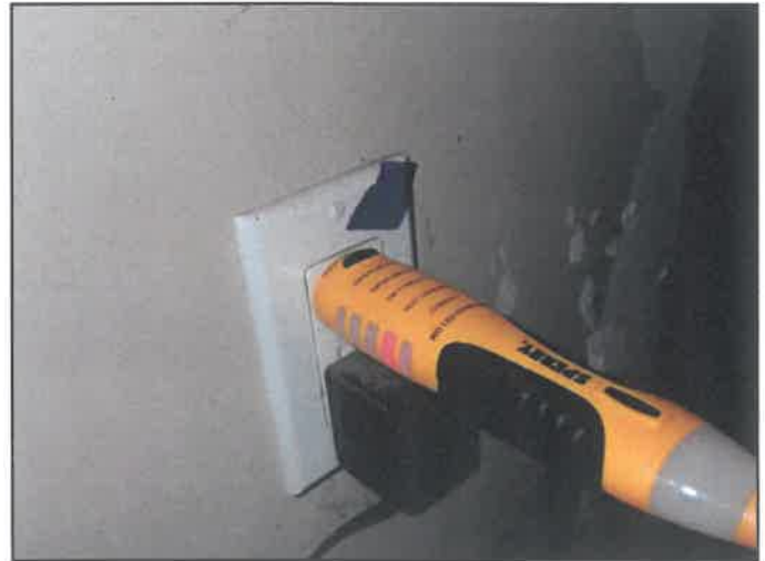
124. Test faulty on GFCI/GFI (Ground Fault...
