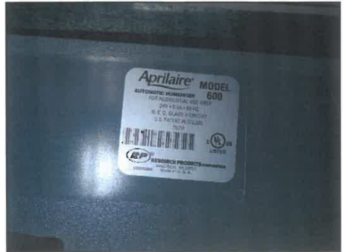
165. Duct mounted bypass humidifer
