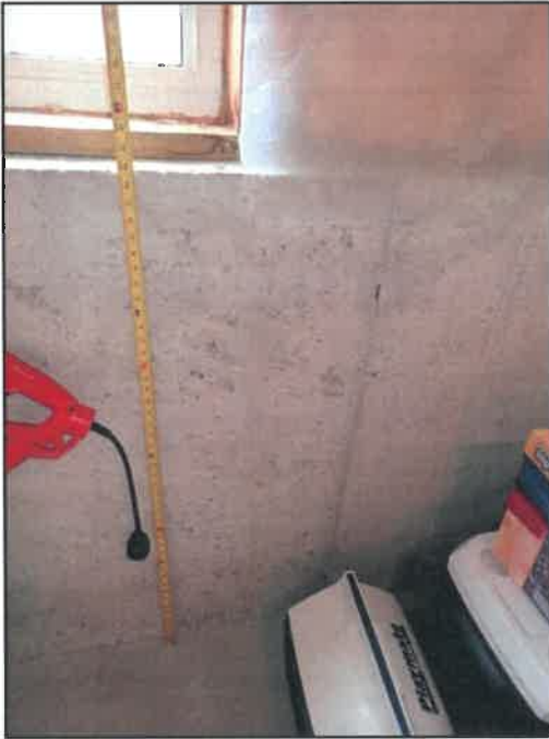
239. not proper egress measurement
