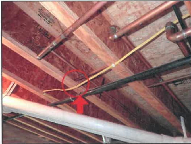
18. Not well secured
