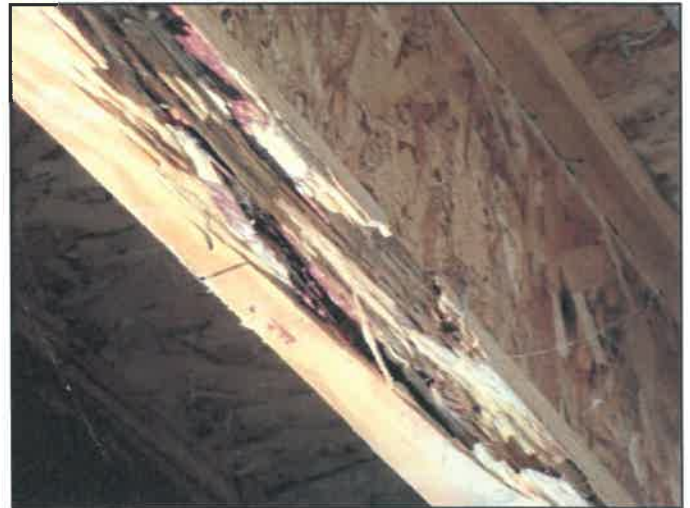
108. Split or damaged
