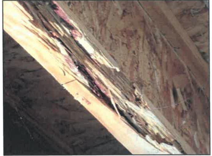
17. Split or damaged
