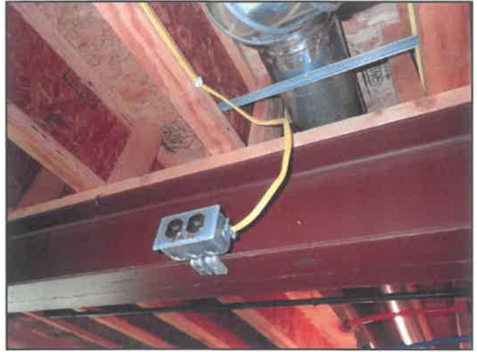
122. Not well secured
