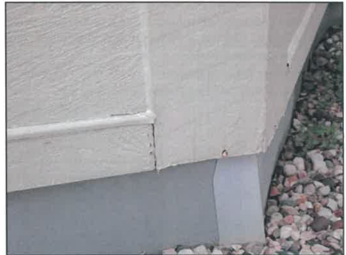
80. Paint or stain needed
