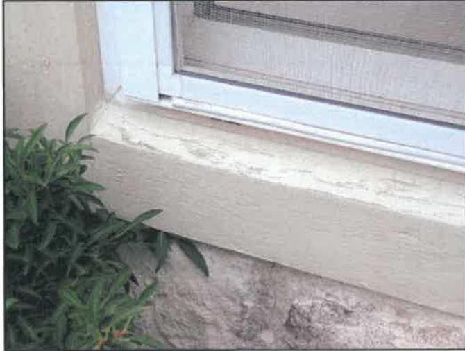
77. Paint or stain needed
