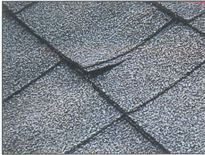
47. Missing, loose or torn
