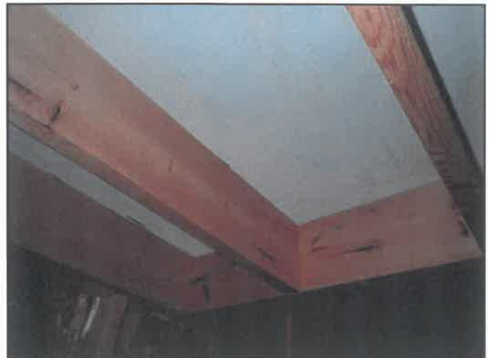
105. Poor end bearing, joist hanger connections
