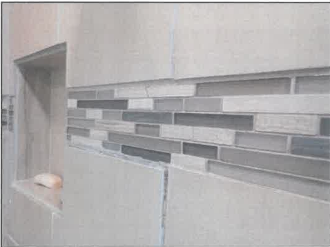
225. Grout loose, missing or deteriorated
