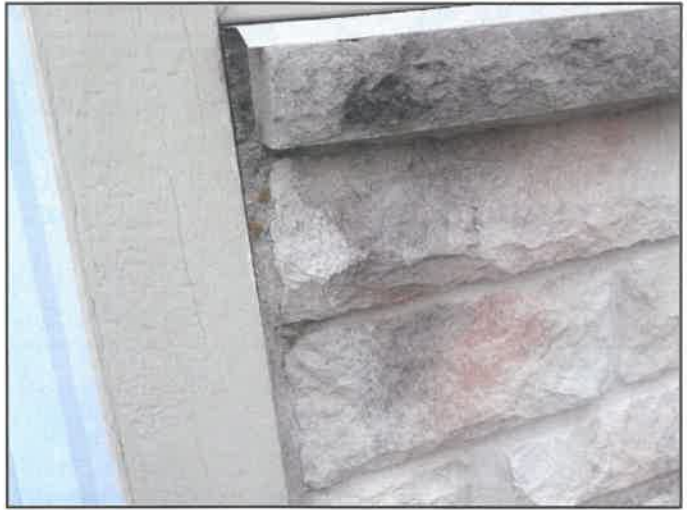
84. Missing, ineffective weep holes or flashings
