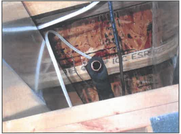
178. Not well secured
