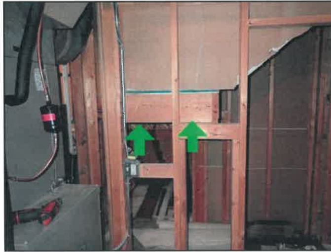
106. Poor end bearing, joist hanger connections
