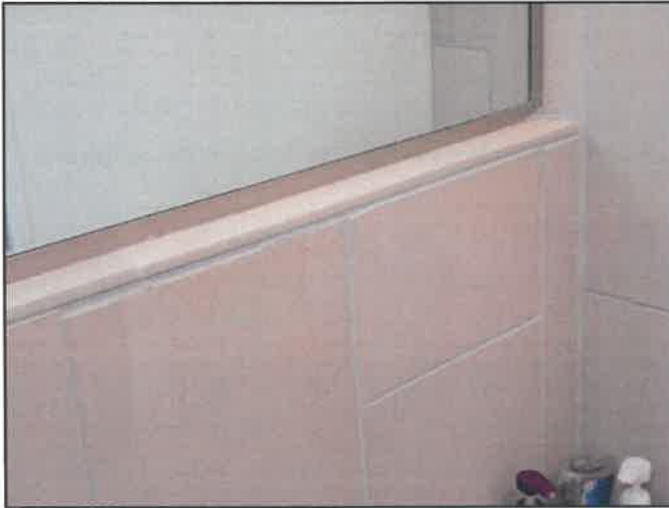
25. Grout loose, missing or deteriorated
