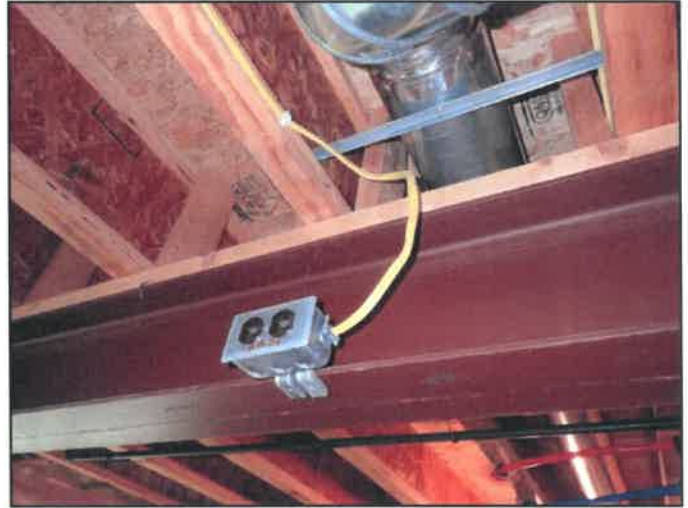
19. Not well secured
