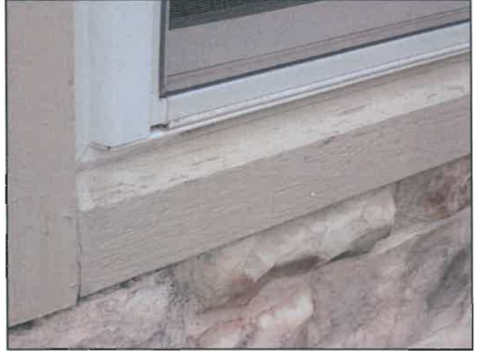
78. Paint or stain needed
