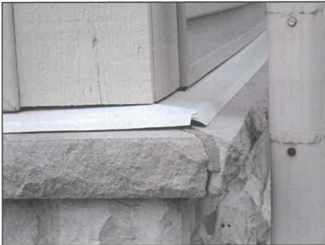
85. Missing, ineffective weep holes or flashings
