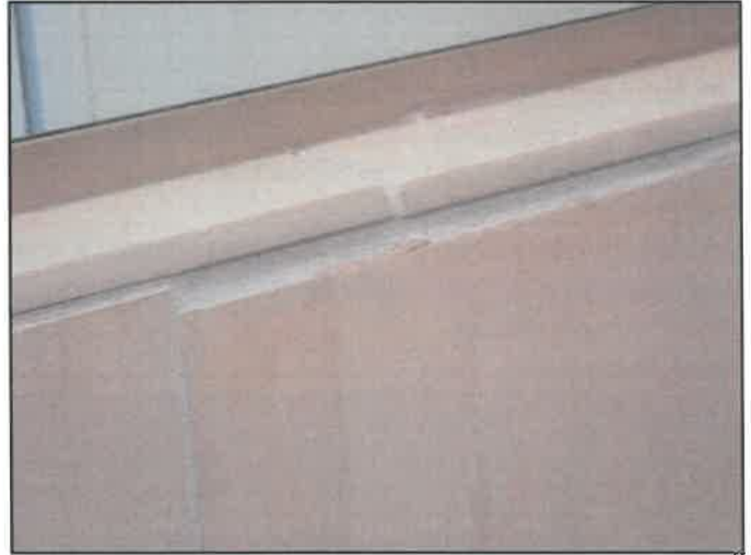
26. Grout loose, missing or deteriorated
