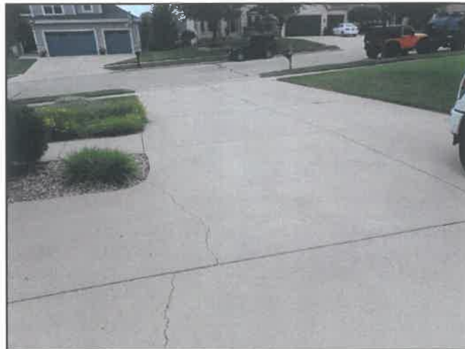
56. Cracked or damaged surfaces
