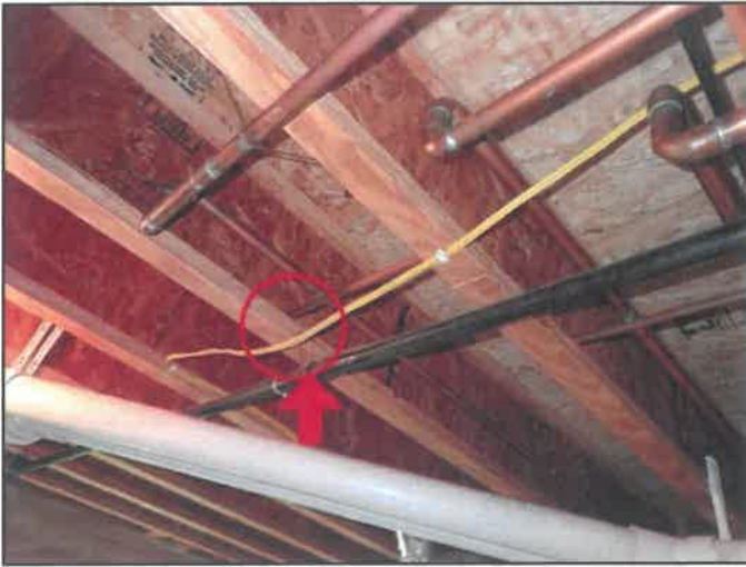
121. Not well secured
