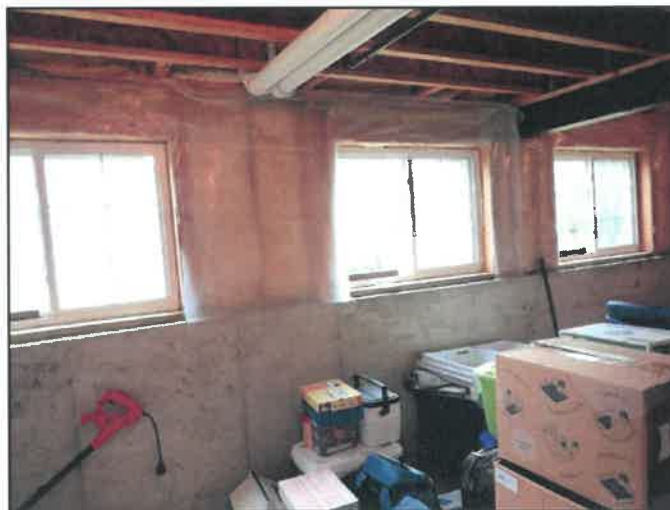
241. not proper egress measurement
