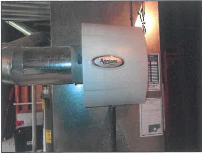
162. Duct mounted bypass humidifer
