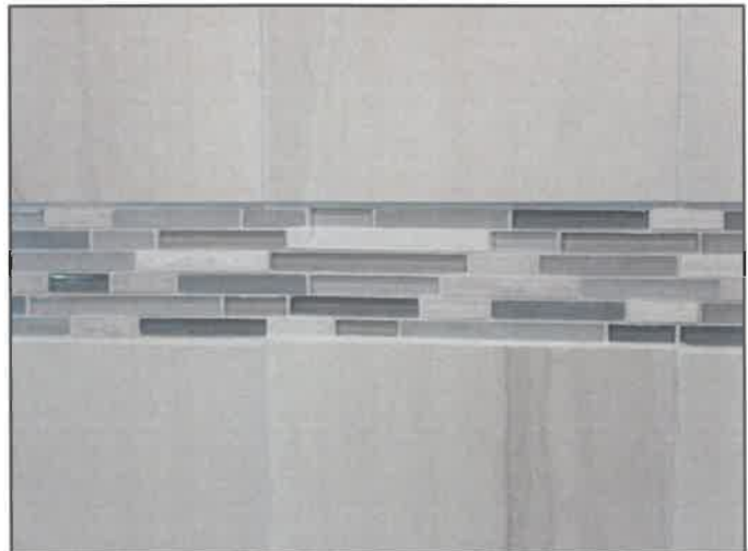
24. Grout loose, missing or deteriorated
