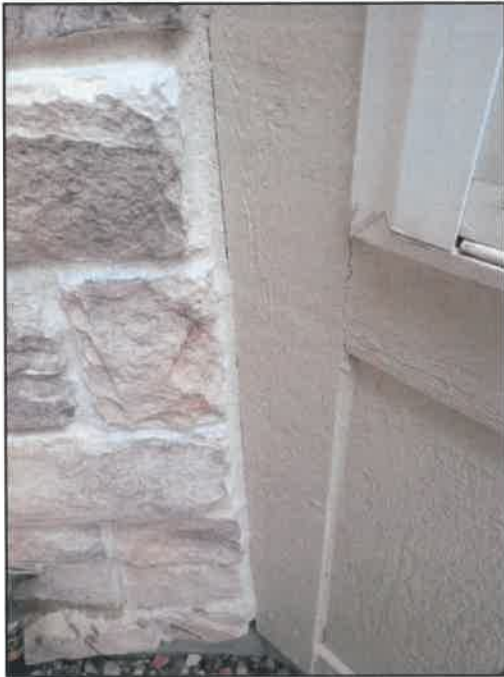
87. Missing, ineffective weep holes or flashings
