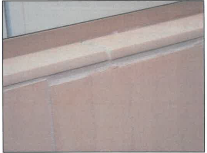
228. Grout loose, missing or deteriorated
