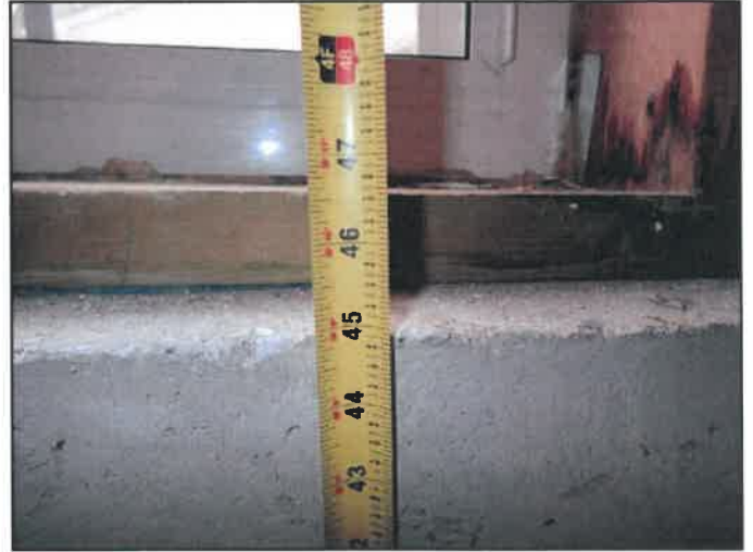
240. not proper egress measurement
