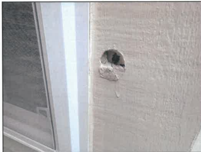
79. Paint or stain needed
