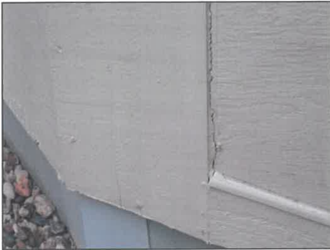
81. Paint or stain needed
