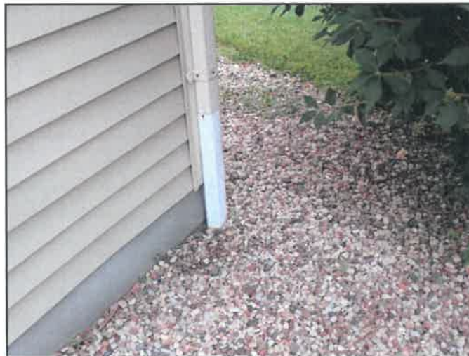
69. Discharge below grade
