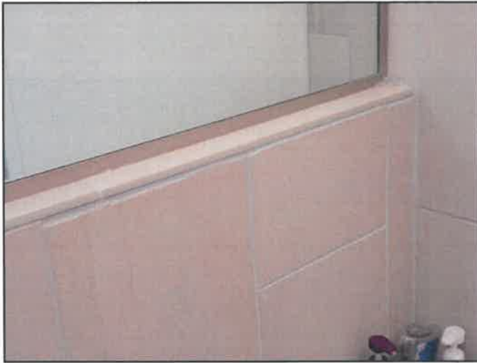
227. Grout loose, missing or deteriorated
