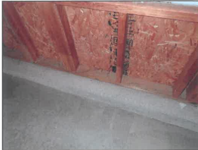
109. Bottom plates have poor bearing
