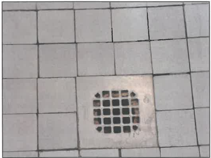
22. Grout loose, missing or deteriorated
