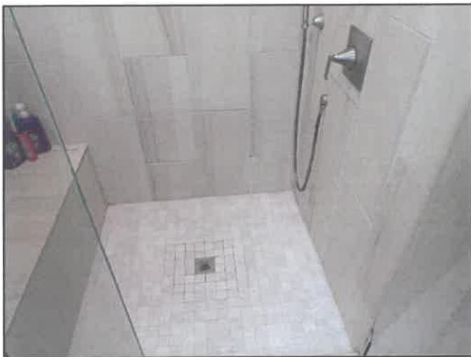
21. Grout loose, missing or deteriorated
