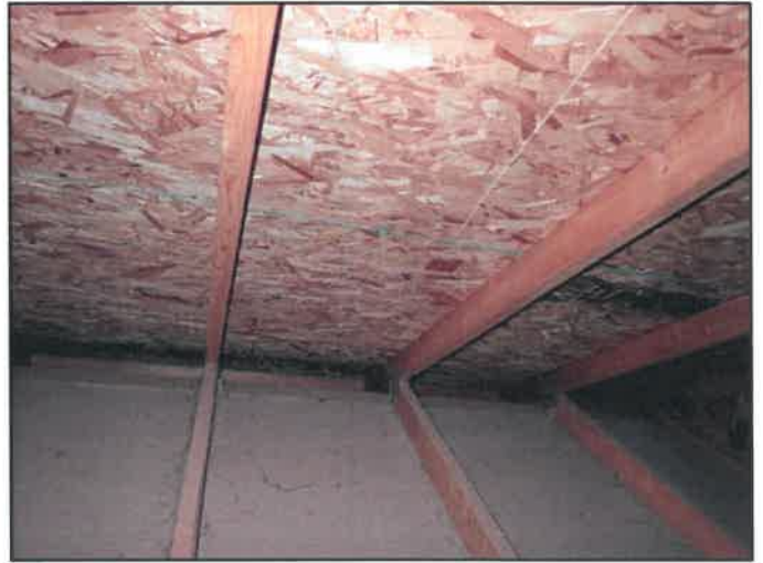
200. Amount inadequate above garage
