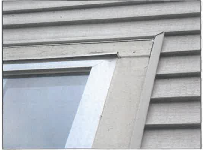
82. Paint or stain needed
