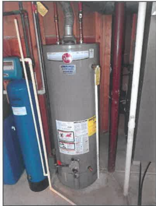
217. Service water heater
