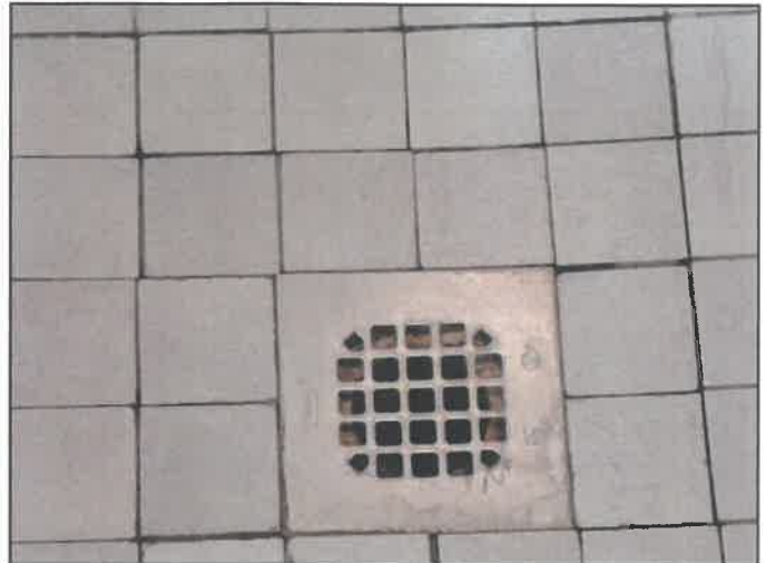
224. Grout loose, missing or deteriorated
