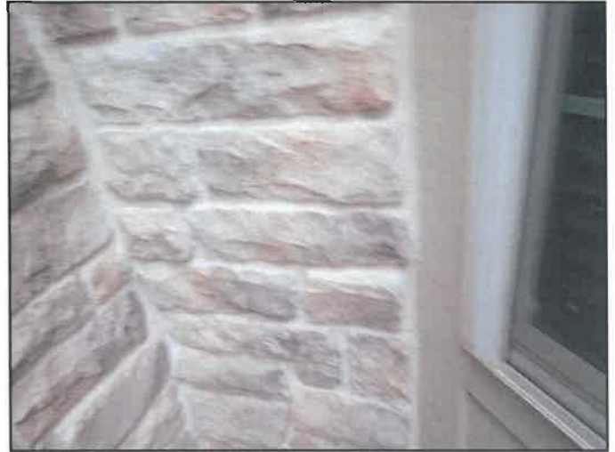
88. Missing, ineffective weep holes or flashings
