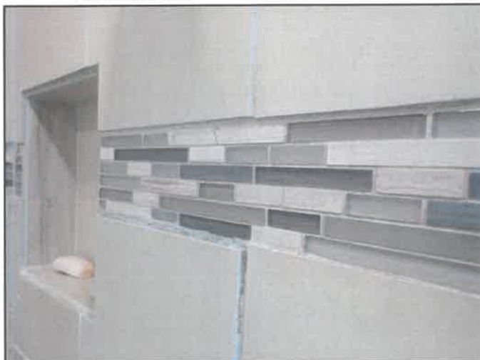
23. Grout loose, missing or deteriorated
