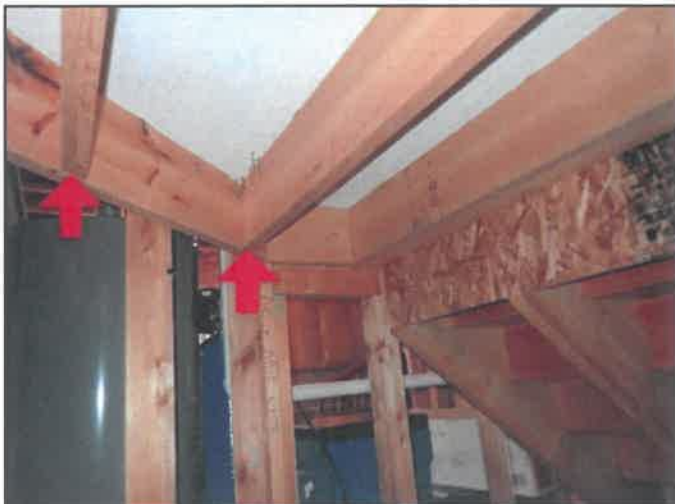
104. Poor end bearing, joist hanger connections
