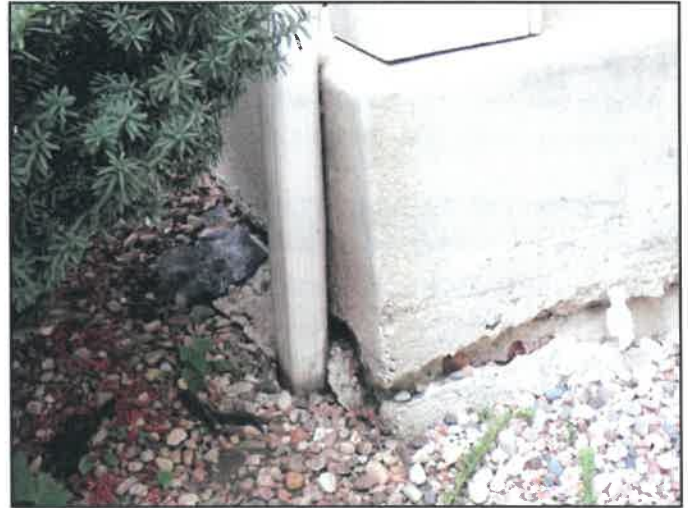
68. Discharge below grade
