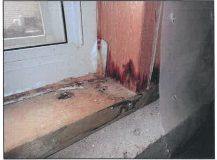
237. signs of moisture interior window trim
