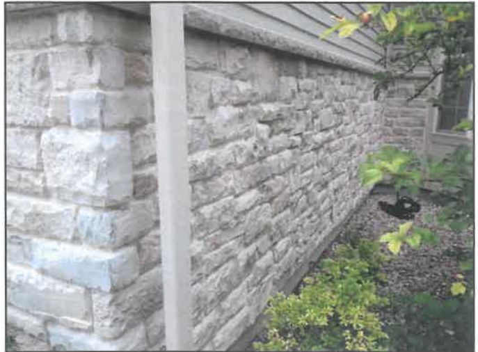
86. Missing, ineffective weep holes or flashings
