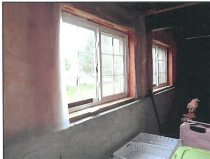
238. window flashing missing
