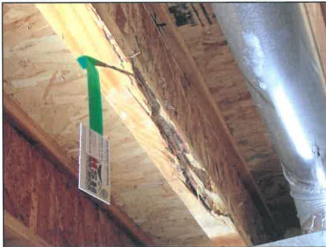
107. Split or damaged
