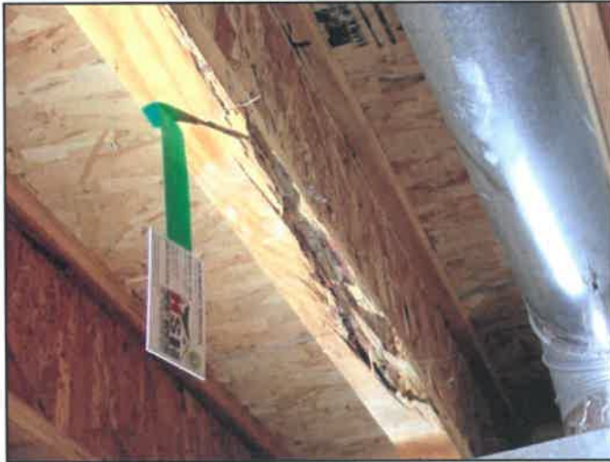
16. Split or damaged
