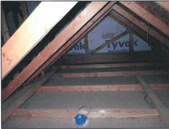
199. Amount inadequate above garage
