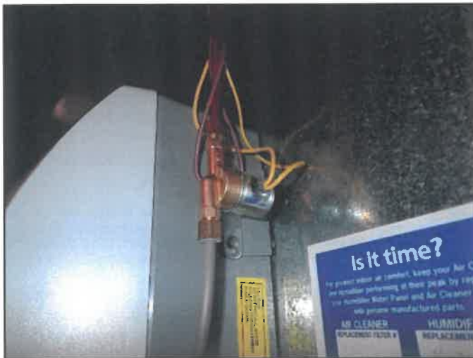
164. Duct mounted bypass humidifer
