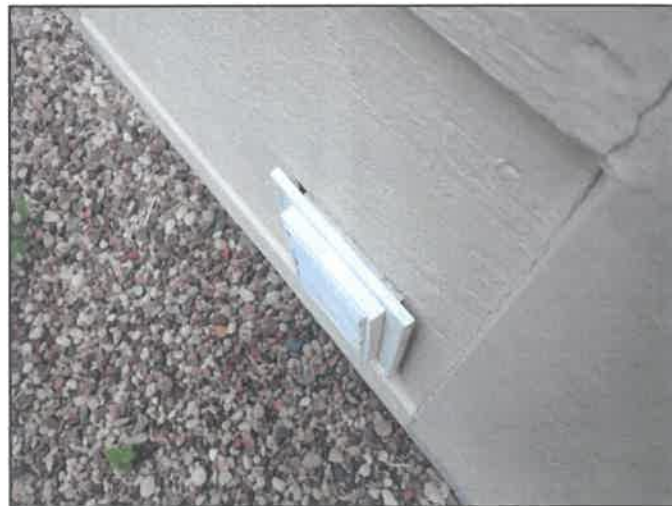
76. Caulking missing or deteriorated
