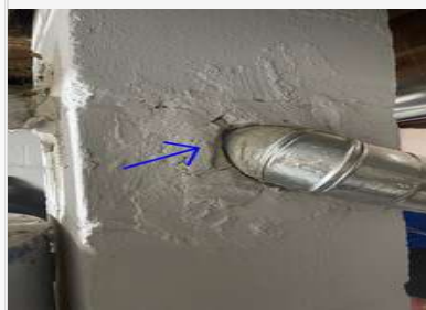
13.2.1.2 Keep areas sealed where flues enter chimney
