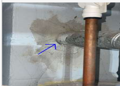
13.2.1.1 Keep areas sealed where flues enter chimney
