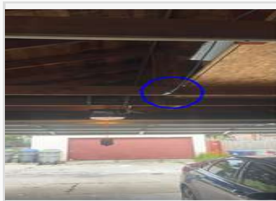
4.1.1.1 Extension cord wiring is not intended for permanent use
