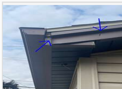
3.7.1.2 Trim rigatoni trim and one or more nails popped
