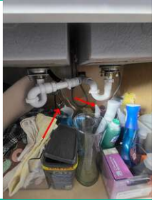
1.1 Pex piping loosely attached
