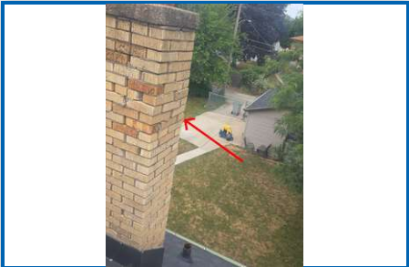
1.2 Repair any damaged/open joints at chimney
