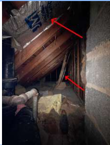
1.1 Insulation at roof sheathing not needed
