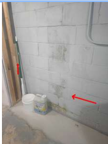
1.3 Minor efflorescence stains keep up with exterior grade and extend downspouts where needed
