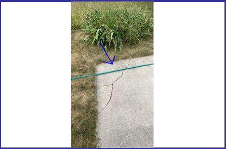
1.2 Seal cracks as needed
