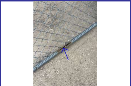
1.1 Fence showing wear/rust
