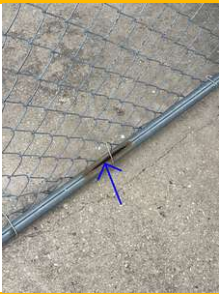
1.1 Fence showing wear/rust
