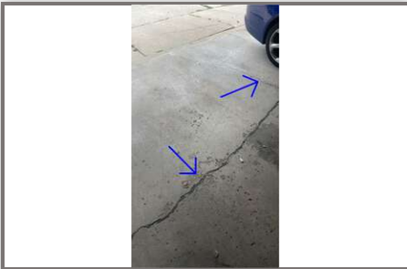
1.1 Seal cracks/flooring as needed
