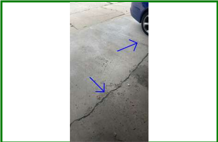
1.1 Seal cracks/flooring as needed
