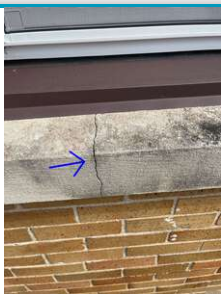
1.1 Seal cracks as needed
