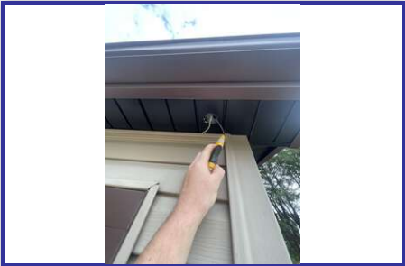
1.1 Properly cover/remove live wiring
