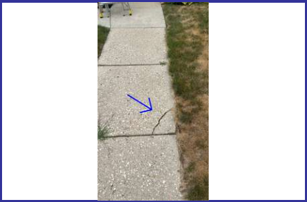
1.1 Seal cracks as needed
