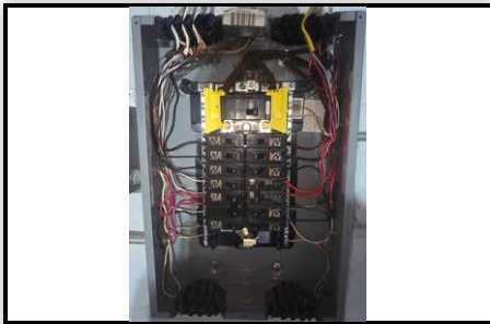
1.1 Electrical panel wiring
