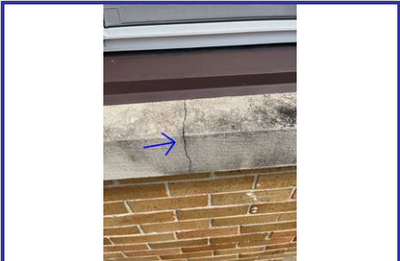
1.1 Seal cracks as needed
