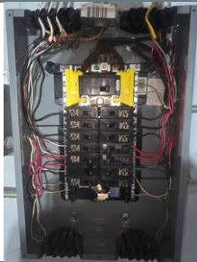
1.1 Electrical panel wiring
