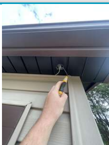
1.1 Properly cover/remove live wiring
