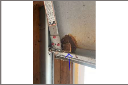
1.1 Damage to door
