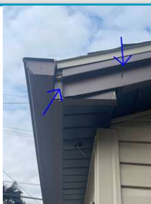
1.5 Trim sagging and one or more nails popped
