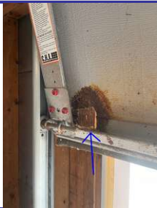
1.1 Damage to door
