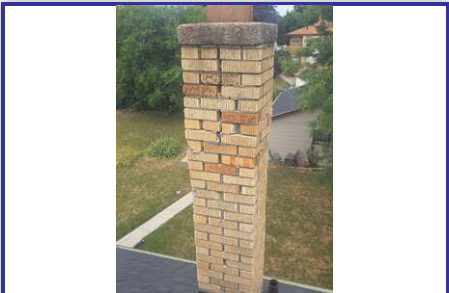
1.1 Repair any damaged/open joints at chimney
