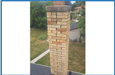
1.1 Repair any damaged/open joints at chimney
