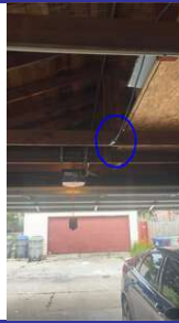
1.2 Extension cord wiring is not intended for permanent use
