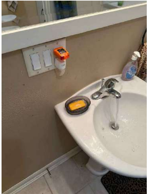
Mis-Wired Recommend GFCI Protection
