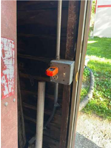
Recommend GFCI Protection
