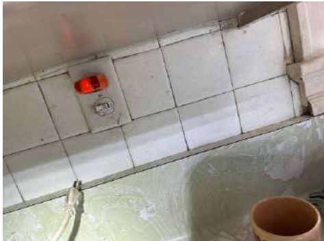
Mis-Wired Recommend GFCI Protection
