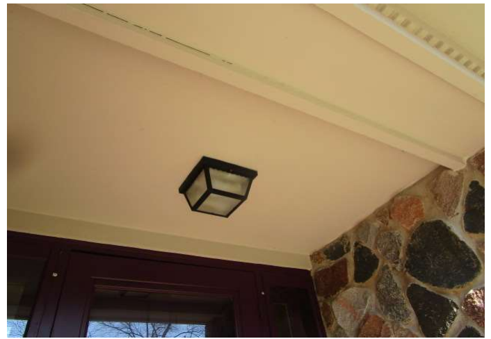
Soffit light fixture (non-typical)
