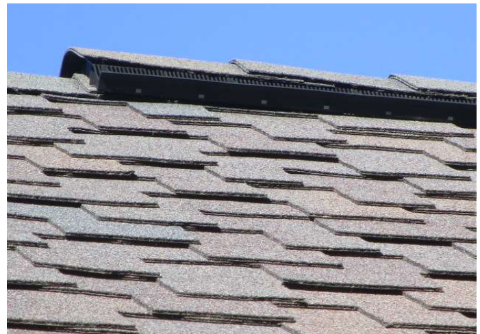
Ridge cap ventilation
