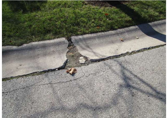
Damaged curb at Pinewood Court
