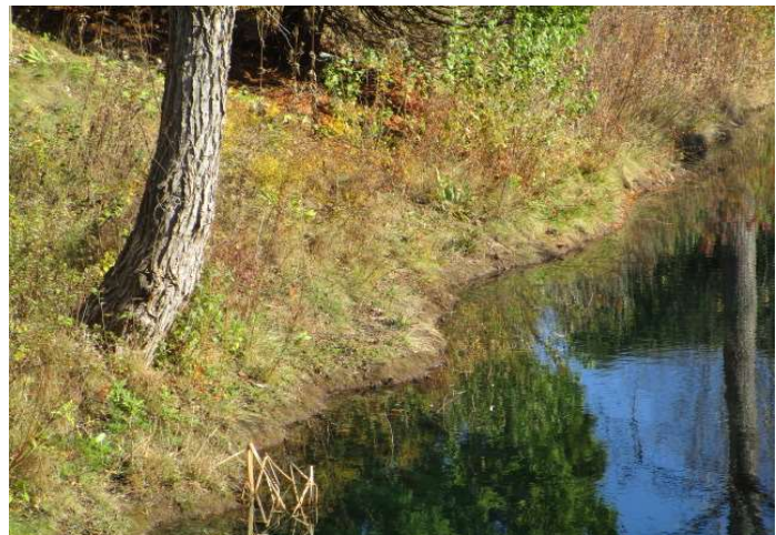
Erosion at the south pond
