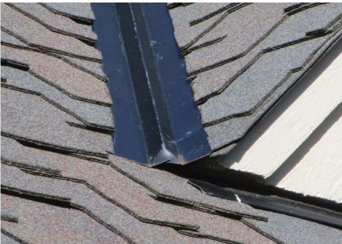
Metal valley flashing with small area of rust
