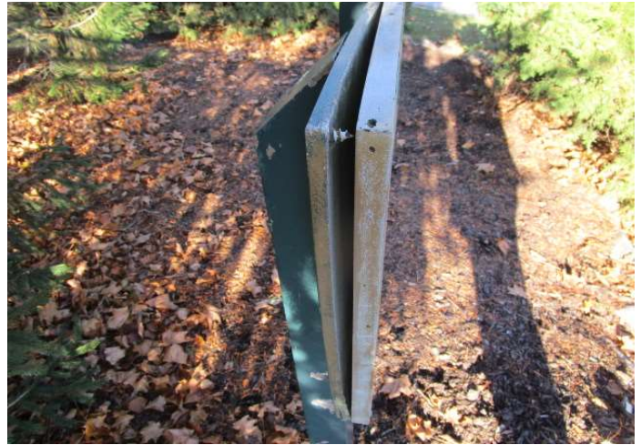
Delaminated signage components
