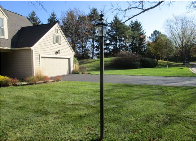
Typical light pole and fixture at a yard
