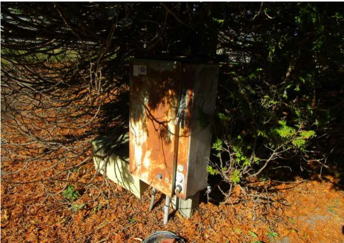
Aerator controller at the south pond
