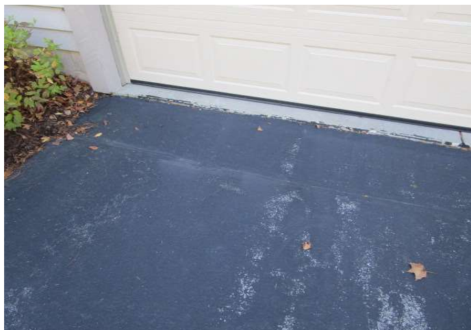
Settlement in the pavement along a garage floor
