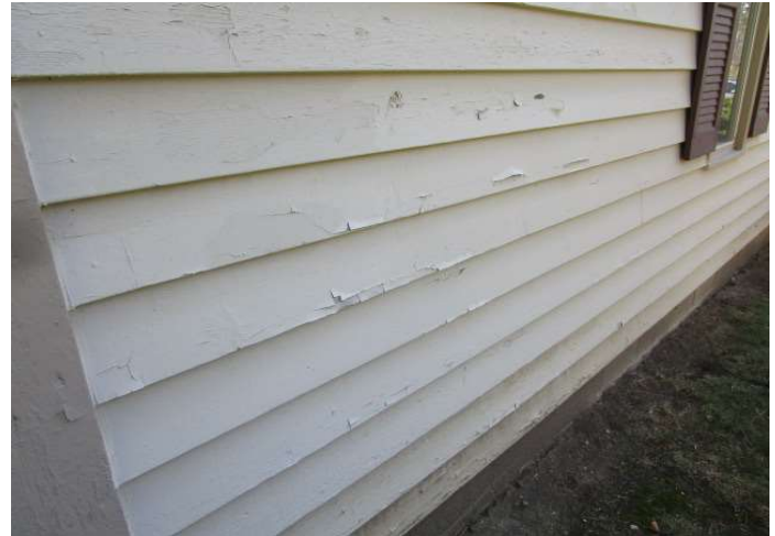
Flaking finish at siding and trim
