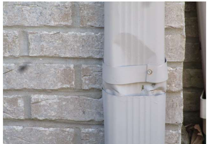
Instance of dented downspout
