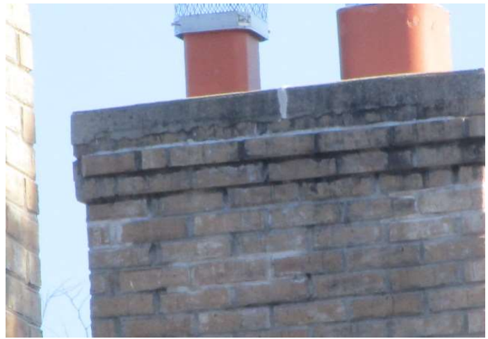
One of four masonry chimneys with staining and evidence of previous repairs
