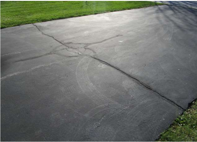
Driveway with open cracks
