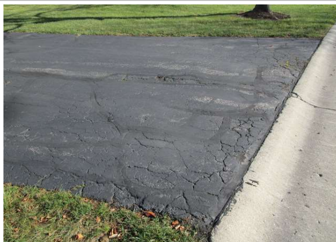
Deterioration at a driveway
