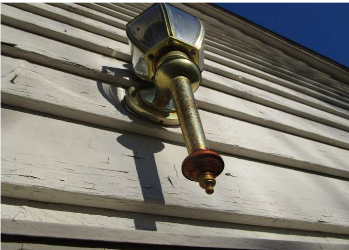
Alternative style large fixture over a garage with rust
