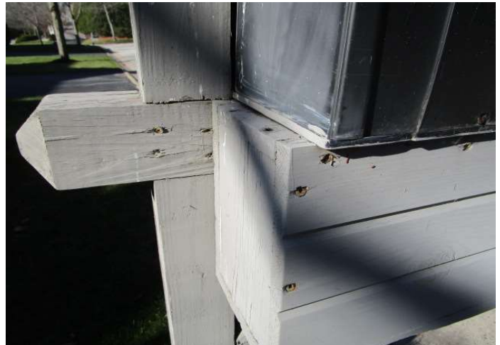
Painted wood components and fasteners
