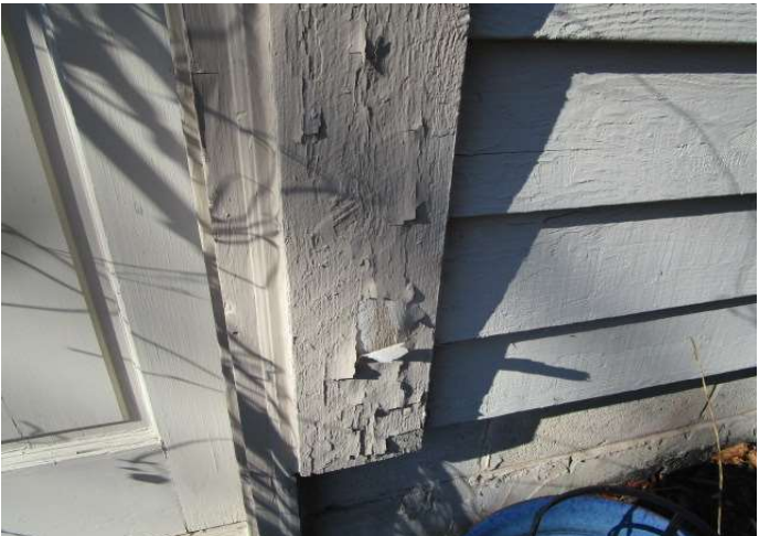
Flaking finish at trim
