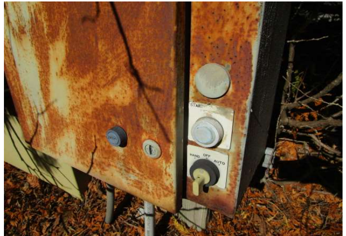
Aerator controller at the south pond
