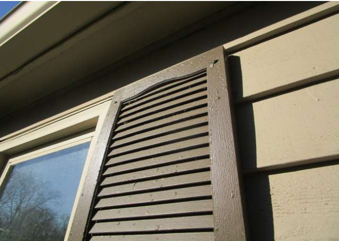
Shutter with blistering finish
