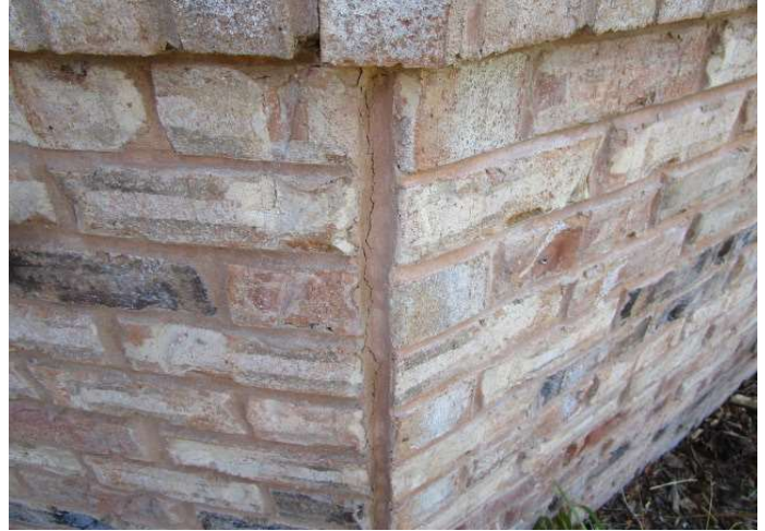
Common location of mortar crack at an outer corner
