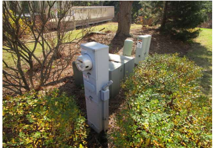
Electrical equipment near the north pond
