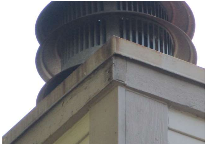
Detail view with some rust
