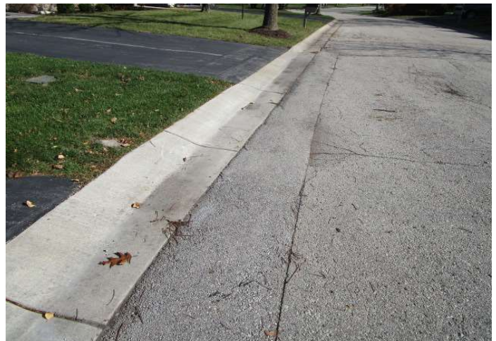
Previous patch along curb at Eastbrook Court
