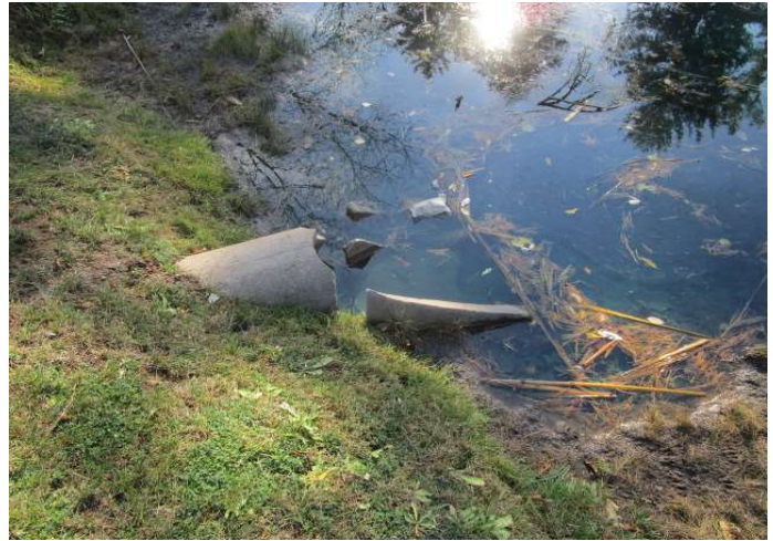
Broken inlet structure at the north pond (City of Mequon responsibility)
