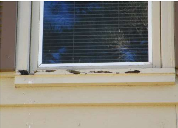
Instance of rot at a sill and trim
