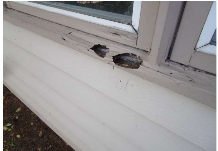
Instance of rot at a sill
