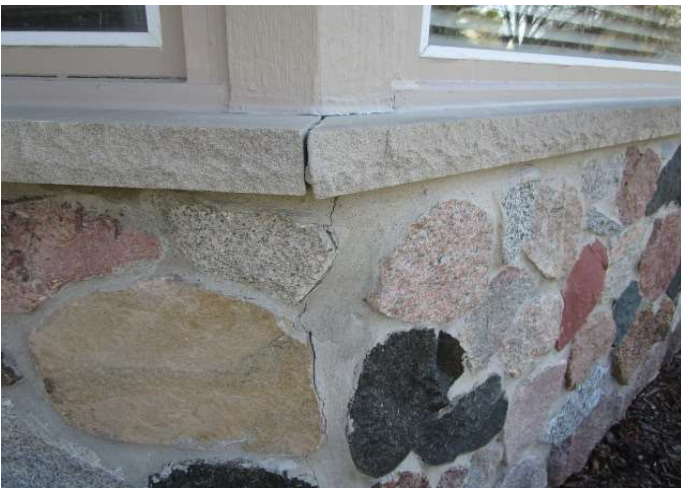
Crack in the mortar
