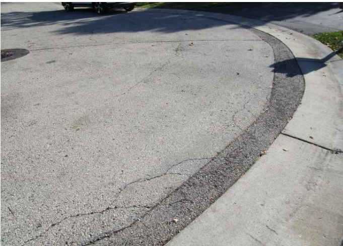
Patch along curb at Pinewood Court
