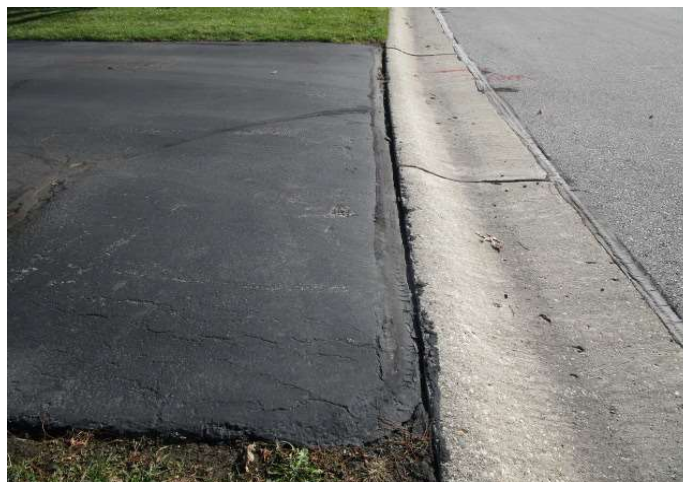
Settlement along a curb and cracks
