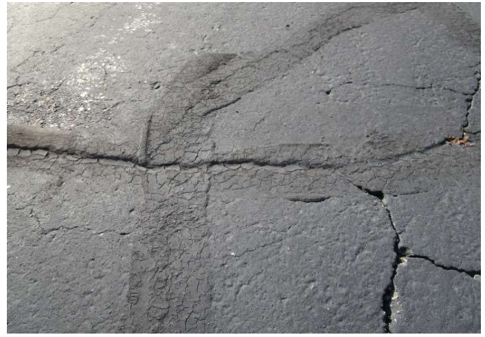
Crack fill at portions of the cracks
