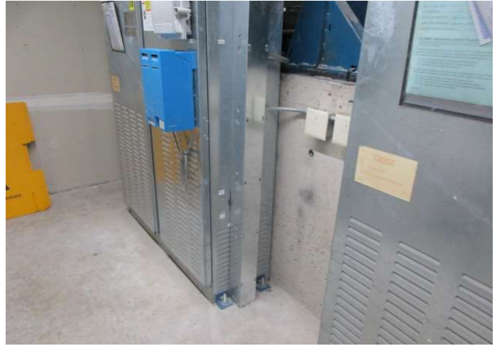
Control at elevator equipment room
