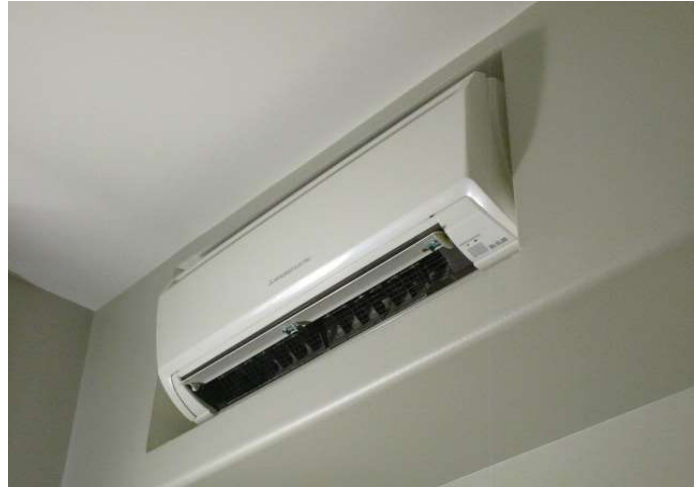
Indoor wall-mounted evaporator / blower unit at hallway
