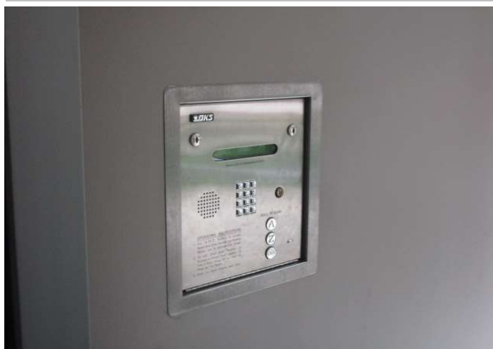
Intercom entry panel at vestibule
