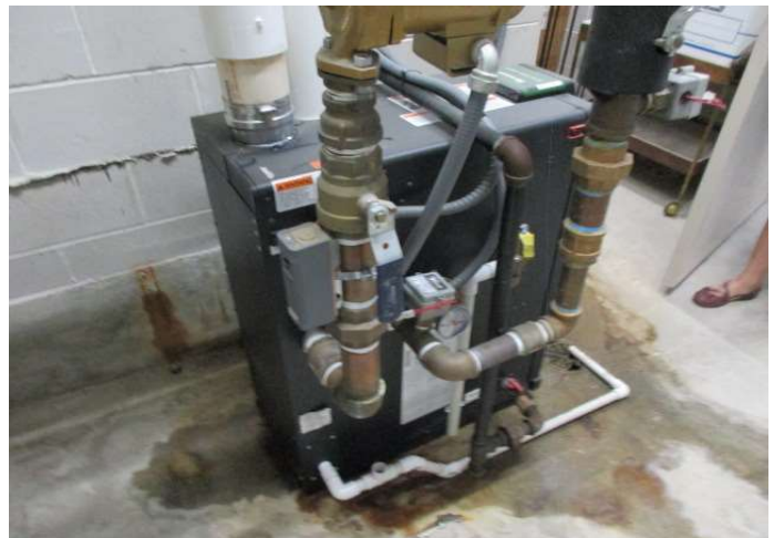
Boiler for domestic hot water
