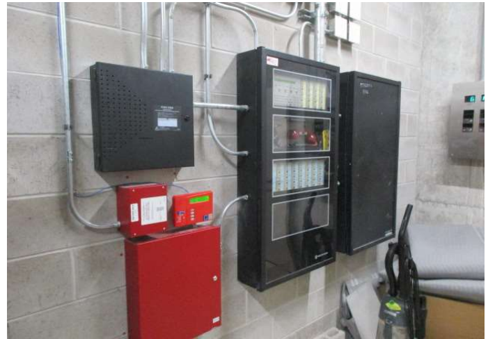
Overview of fire control panel (shared)
