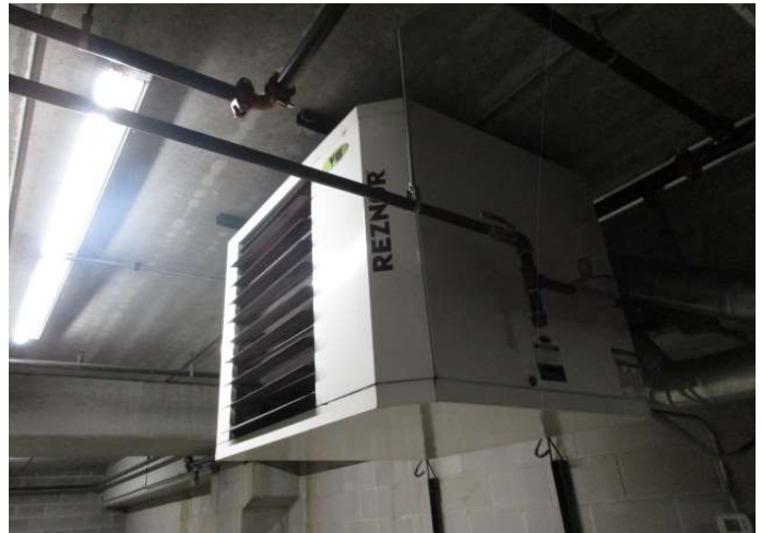
Typical unit heater at garage
