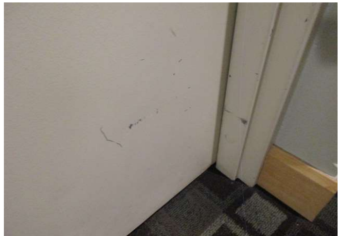
Markings at unit door and door frame
