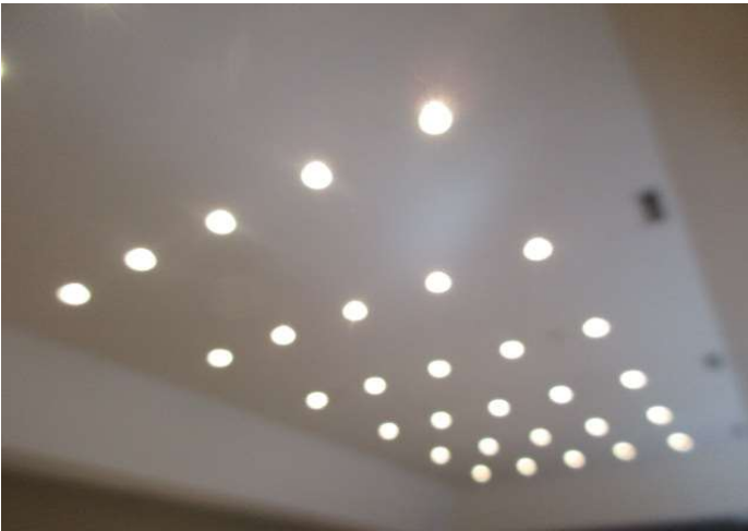
Recessed can lighting at Community Room
