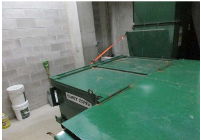
Compactor at trash room
