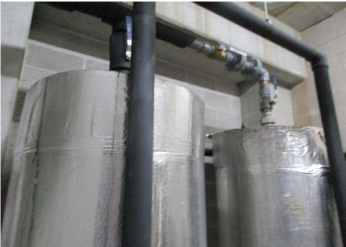
Domestic hot water storage tanks
