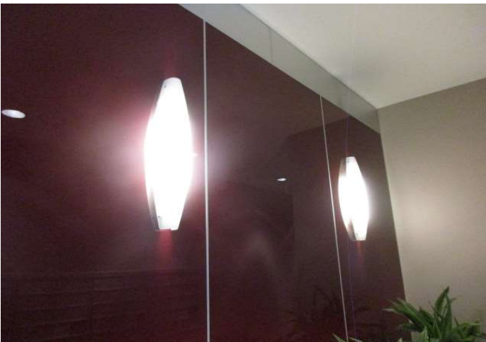
Wall sconces at lobby
