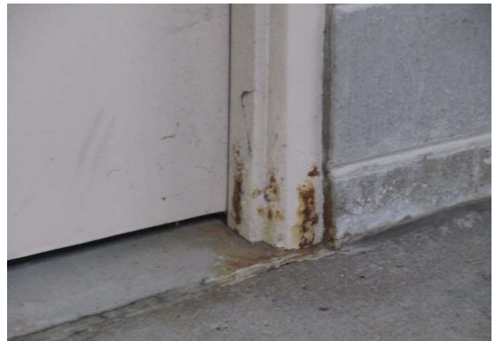
Poor finishes near concrete floor - typical condition
