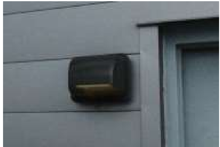
Wall pack fixture at roof
