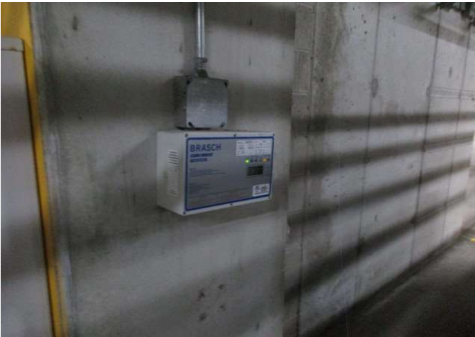
Carbon monoxide detector at parking garage
