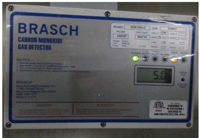
Carbon monoxide detector at parking garage
