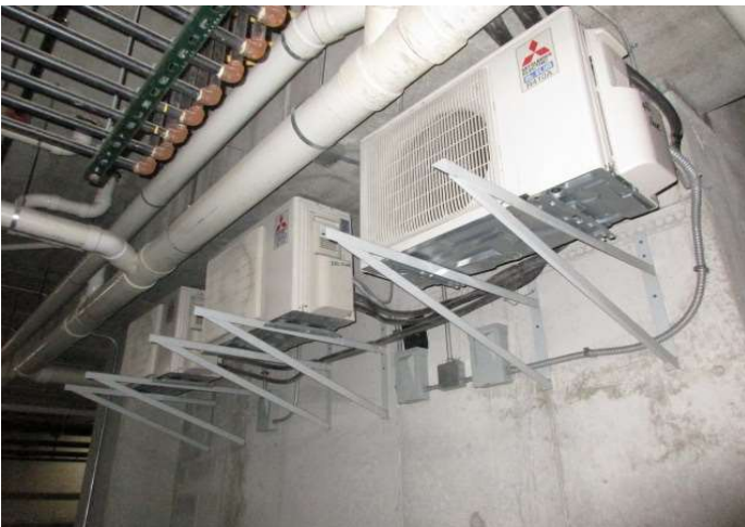
Condensing units at garage
