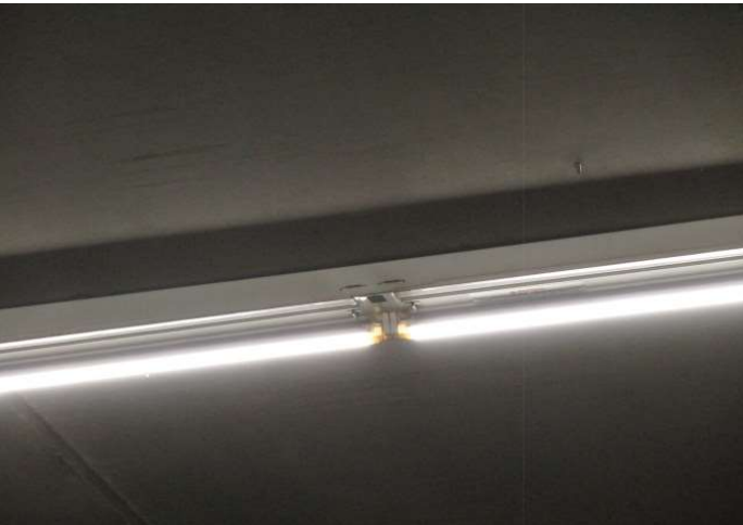
Typical garage light fixture
