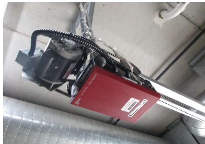
Garage door operator, replaced 2018
