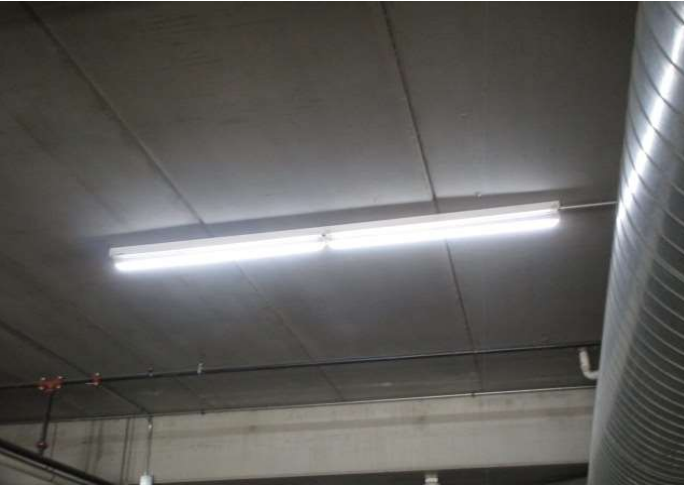
Typical garage light fixture
