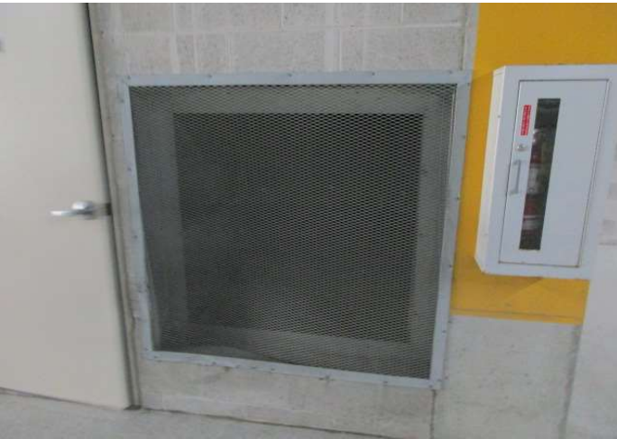
Grille at exhaust fan room
