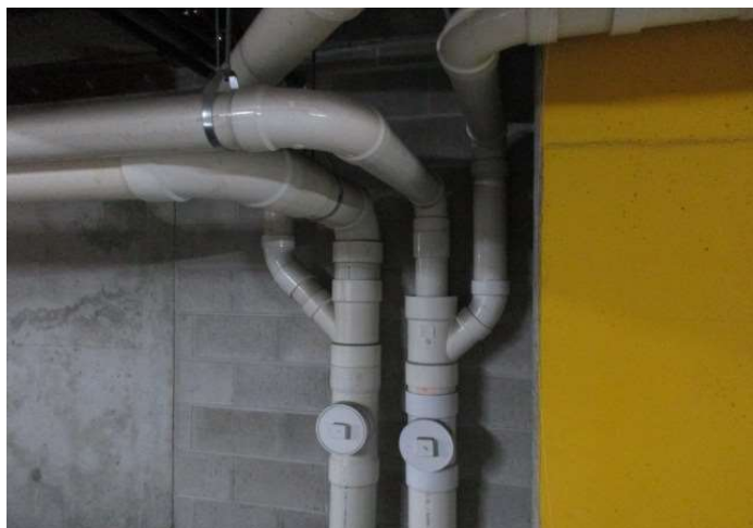
Plumbing waste pipes visible at garage
