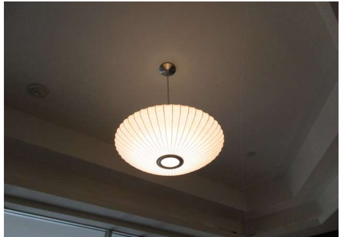
Ceiling fixture at lobby
