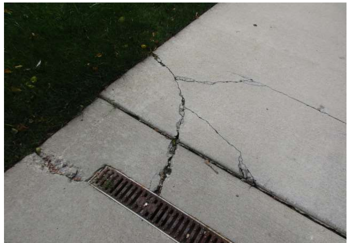
Cracked flatwork at driveway trench drain
