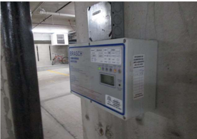
Carbon monoxide detector at parking garage
