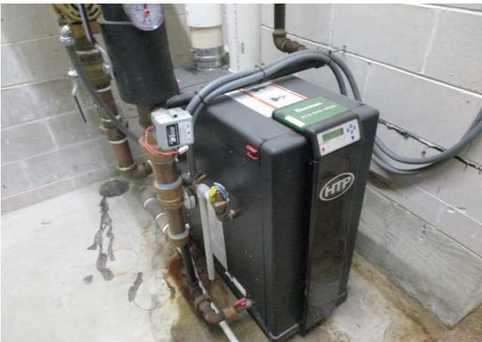
Boiler for domestic hot water
