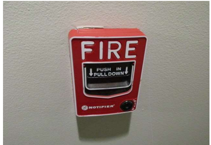
Manual pull station at hallway
