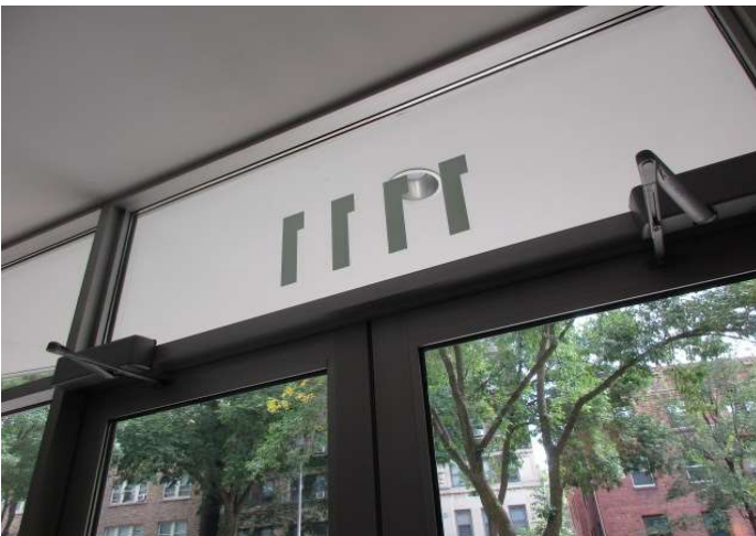
Door closers at entrance doors
