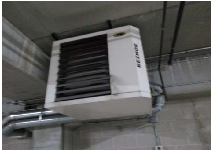
Typical unit heater at garage
