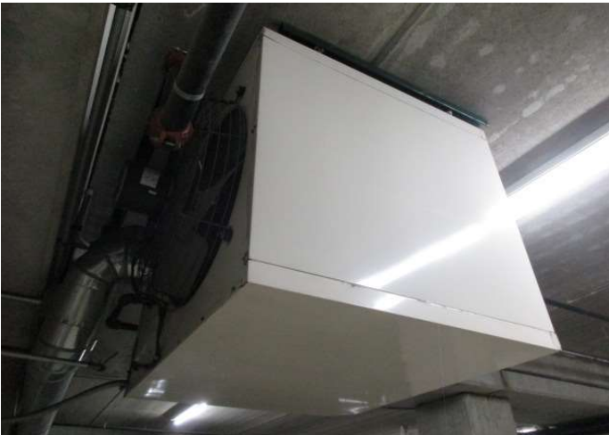
Garage unit heater
