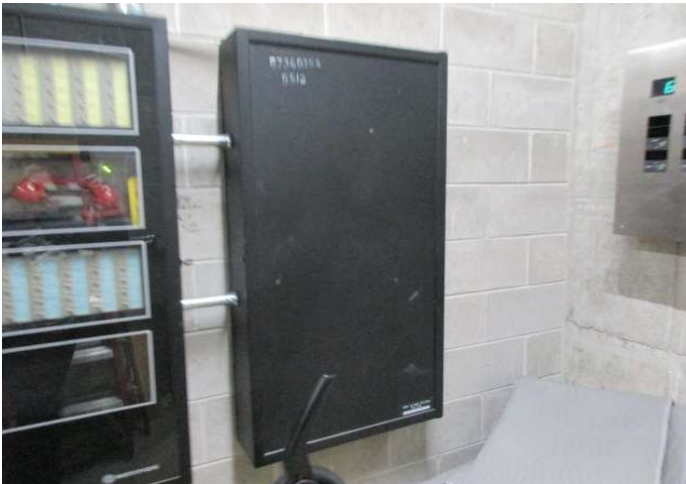
Fire alarm system sub panel (shared)
