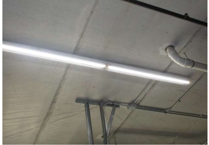
Typical garage light fixture
