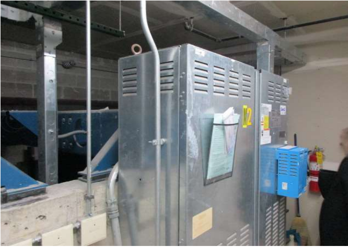
Control at elevator equipment room
