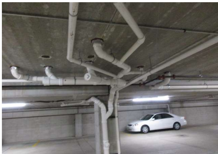
Plumbing waste pipes visible at garage
