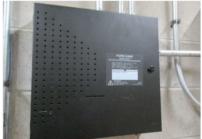
FCPS-24S8 power supply box (shared)
