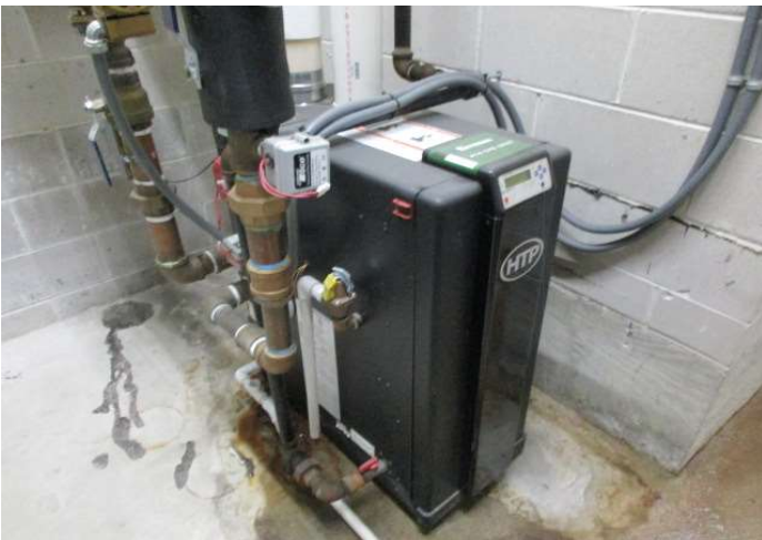
Boiler for domestic hot water
