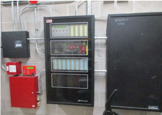
Overview of fire control panel (shared)
