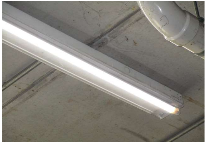
Typical garage light fixture
