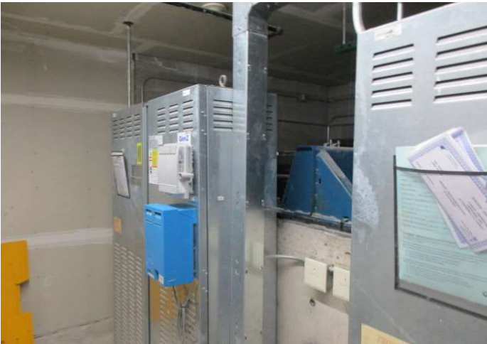
Control at elevator equipment room
