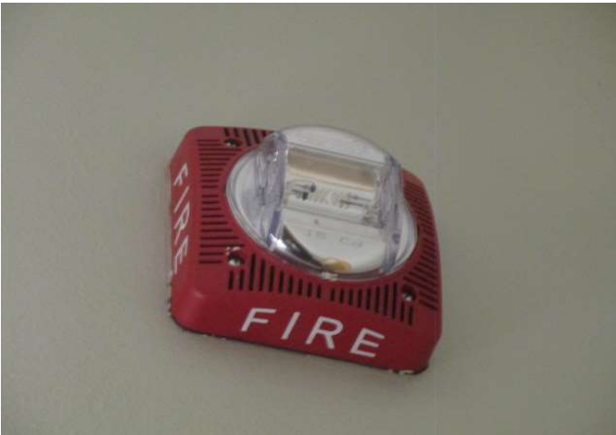
Horn/strobe unit at hallway
