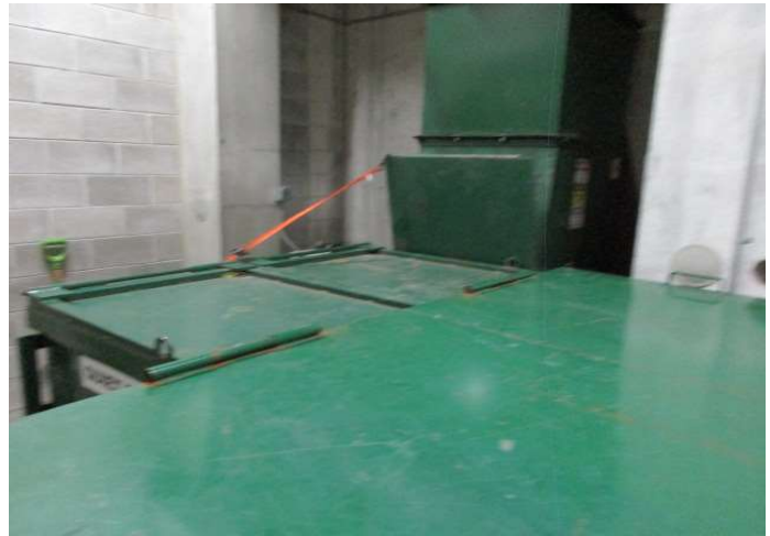
Compactor at trash room
