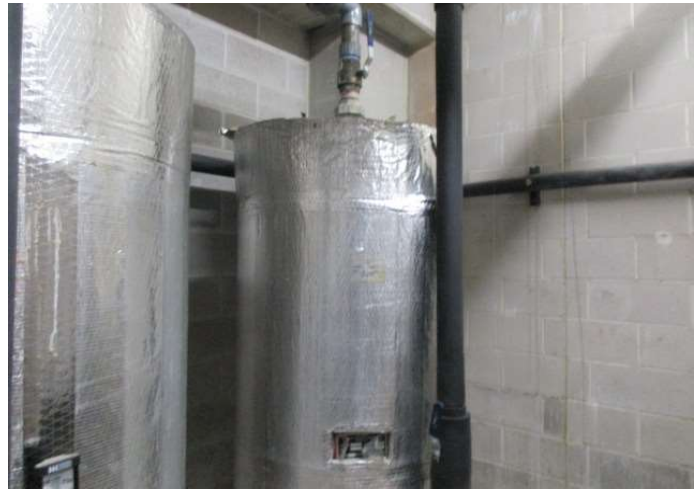
Domestic hot water storage tanks
