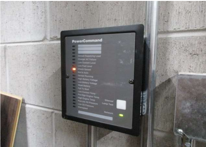
Generator panel at fire command room
