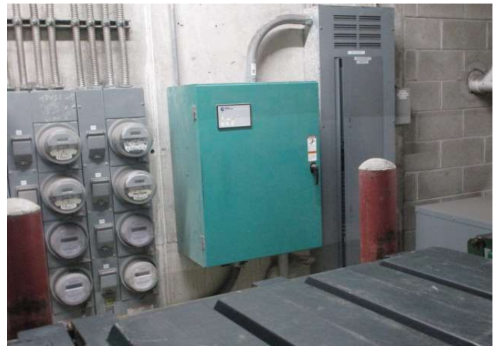
Generator panel at garage
