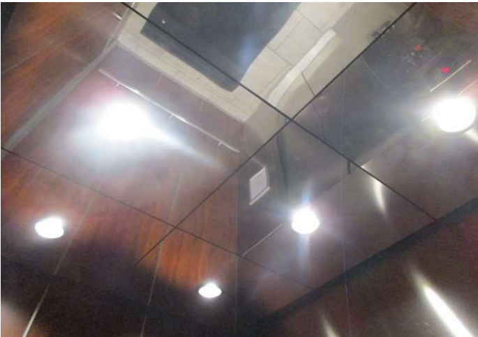
Ceiling grid with lighting
