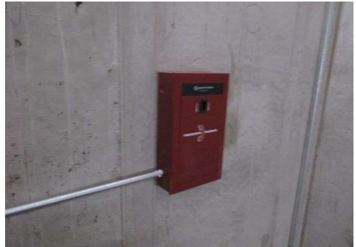
Emergency phone at stairwell
