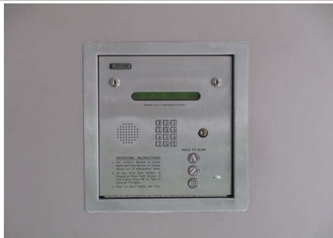
Intercom entry panel at vestibule
