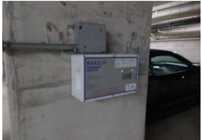
Carbon monoxide detector at parking garage
