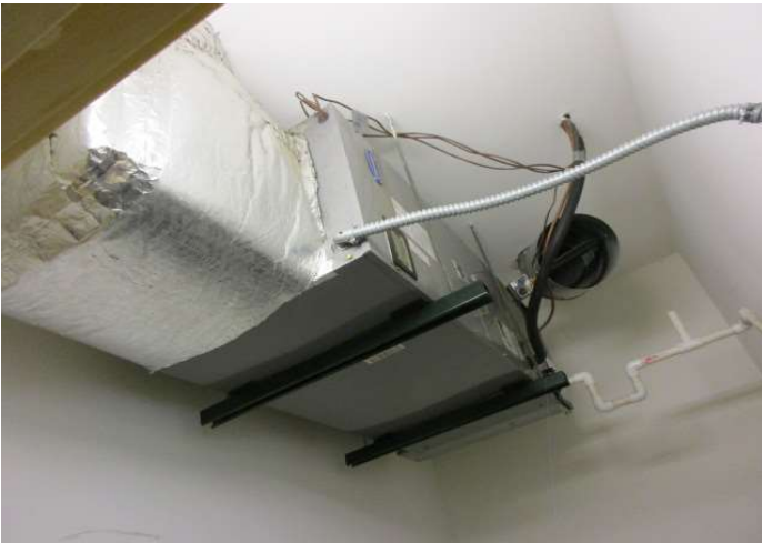
Air handling unit at Community Room
