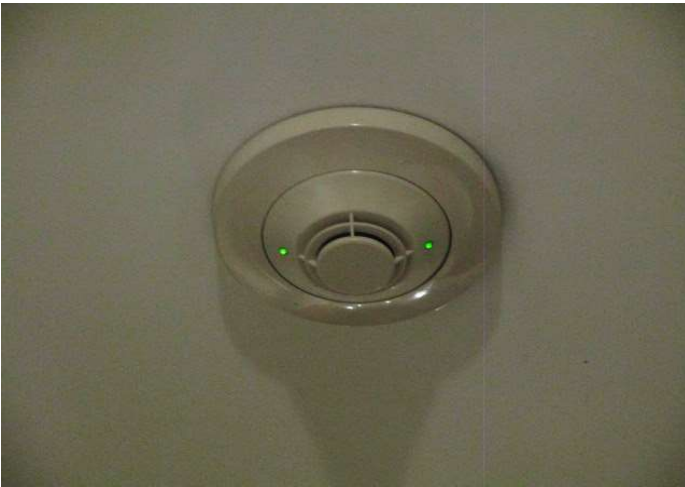
Detector at hallway
