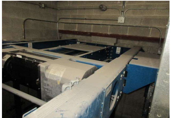
Hoistway equipment at top of shaft
