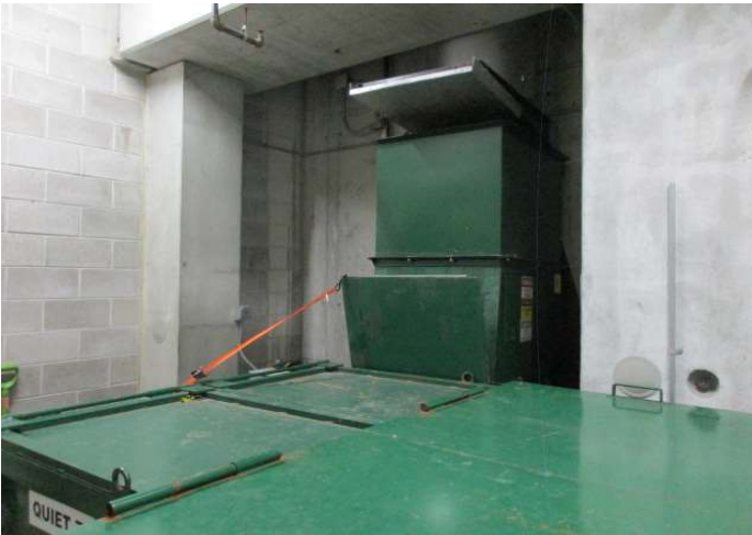
Compactor at trash room
