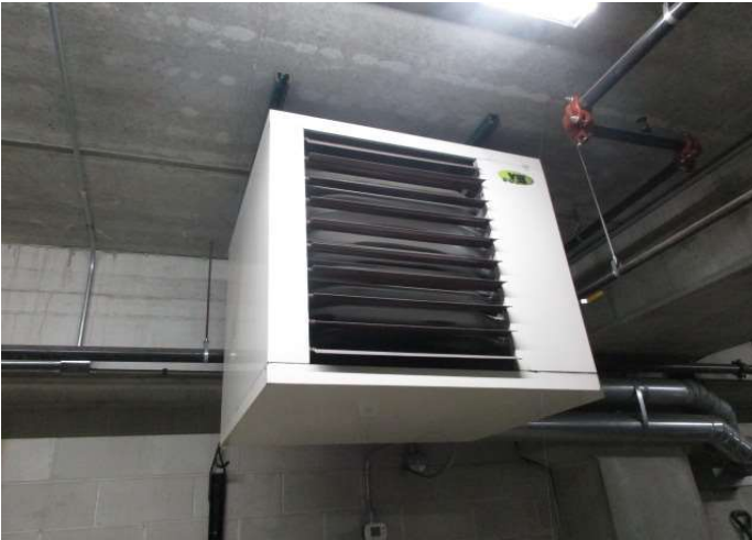
Garage unit heater
