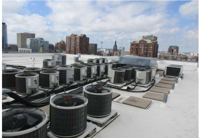
HVAC equipment located centrally at roof
