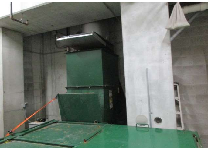
Compactor at trash room
