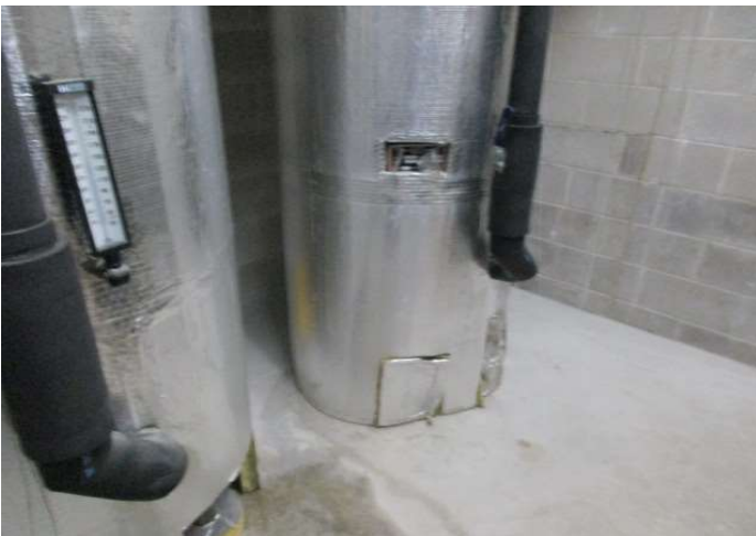
Domestic hot water storage tanks
