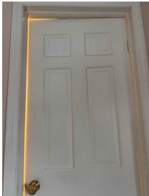
Closet door does not close
