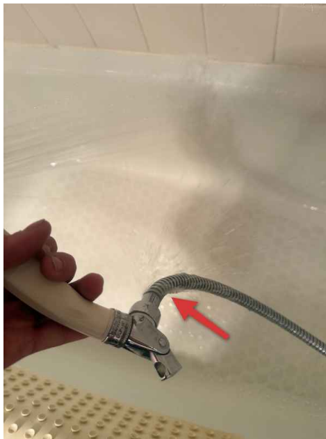
Leaks when in use
