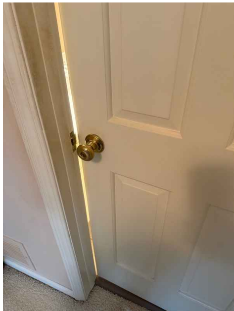
Bathroom door does not latch
