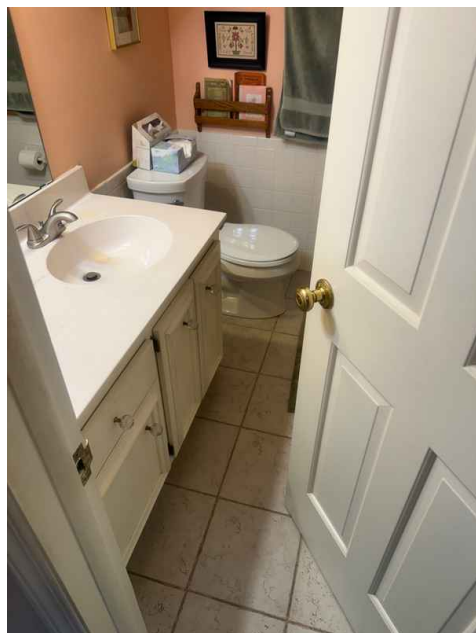
Bathroom door does not latch
