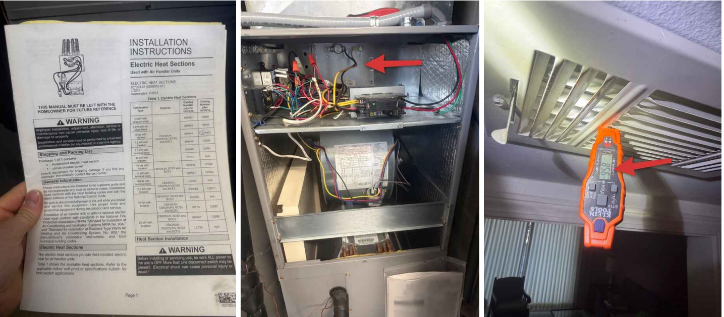
Supply vent temperature
