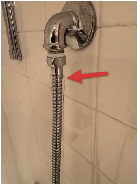
Leaks when in use
