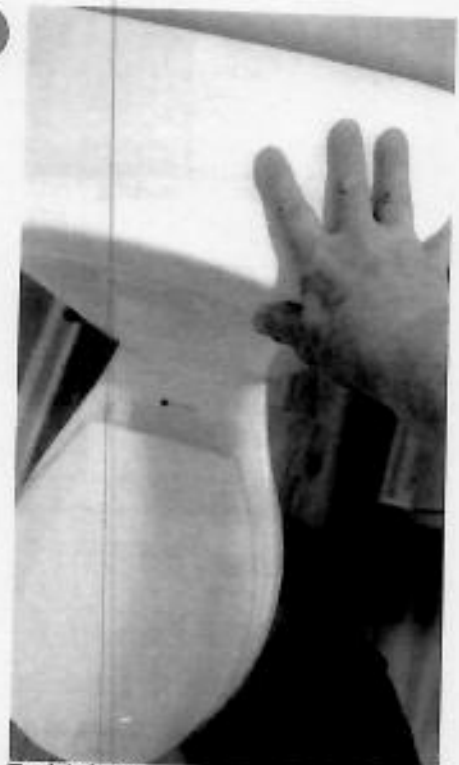
Tank is loose
