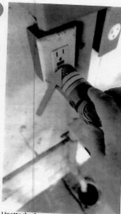
Unattached garage GFCI
