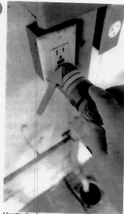
Unattached garage GFCI
