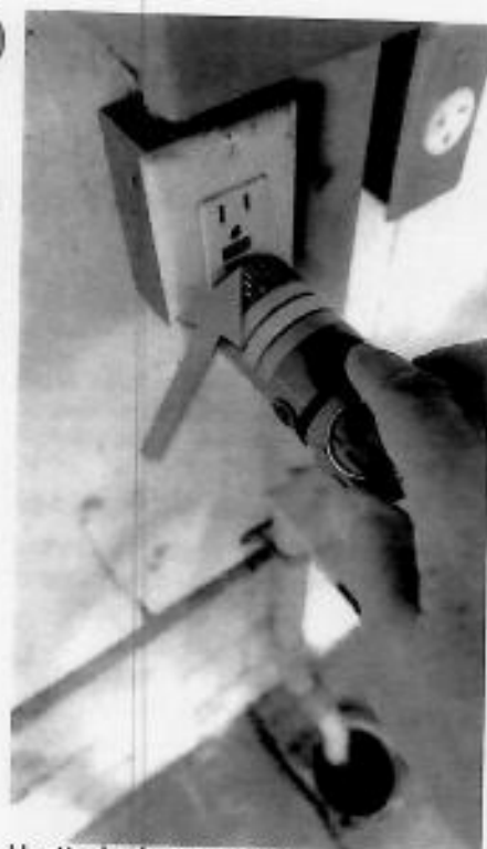
Unattached garage GFCI
