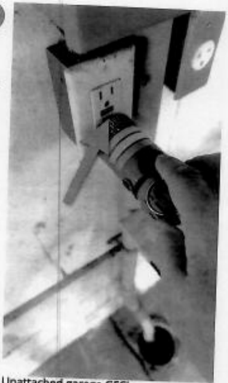
Unattached garage GFCI
