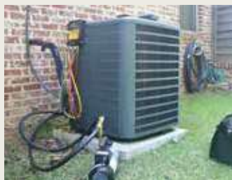
Pre-season HVAC tune ups
