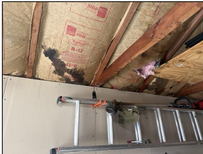
59. Moisture staining. Was dry
