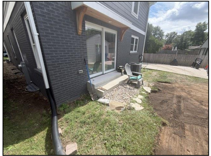
22. Improper slope or drainage
