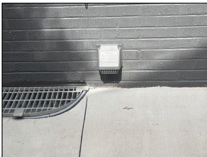
17. Exhaust vent is too close to grade. Monitor
