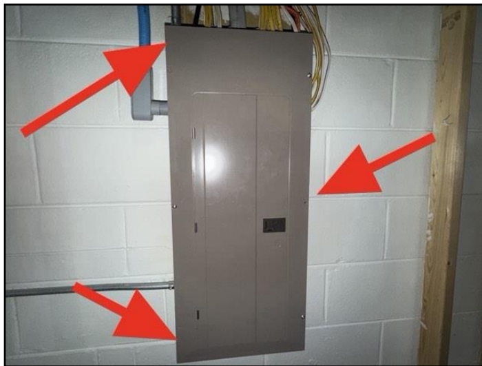
37. Missing screws on electrical box
