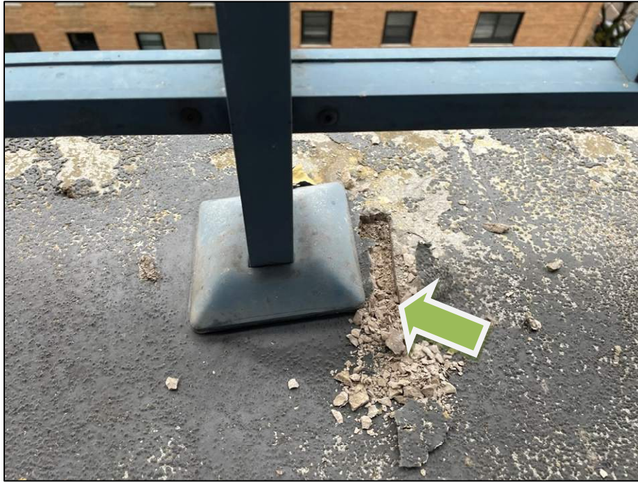
Photo A1-2: Water had penetrated the post anchorage zone and the freeze-thaw cycle crushed the concrete into small chips. Both the concrete and membrane need to be removed and replaced.
