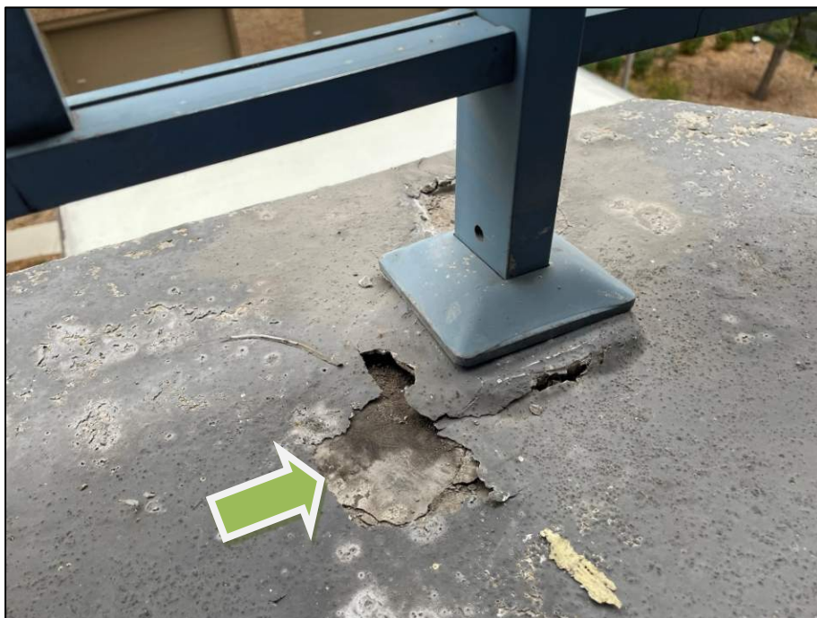
Photo A1-3: In this case only the membrane has failed. Eventually the concrete will fail if the membrane is not replaced.
