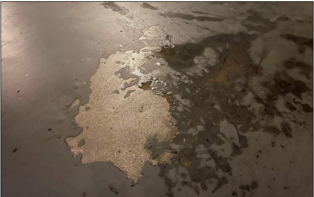
Photo A4-1: A whole section of traffic bearing membrane is missing at a vehicle turning area. A water leak causes a puddle that will freeze in winter and cause a tripping hazard.
