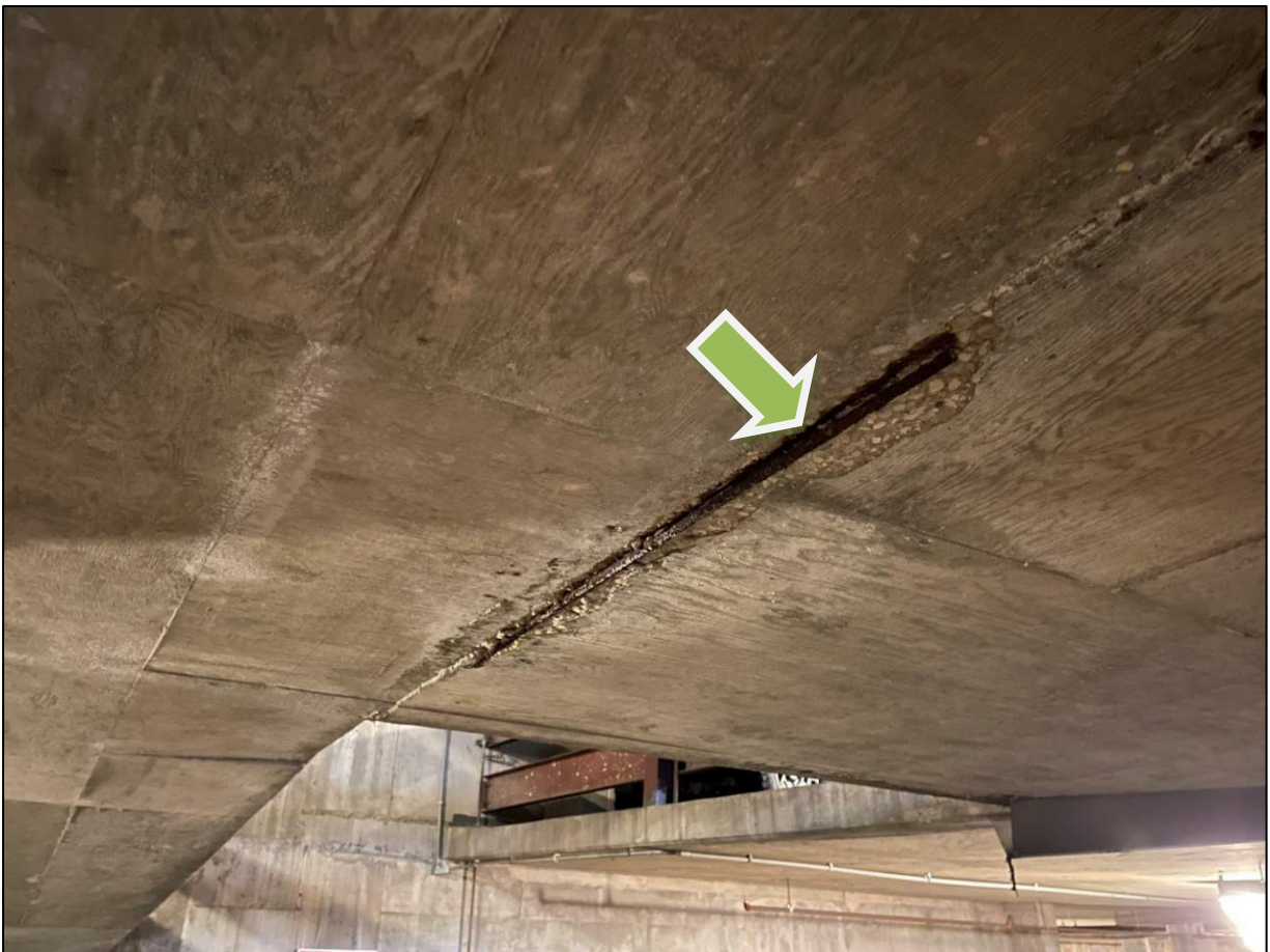
Photo A2-1: A rusted rebar is exposed within a concrete spall.
