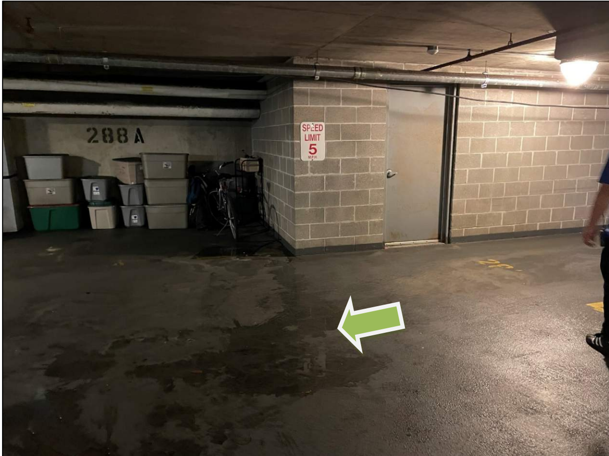
Photo A4-2: The failed traffic membrane and puddle is located between designated parking spaces 288A and 288.
