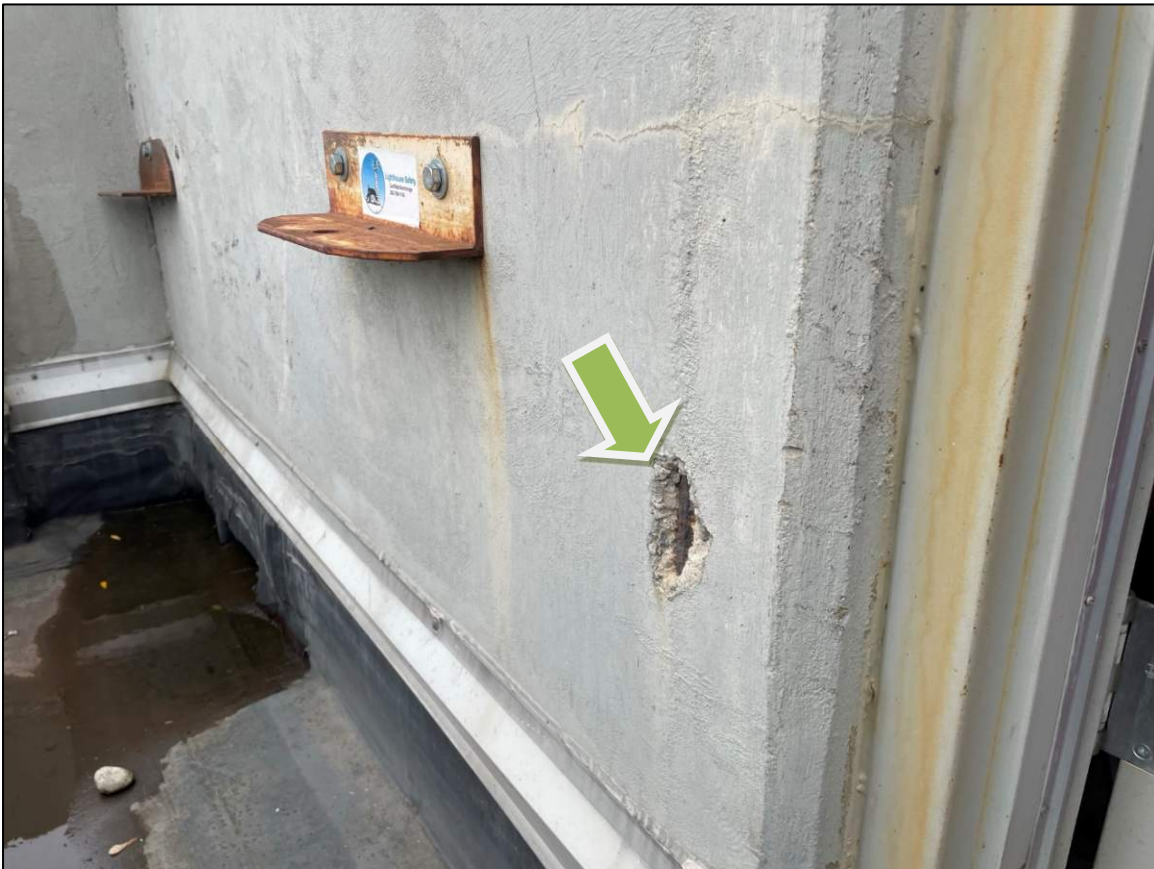
Photo C3-1: A concrete spall on the south wall of the mechanical penthouse has an exposed rebar.
