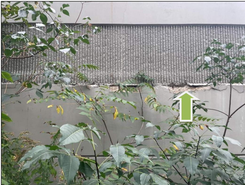
Photo B2-1: Large concrete spalls are at the cold joint between the parking wall and the parapet wall above.
