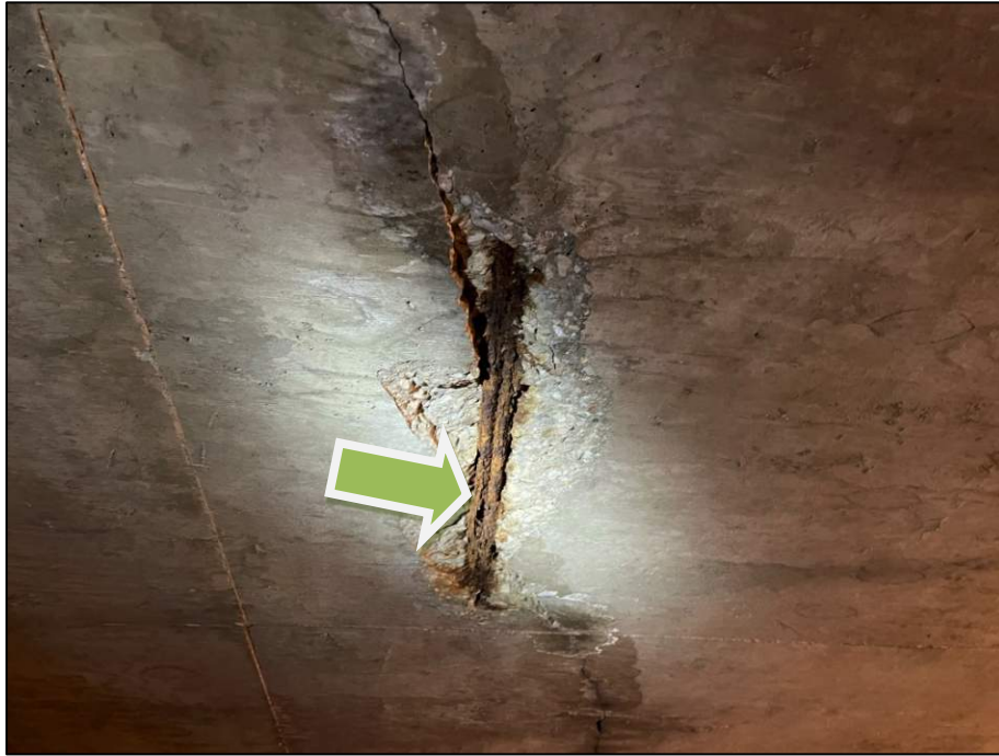
Photo A2-2: The rebars shown within the spall are very low in the slab profile, which lead to their premature rusting.
