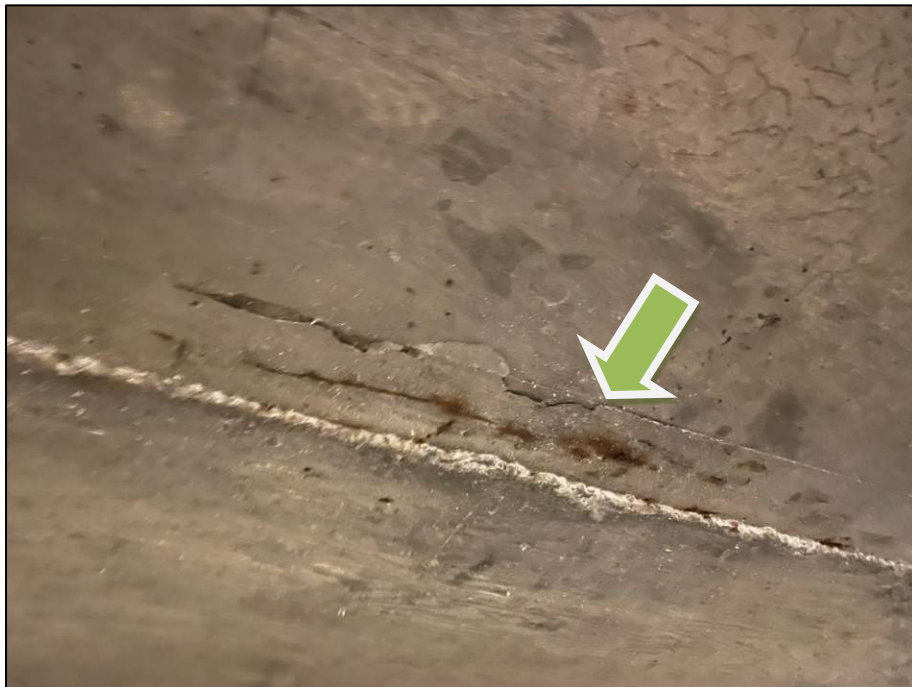
Photo A2-3: This is an imminent spall. Loose concrete should be tapped with a hammer, and removed so it does not fall on a person or vehicle.
