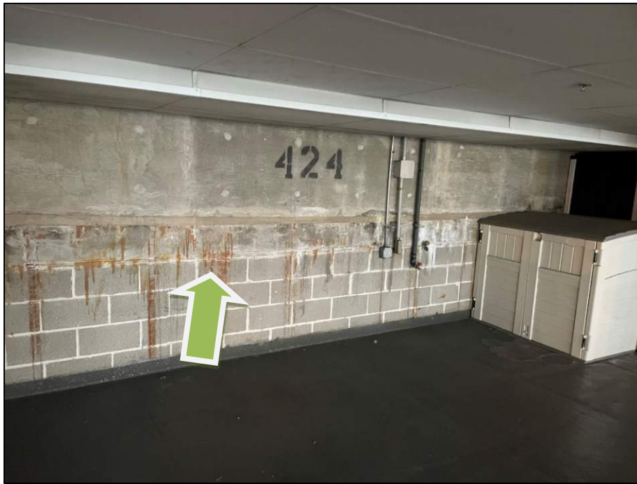
Photo A3-2: Efflorescence and rust staining coming from top and bottom of pool slab down the block wall.
