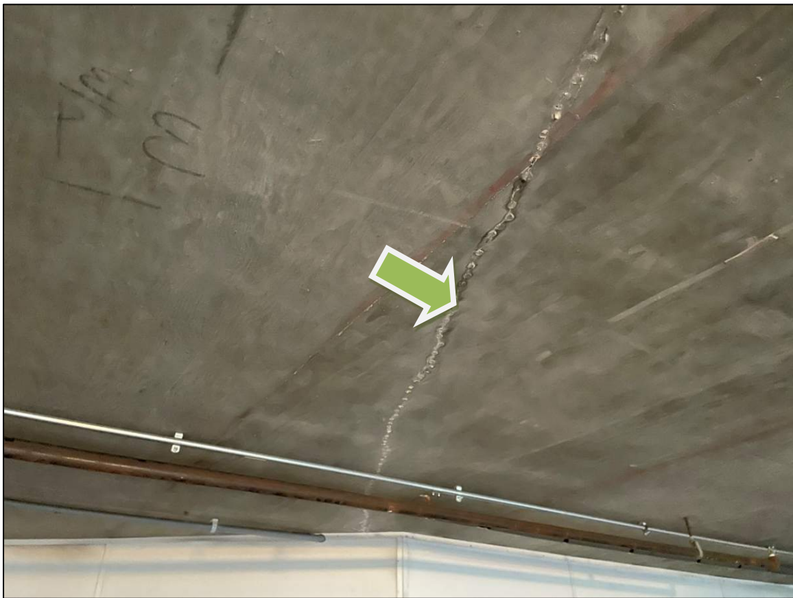
Photo C4-1: A crack on the bottom of the floor slab (ceiling) had been injected with epoxy and still has some of the damming material (to keep epoxy from spilling out) left in place.
