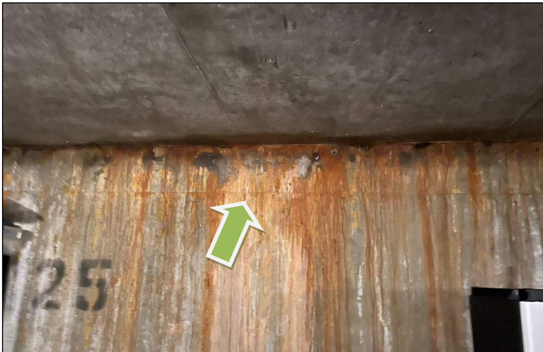
Photo C1-1: Rust has stained the rubber adhesive on the side of the wall. The cold joint between the wall and the floor slab or previously repaired cracks could have stained the adhesive the rust color long ago.
