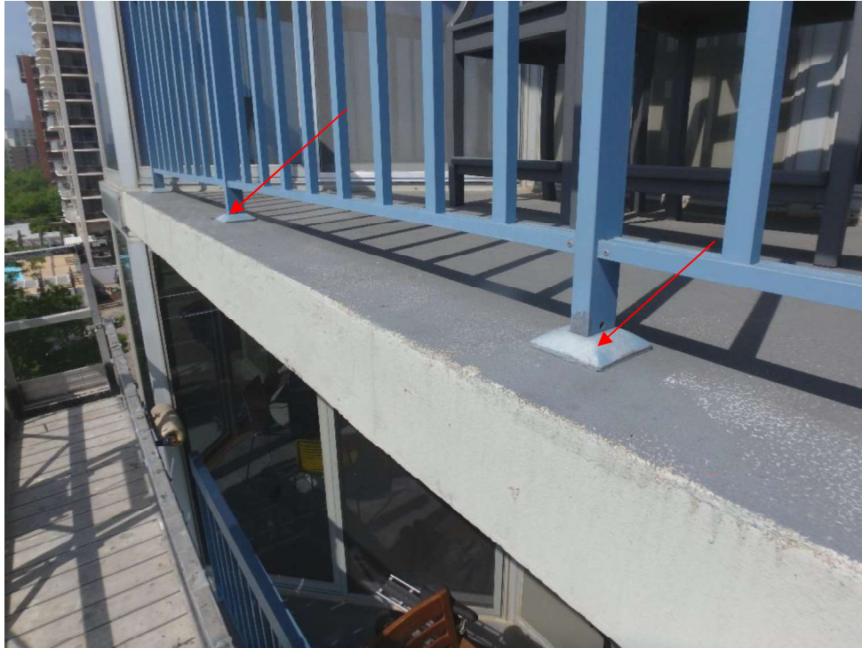
8- Spalled concrete at balcony rail footing- repairs completed by others in 2022.
