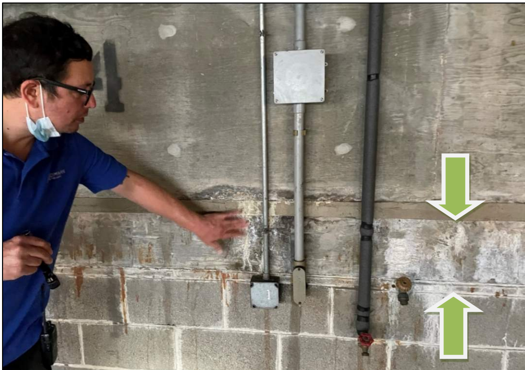
Photo A3-1: Mineral deposits (efflorescence) and rust stains streak down sides of pool slab joint.
