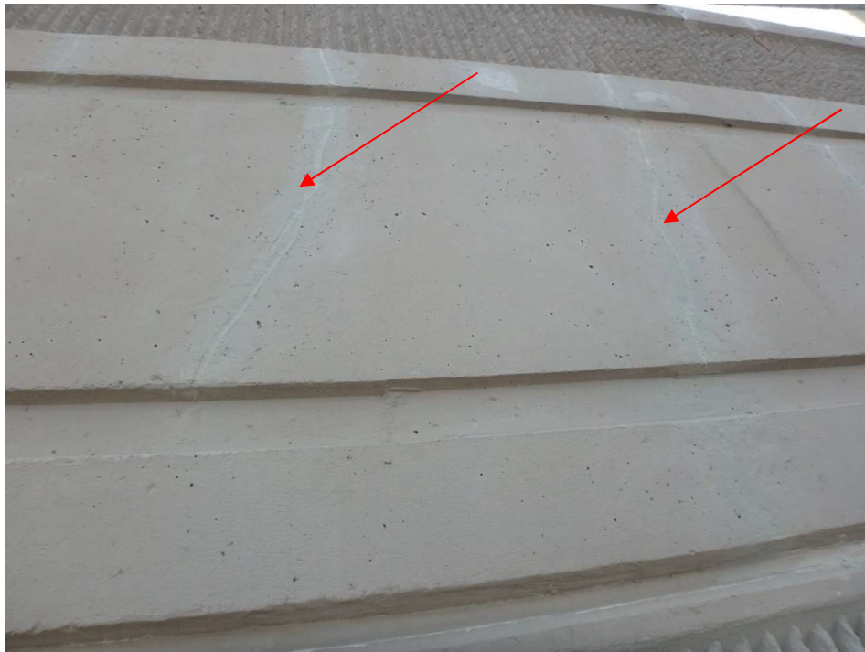
2- De-bonded sealant and hairline crack in concrete repairs - cracks were routed, and sealant replaced with a new sealant
