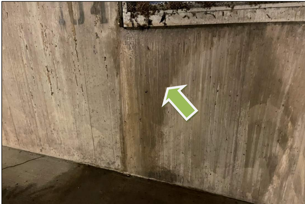
Photo B3-2: Water overflows inside the area well and leaks down the side of the wall. Debris inside the areas to be removed so the saturation problem can properly be identified.
