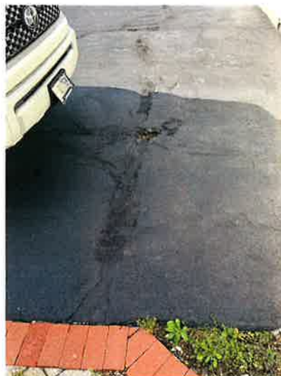
Surface damage at the drive
