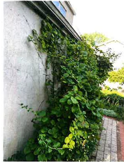
Recommend trimming and/or removal of vegetation away from home
