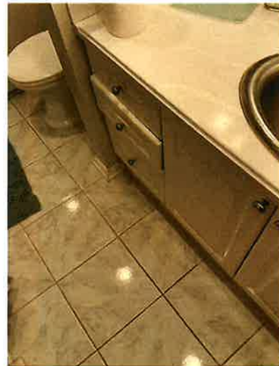
Repair the vanity cabinet drawer two close properly
