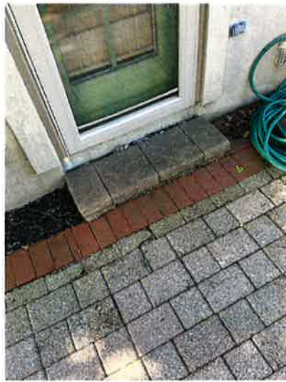
Uneven risers at the entry step
