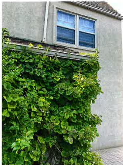
Recommend trimming and/or removal of vegetation away from home
