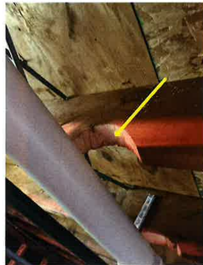
Cut joist looks recent.
