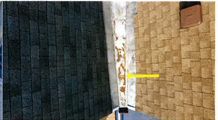
Corroded galvanized pan valley
