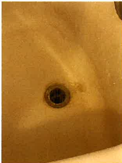
Missing tub stopper
