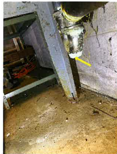
Corrosion noted. No moisture observed
