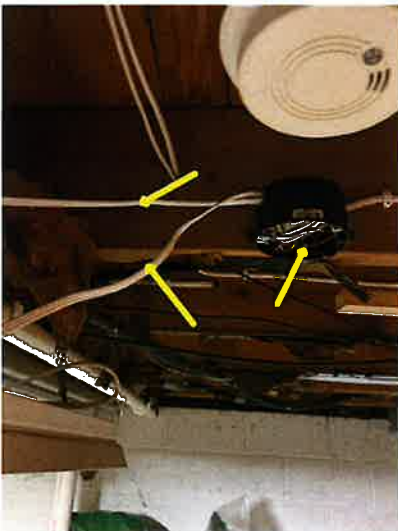
Handyman wiring of basement lighting into an open junction box. Have an electrician evaluate and repair
