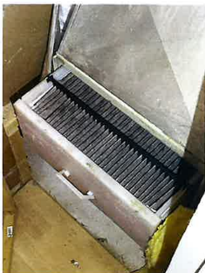
Dirty furnace filter needs to be changed.
