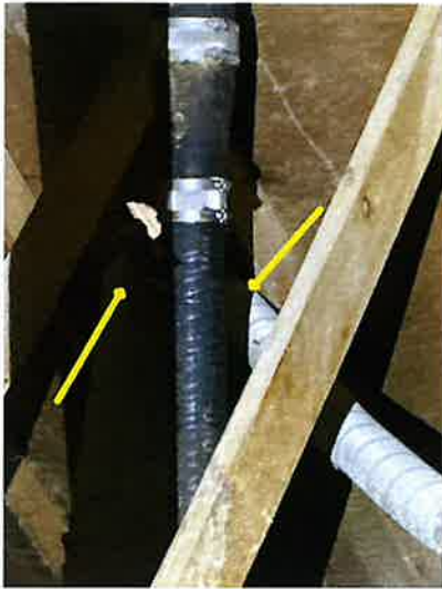
Fans don't vent sealed through the roof opening
