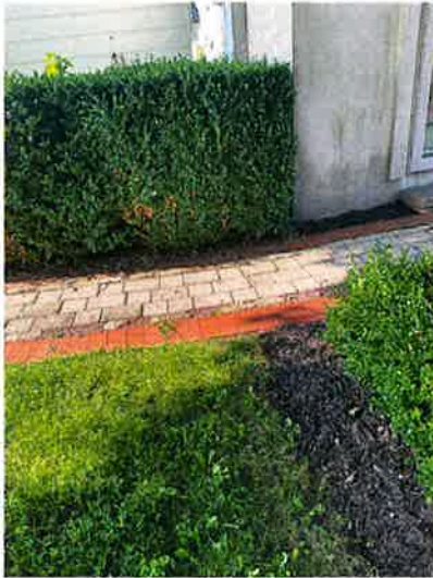
Some brick deterioration and sloping toward the home at the sidewalk. Make repairs as needed
