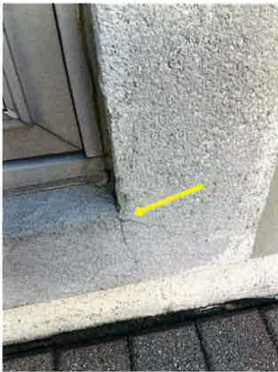
Cracks at trim
