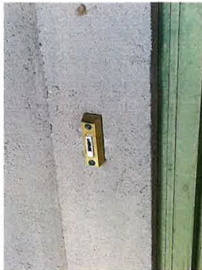
Missing door bell
