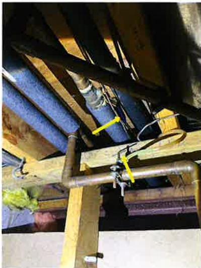
Main water shutoff
