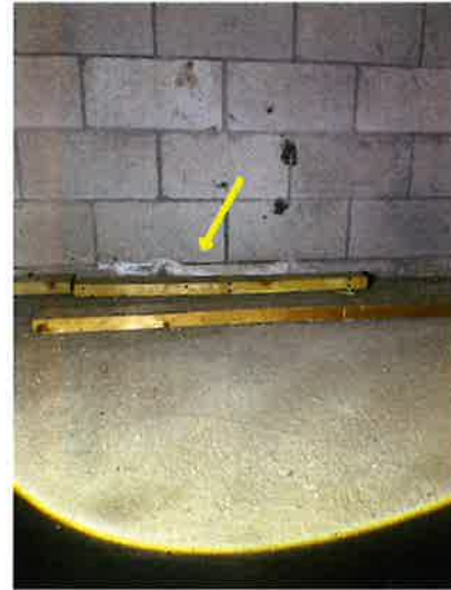
Low moisture stains
