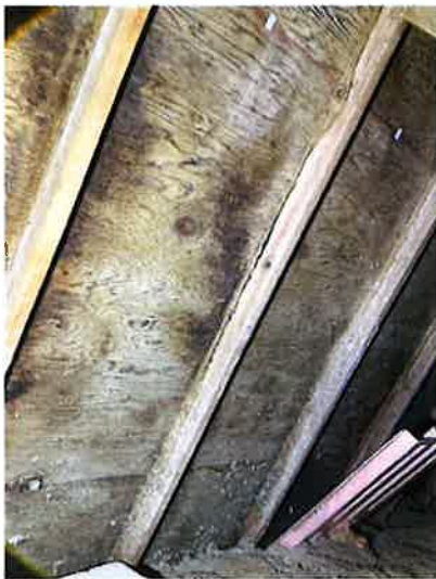
Microbial growth/condensation stains
