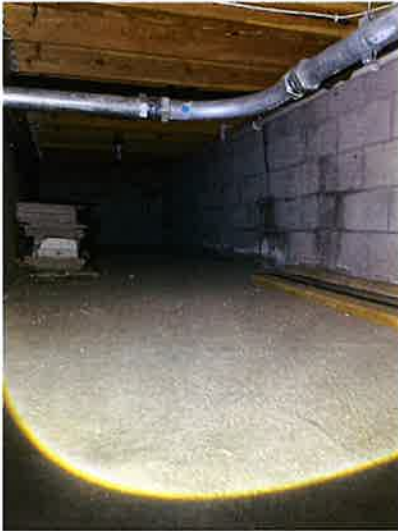
High moisture stains.
