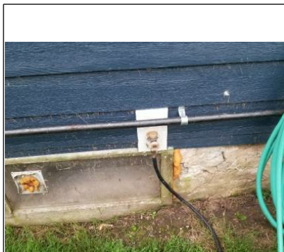
North hose bib operational
