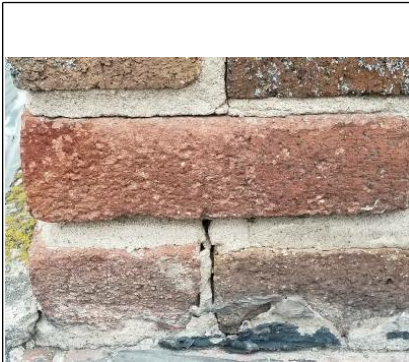
Tuckpointing maintenance recommended
