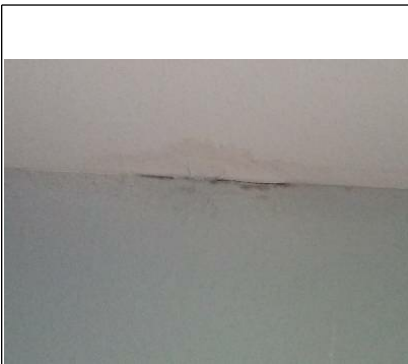
Moisture stains in entryway.
