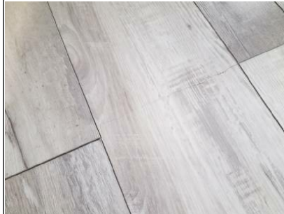
Floor is cracked
