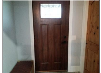
Unable to open door. Deadbolt malfunctioning. Safety Hazard
