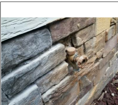
East hose bib not operating at time of inspection
