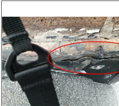
Flashings. Loose, recommend qualified contractor evaluate and repair
