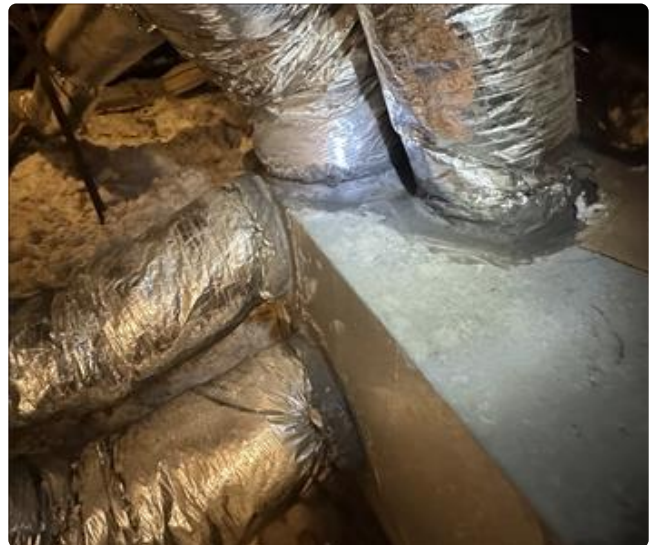
Clean HVAC exhausts
