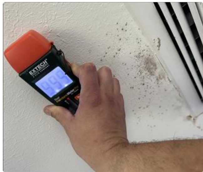
Elevated moisture, visual microbial growth, water damage
