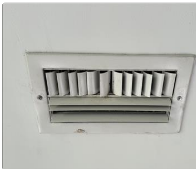
HVAC vent overview
