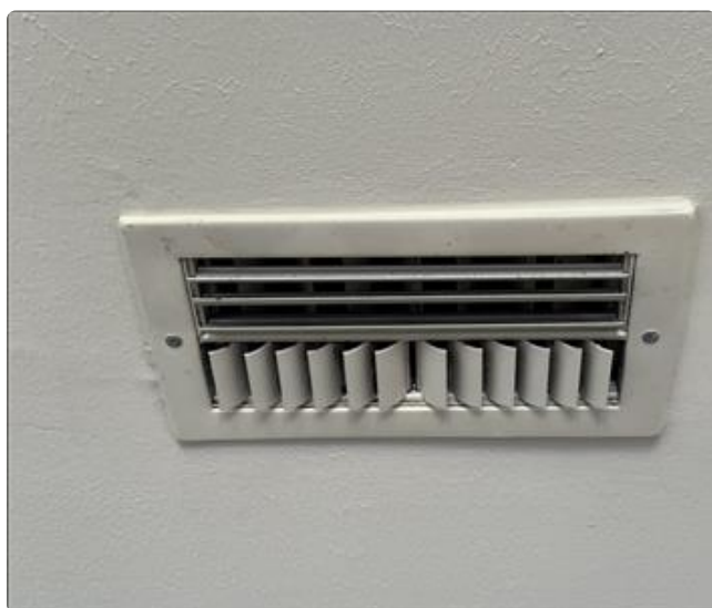
HVAC vent overview
