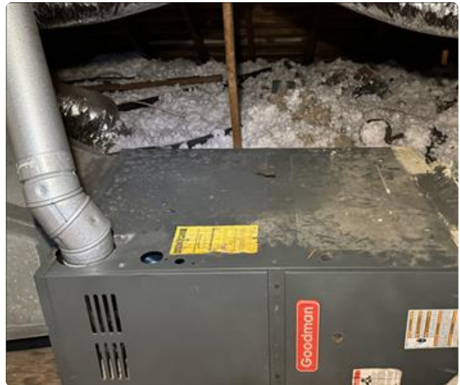
Dust/microbial growth on HVAC
