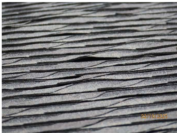
Lifted shingles at the west end center of the north sloping roof covering
