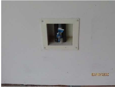
Shut off valve in the north wall of the garage
