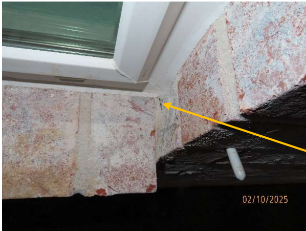
Gap in the mortar at the right side of the north side right window ledge
