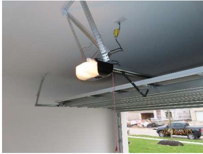
General view of the garage door opener
