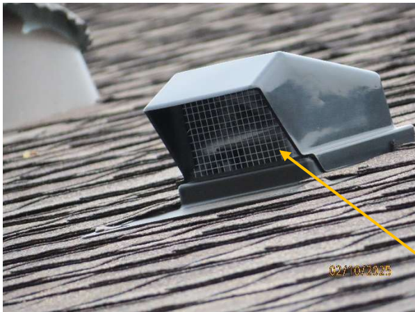
The dryer vent termination cover through the north sloping roof has a screen
