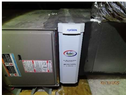
General view of the media filter
