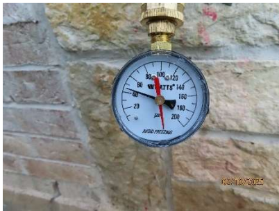
Water pressure approximately 45 psi
