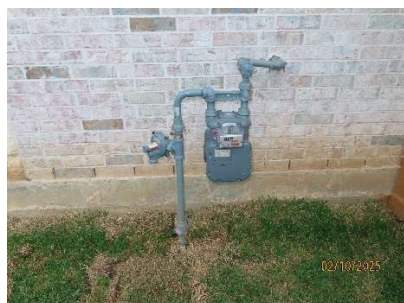
General view of the gas service entrance / meter
