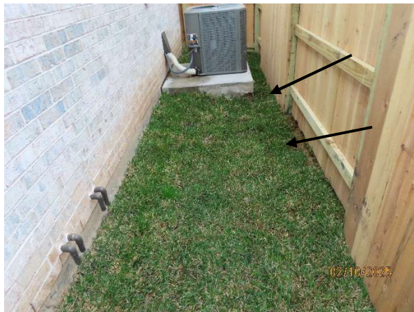
Water collecting the north side swale around the a/c condenser pad
