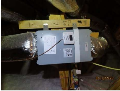
General view of the ventilation controller
