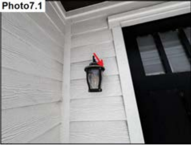
Penetration Sealants / Seal
