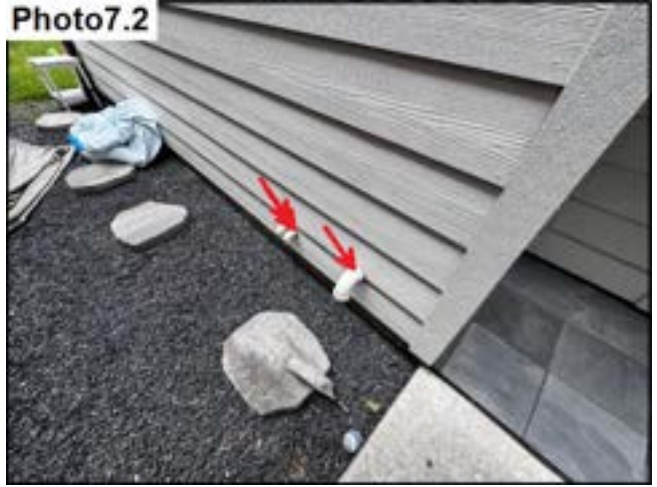
Penetration Sealants / Seal
