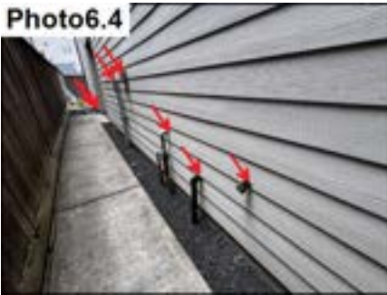
Penetration Sealants / Seal
