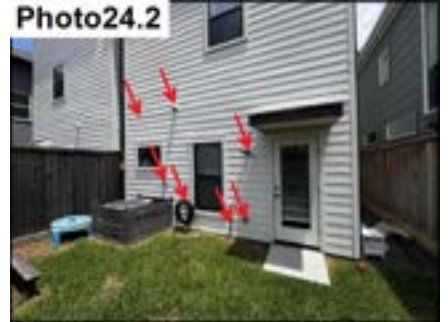
Penetration Sealants / Seal
