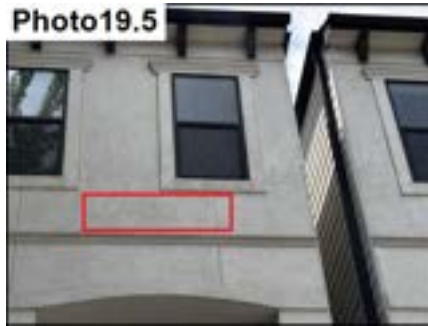
Hairline Cracks / Paint (Aesthetic)
