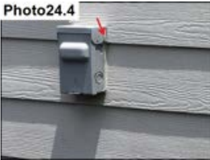
Penetration Sealants / Seal
