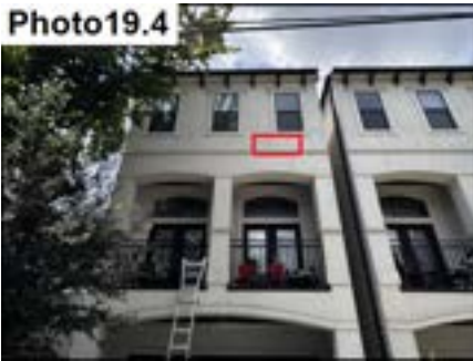
Hairline Cracks / Paint (Aesthetic)
