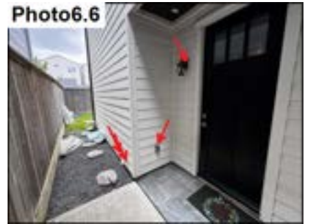
Penetration Sealants / Seal
