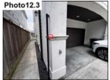
Impact Damage / Repair
