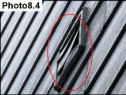
Broken Vent / Replace and Seal
