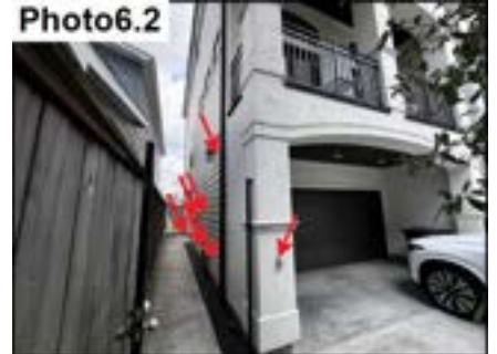
Penetration Sealants / Seal
