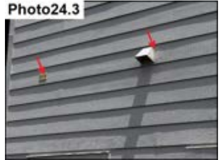
Penetration Sealants / Seal
