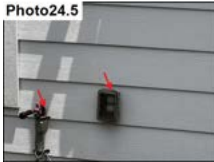
Penetration Sealants / Seal
