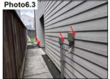
Penetration Sealants / Seal
