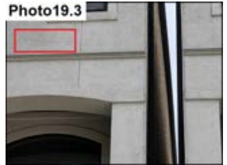
Hairline Cracks / Paint (Aesthetic)
