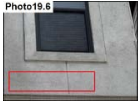
Hairline Cracks / Paint (Aesthetic)
