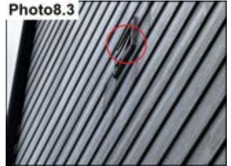
Broken Vent / Replace and Seal
