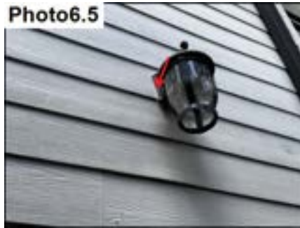
Penetration Sealants / Seal
