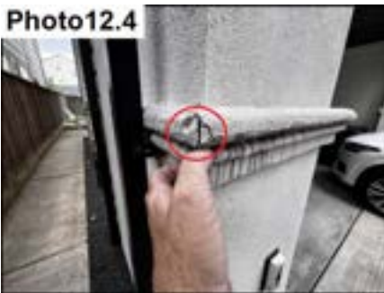
Impact Damage / Repair
