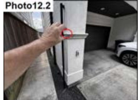
Impact Damage / Repair
