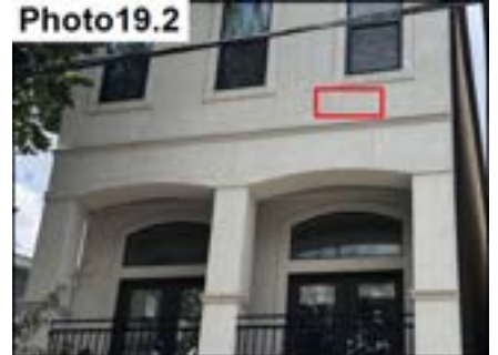
Hairline Cracks / Paint (Aesthetic)
