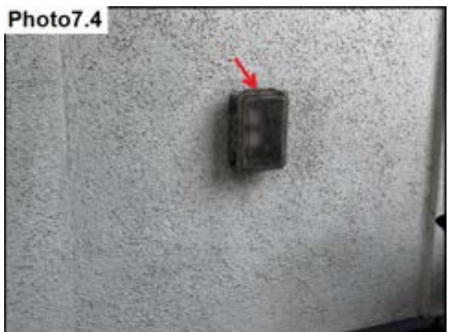
Penetration Sealants / Seal
