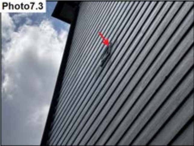
Penetration Sealants / Seal
