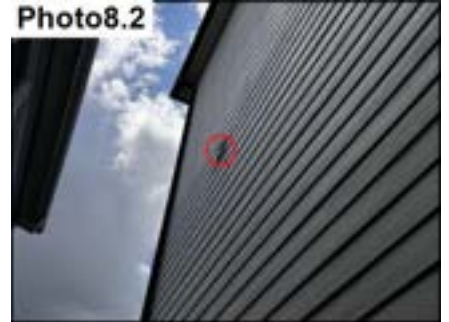
Broken Vent / Replace and Seal
