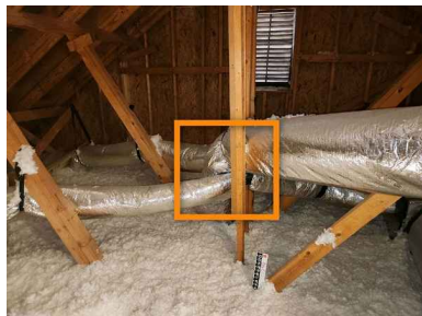
For Example:Ducts In Contact in the Attic
