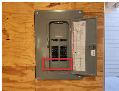
Garage Electrical Panel
