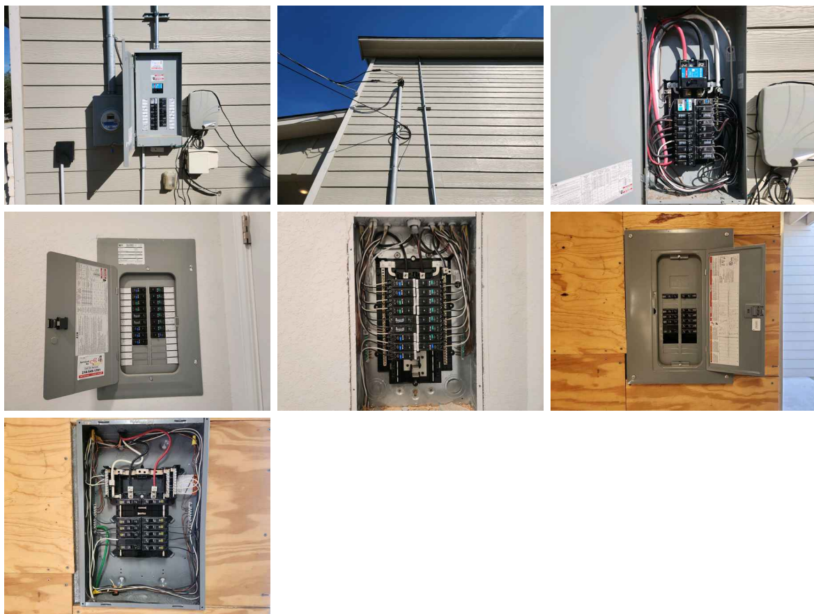
General Infrared Photos of Distribution Panels:
