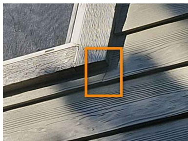
For Example:Damaged Siding Rear
