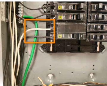
Garage Electrical Panel
