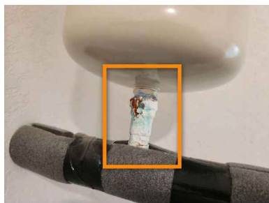
Corroded Fittings at Water Heater Expansion Tank
