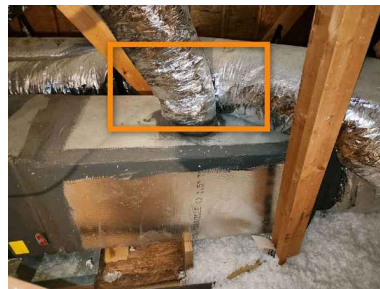
For Example:Ducts in Contact in the Attic
