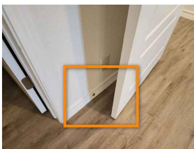
Missing Door Stopper Primary Bedroom
