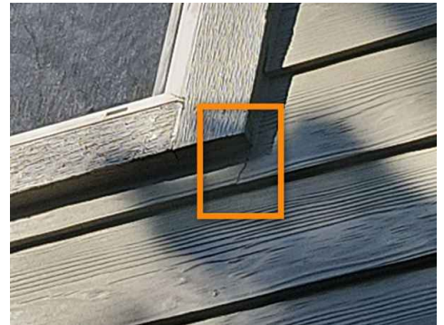
For Example: Damaged Siding Rear
