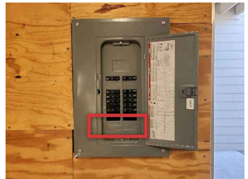
Garage Electrical Panel
