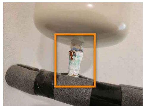
Corroded Fittings at Water Heater Expansion Tank
