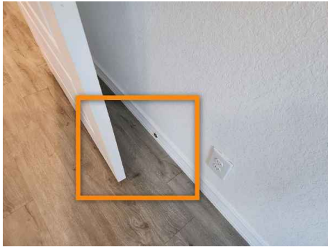
Missing Door Stoppers 2nd Floor Bedrooms
