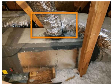
For Example:Ducts in Contact in the Attic
