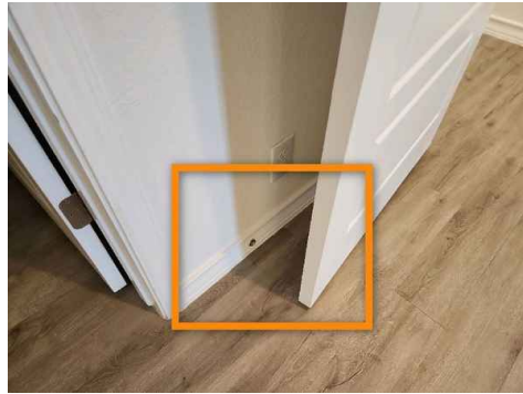
Missing Door Stopper Primary Bedroom
