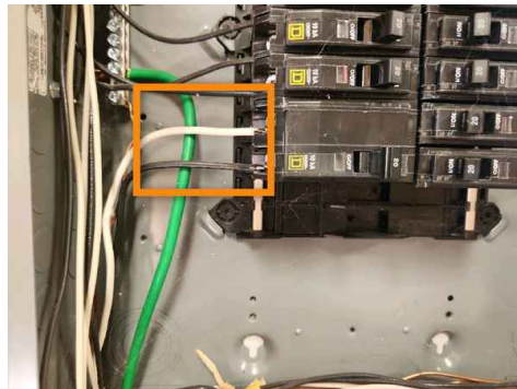
Garage Electrical Panel
