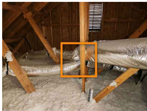
For Example:Ducts In Contact in the Attic
