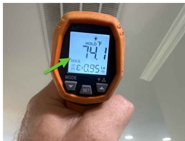
Return air temperature
