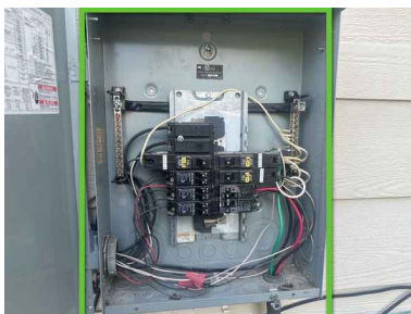
Sub panel with dead front removed
