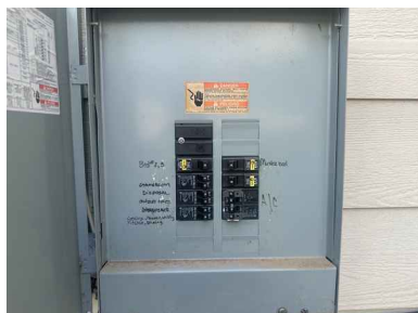
Rear: Eaton Sub Panel
