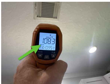
1st Floor Hot air temperature
