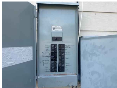
Rear: Cutler Hammer Service Panel
