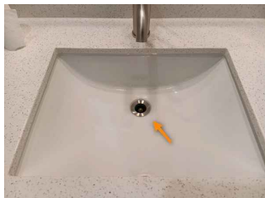
Missing stopper, half bathroom
