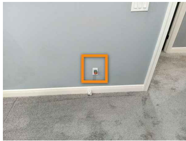
Hot / neutral reversed, second floor left bedroom
