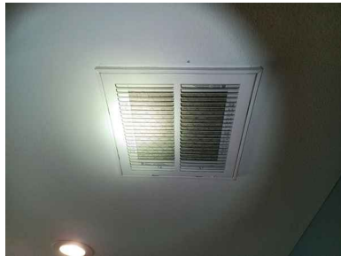
Dirty, primary bedroom
