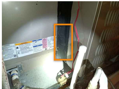
Air leakage, coil cabinet
