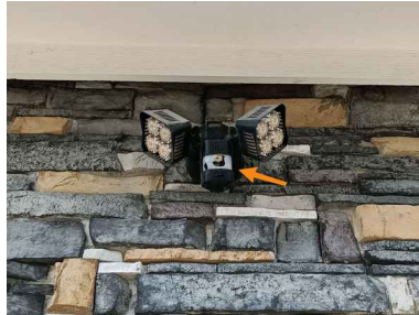
Damaged sensor, front
