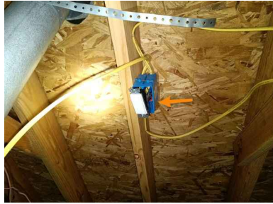
Loose, furnace switch
