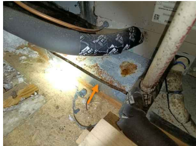
Corrosion, dry at time
