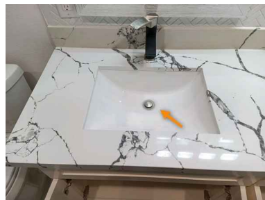
Stuck, Primary Bathroom
