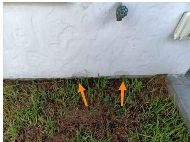
Damaged siding, rear
