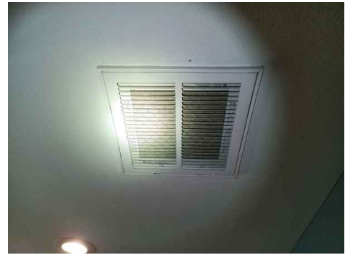
Dirty, primary bedroom
