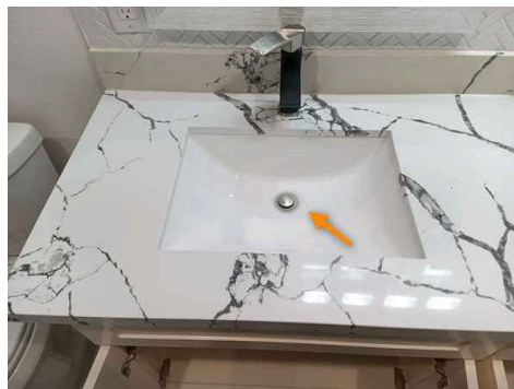
Stuck, Primary Bathroom
