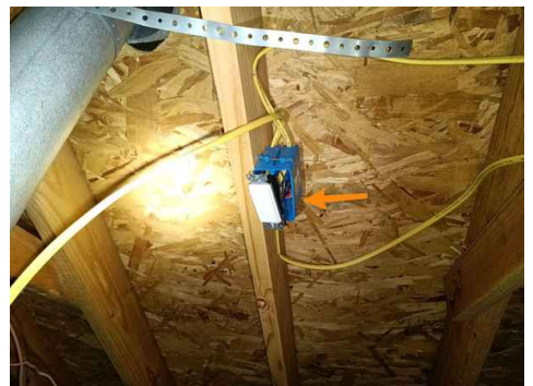
Loose, furnace switch
