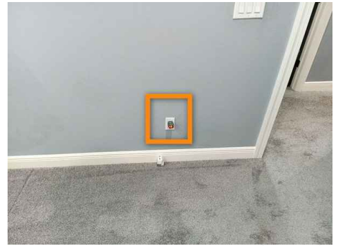
Hot / neutral reversed, second floor left bedroom
