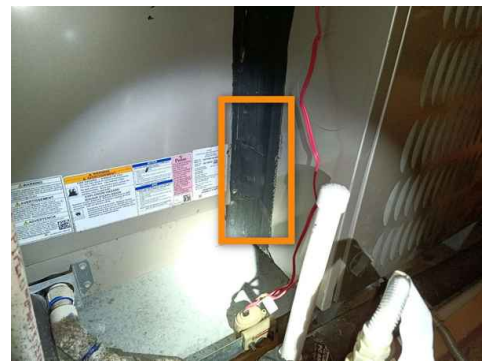
Air leakage, coil cabinet
