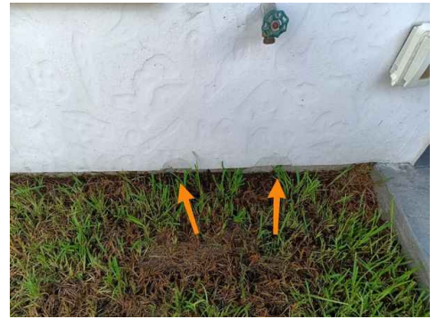
Damaged siding, rear
