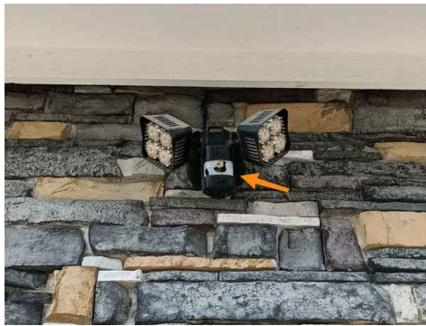
Damaged sensor, front
