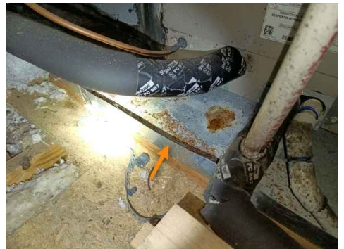
Corrosion, dry at time
