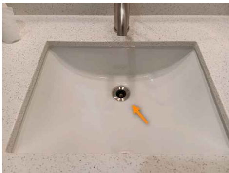
Missing stopper, half bathroom
