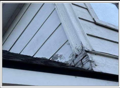
Rotted siding and trim
