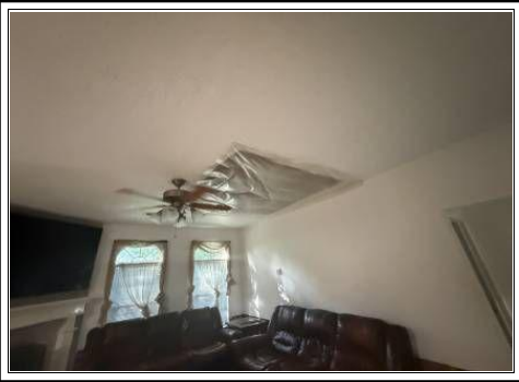
Missing sheetrock section in ceiling
