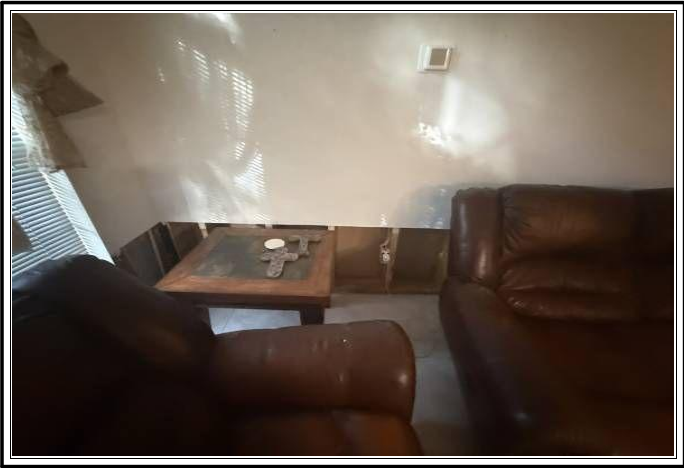
Missing lower section of sheetrock
