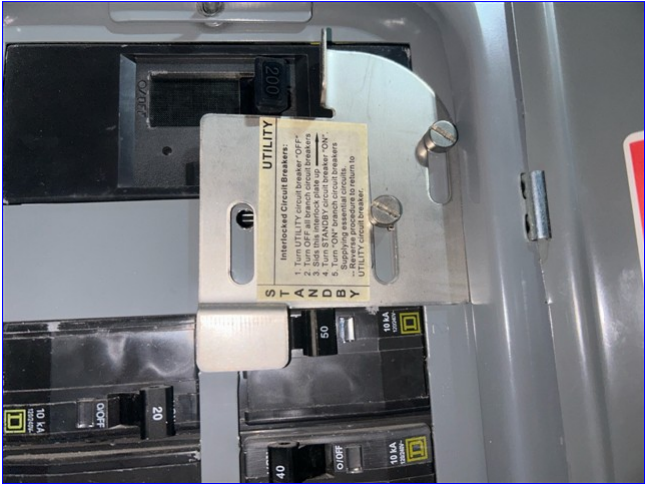
C. Item 1 (Picture) View of 50 amp generator interlock kit installed in breaker panel
