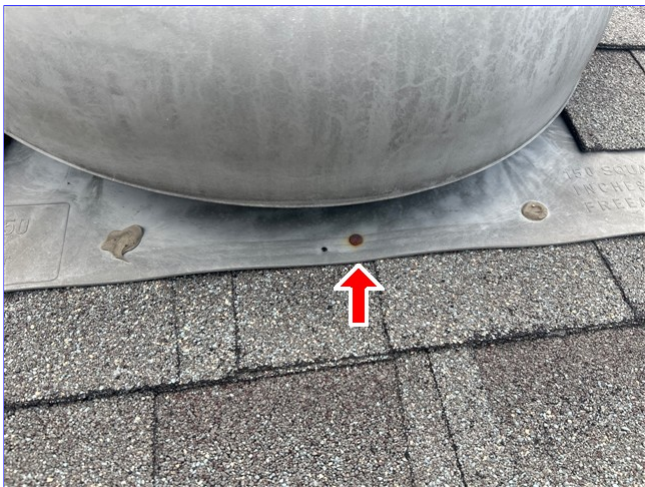
D. Item 1 (Picture) View of exposed nail head at passive roof vent
