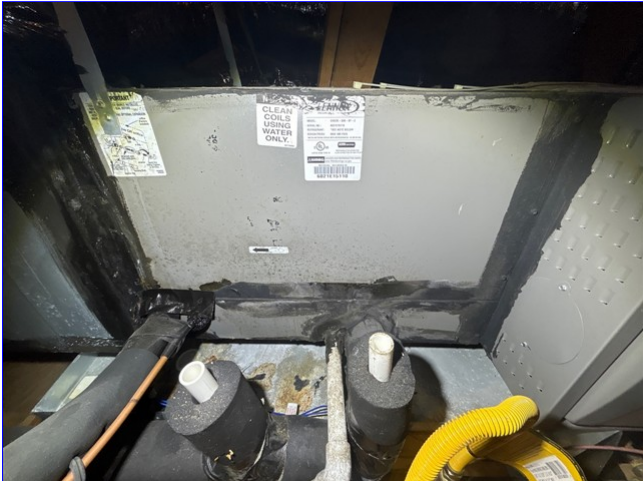
B. Item 13 (Picture) View of the cooling system 2 evaporator
