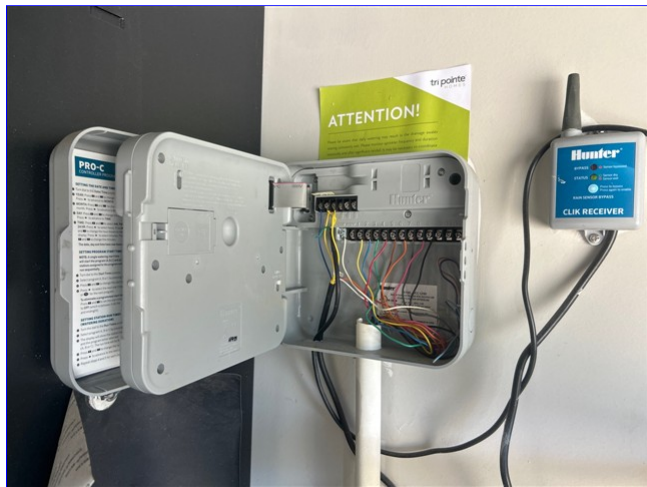
A. Item 1 (Picture) View of the sprinkler controller in the garage open for inspection
