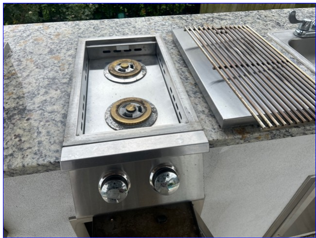
H. Item 1 (Picture) View of outdoor gas range unable to light the burners
