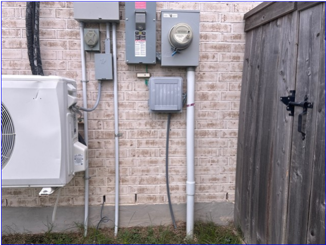
A. Item 7 (Picture) View of electrical service entrance equipment at right side of home
