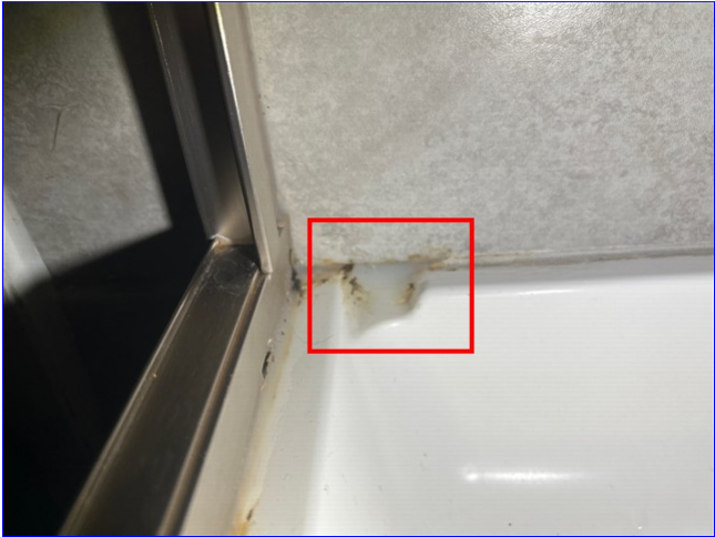
F. Item 1 (Picture) View of block weep holes in the second floor jack and jill bathroom shower enclosure
