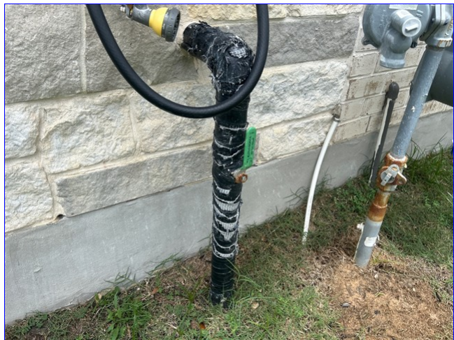
A. Item 2 (Picture) View of the main water shutoff at the right side of the home
