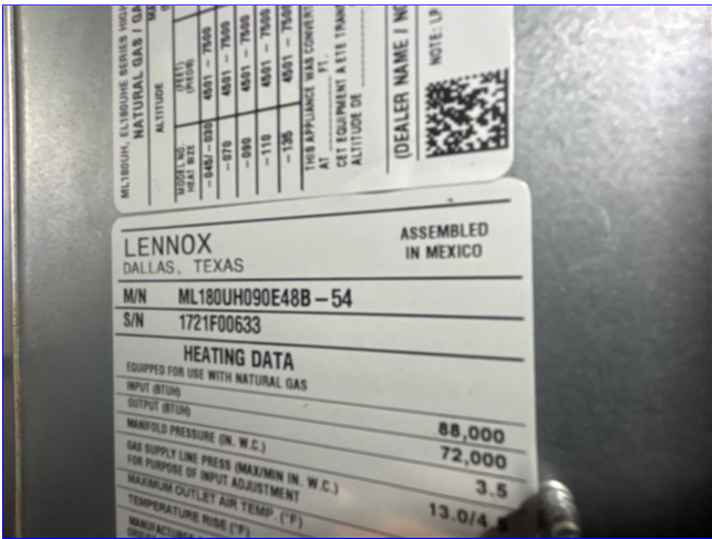
A. Item 6 (Picture) View of furnace 2 data plate
