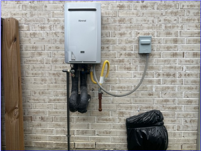
C. Item 1 (Picture) View of the water heater
