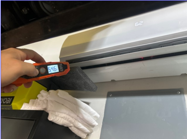
B. Item 4 (Picture) View of the measured temperature of the cooled air produced by the mini split
