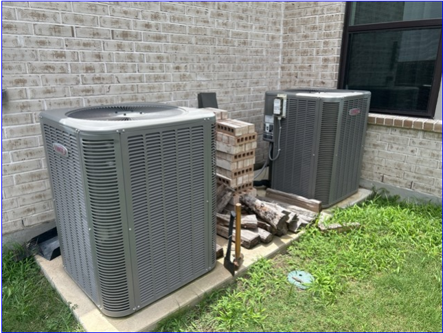
B. Item 8 (Picture) View of the cooling systems condensing units
