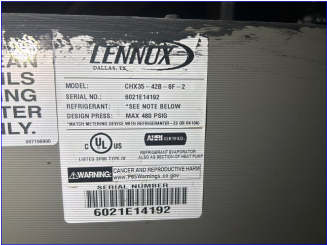
B. Item 12 (Picture) View of the cooling system1 evaporator data plate
