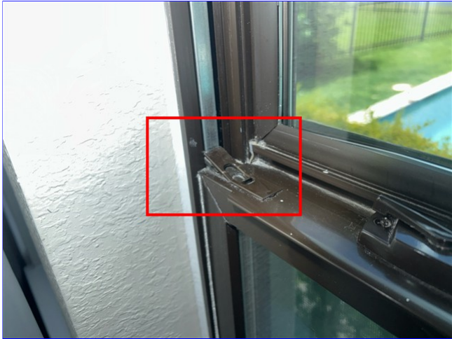
H. Item 1 (Picture) View of broken window tilt lever
