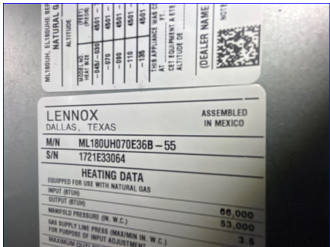
A. Item 4 (Picture) View of furnace 1 data plate
