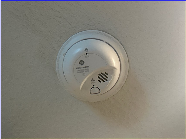
B. Item 3 (Picture) View of combo smoke and CO detector installed in home
