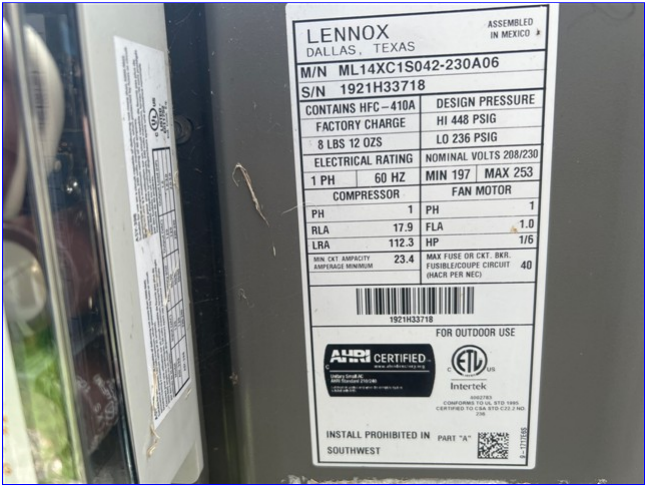
B. Item 9 (Picture) View of the cooling system 1 condenser data plate
