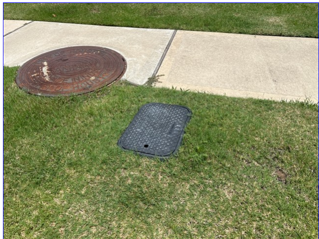
A. Item 1 (Picture) View of the water meter
