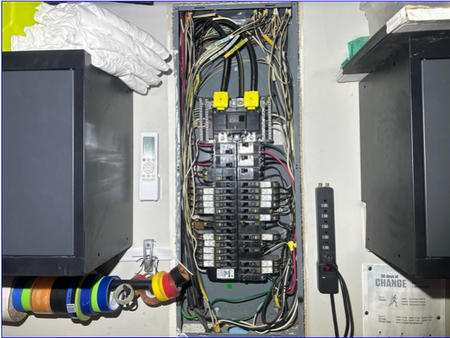
A. Item 4 (Picture) View of breaker panel open for inspection
