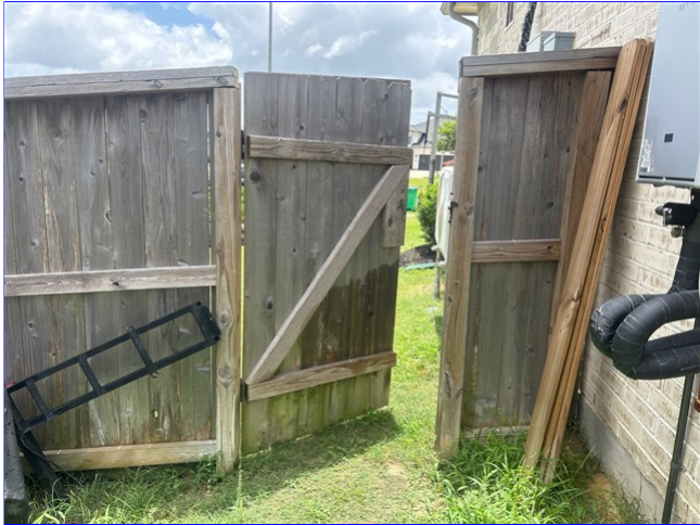
L. Item 1 (Picture) View of privacy fence gate not self closing or latching
