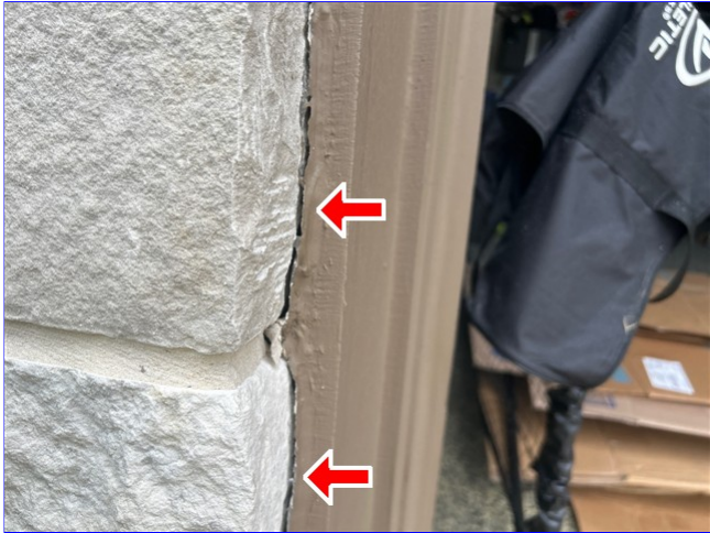
E. Item 1 (Picture) View of brick veneer to garage door frame transition not sealed
