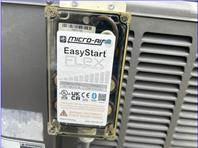
D. Item 1 (Picture) View of soft start kit installed on cooling system condenser
