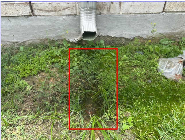
B. Item 1 (Picture) View of gutter downspout missing splashblock and washed area
