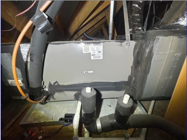
B. Item 11 (Picture) View of the cooling system 1 evaporator
