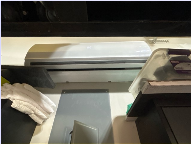
B. Item 5 (Picture) View of the interior component of the mini split
