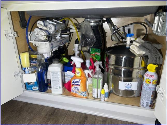
F. Item 3 (Picture) View of drinking water filtration system installed under kitchen sink
