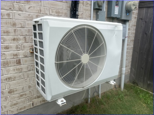
B. Item 6 (Picture) View of the outdoor component of the mini split
