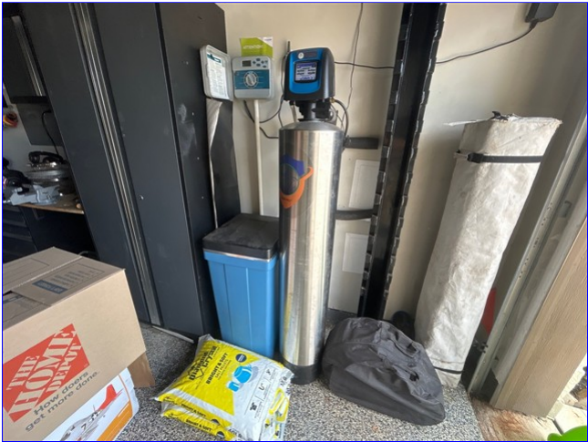
F. Item 2 (Picture) View of water softener installed in garage
