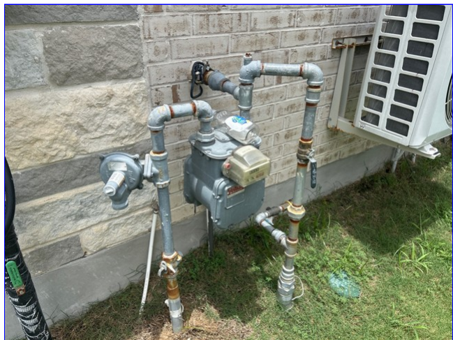
E. Item 1 (Picture) View of the gas meter at the right side of the home
