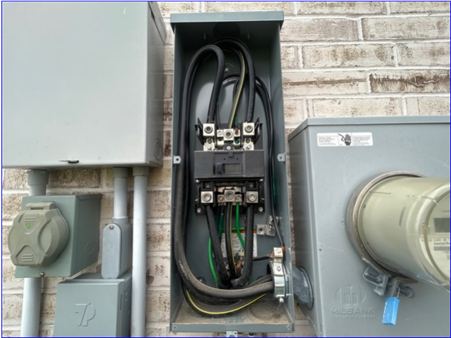
A. Item 6 (Picture) View of service disconnect open for inspection
