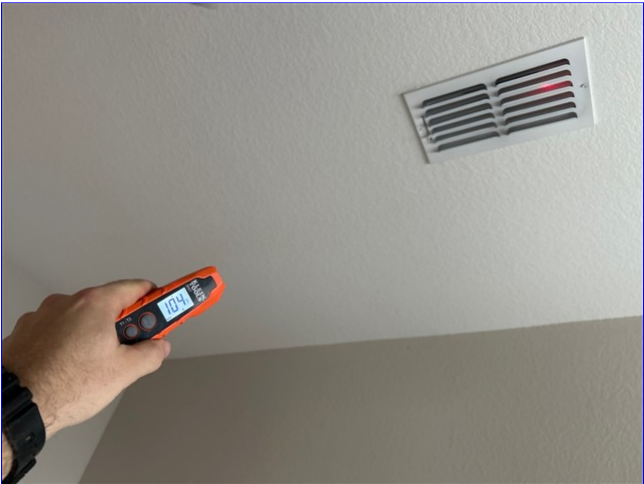
A. Item 1 (Picture) View of the measured supply air temperature from heating system 2 at the 2nd floor supply register
