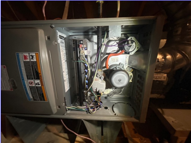
A. Item 5 (Picture) View of furnace 2 open and lit for inspection
