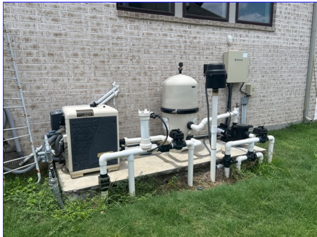
B. Item 1 (Picture) View of pool equipment installed at the right side of the home
