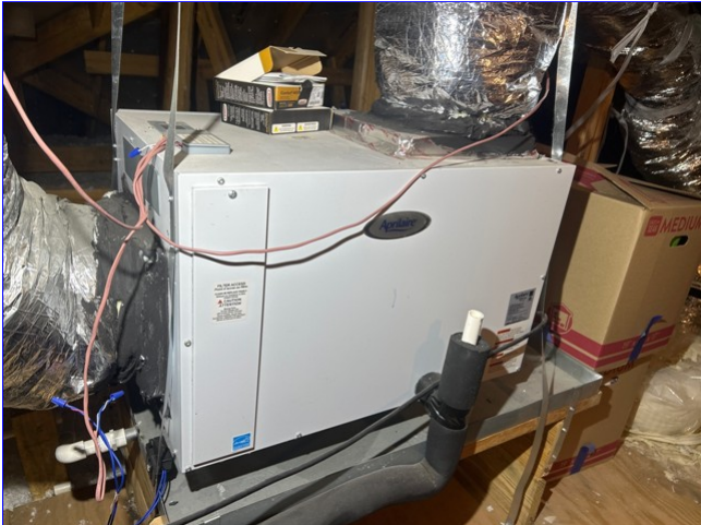
D. Item 2 (Picture) View of whole home dehumidifier installed in attic space
