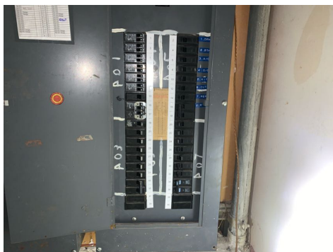
Exterior of subpanel located in electrical closet
