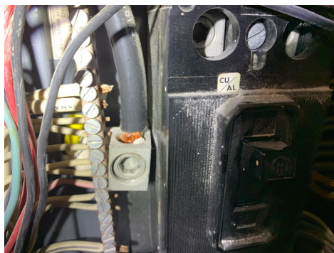
Copper feeder wires at subpanel located in electrical closet
