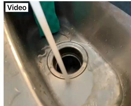
The unit has excessive noise/vibration
