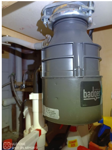
General Photos of Range Hood/Exhaust Systems:
