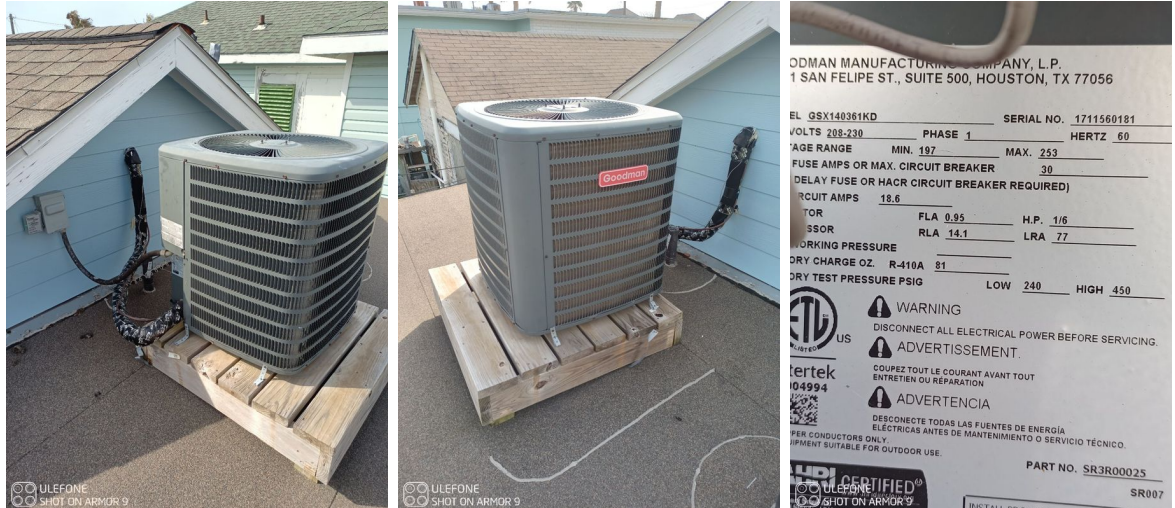
General Photos of HVAC Equipment:
