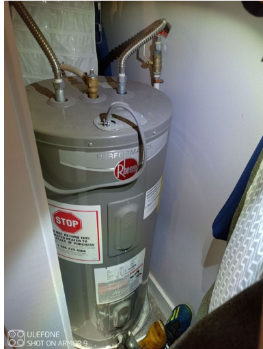
General Photos of Water Heating Equipment:
