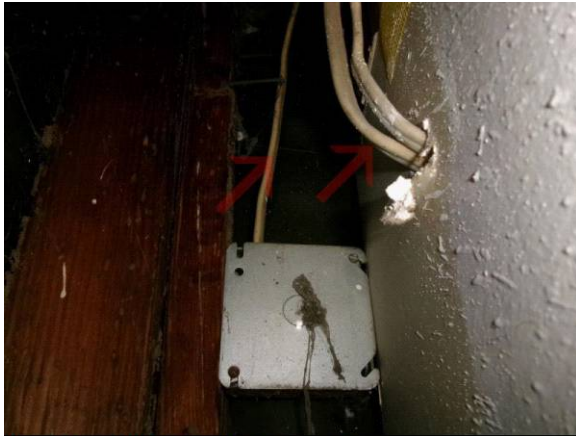
Improper wiring in the garage.
