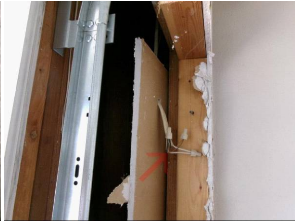
Improper wiring in garage.
