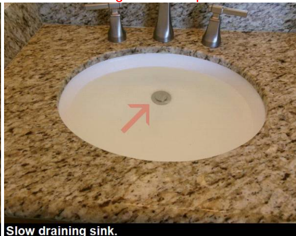
Slow draining sink.
