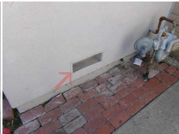
Vents missing inside of garage.
