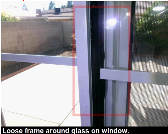
Loose frame around glass on window.
