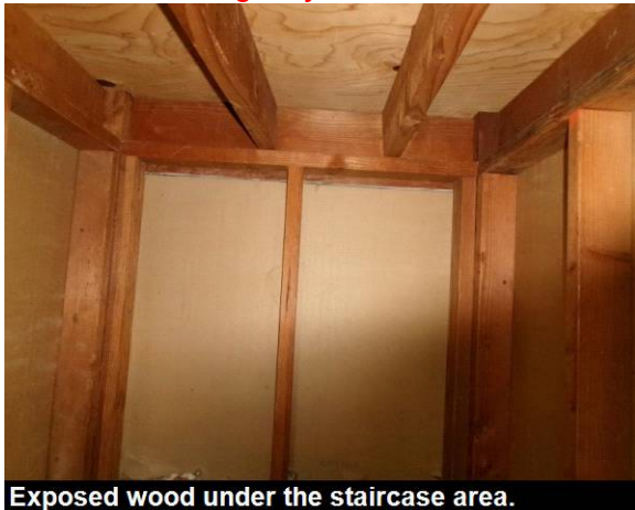
Exposed wood under the staircase area.
