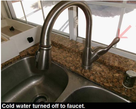
Cold water turned off to faucet.
