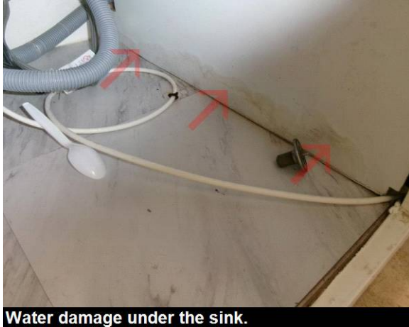
Water damage under the sink.
