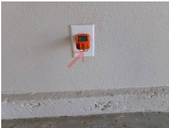
No power to receptacle.
