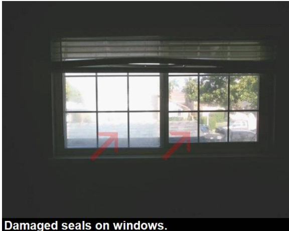
Damaged seals on windows.
