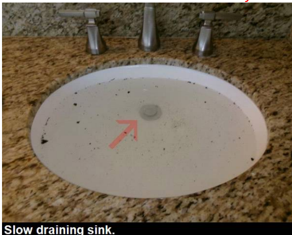
Slow draining sink.
