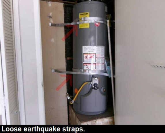
Loose earthquake straps.
