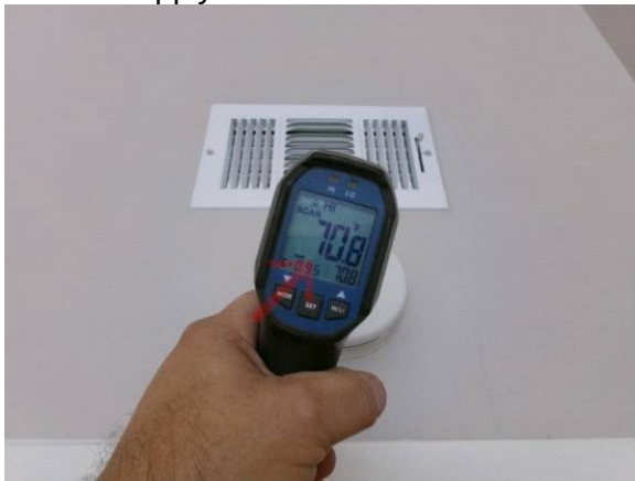
A/C cooling properly.
