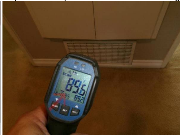
Upstairs air temperature, return air.
