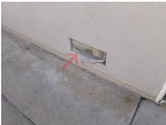
Vents missing inside of garage.
