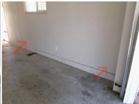
Vents missing inside garage on side wall.
