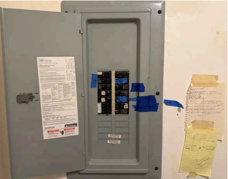
Laundry Area Sub-Panel
