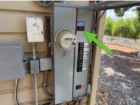
Front Left Exterior Main Panel
