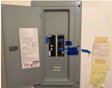
Laundry Area Sub-Panel
