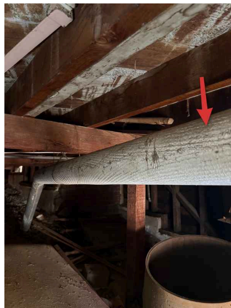
This additional pipe was also noted to have Tran in the crawlspace, but no longer appears to be in use
