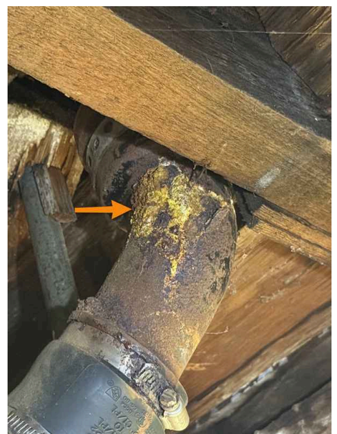
Example Noted at Crawlspace
