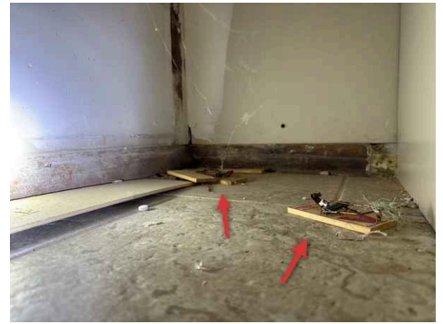
Example Noted at Kitchen
