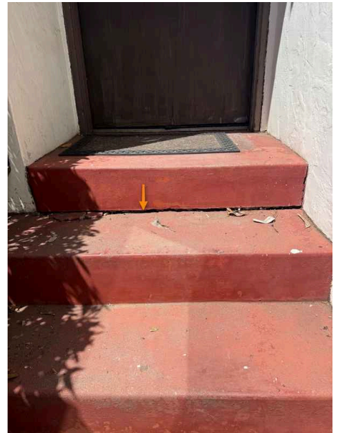
Example Noted at the front porch
