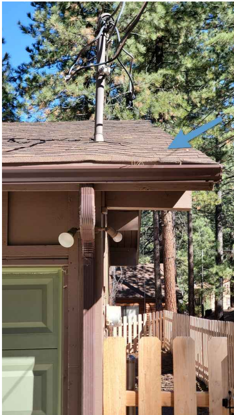
Looks to be a failure of the fascia and roof deck
