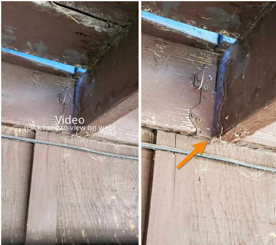
wrong type of hanger for purpose.
