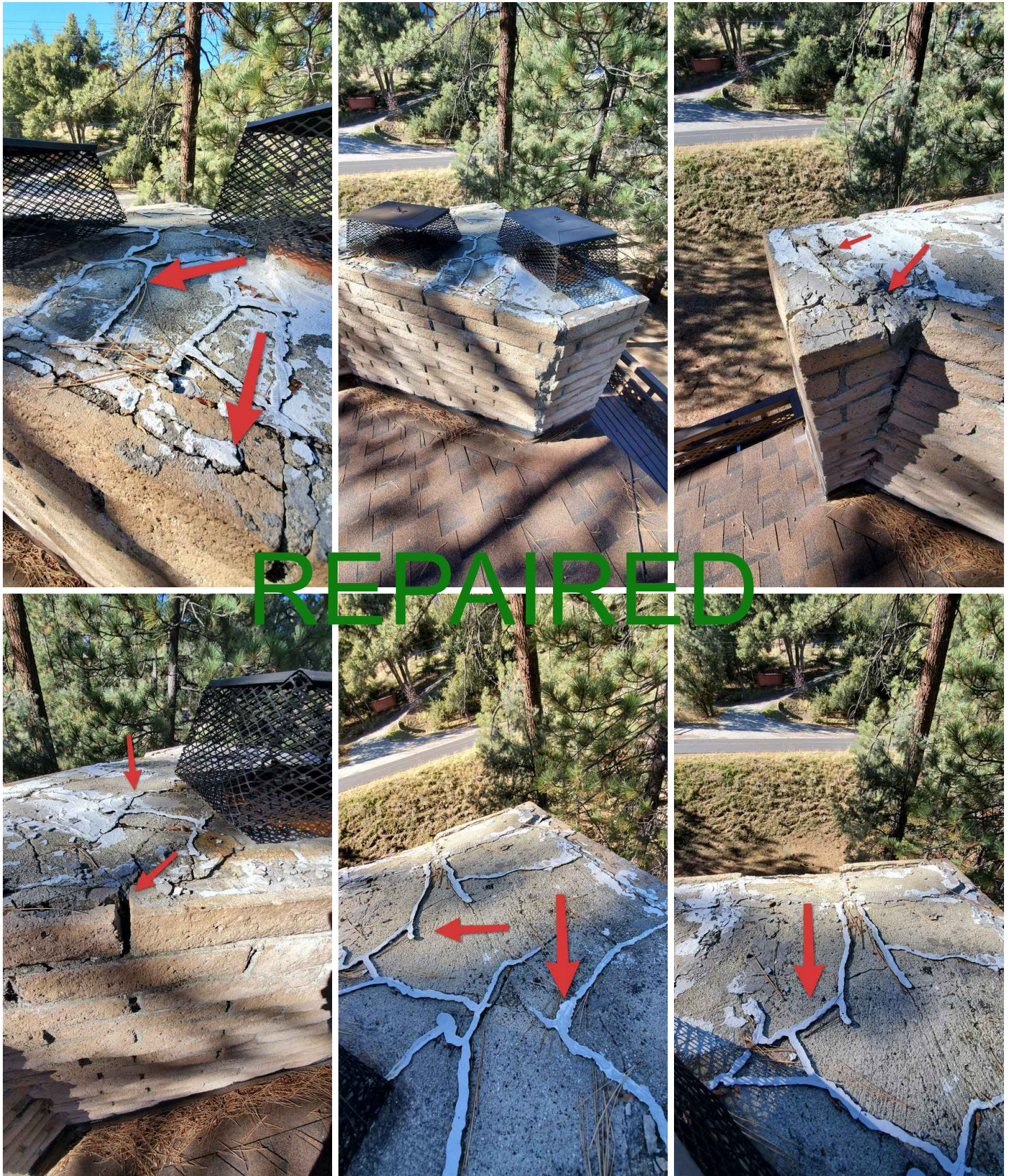
Failed caulking, inappropriate repair
