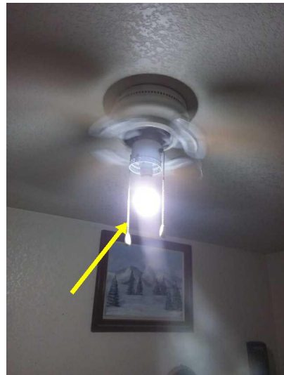
A light cover or globe is missing and should be installed.
