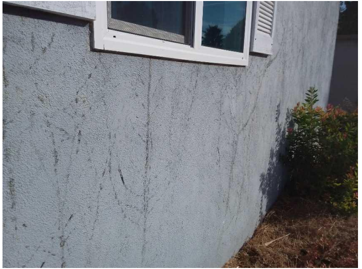
There are stains present that may be difficult to remove.
