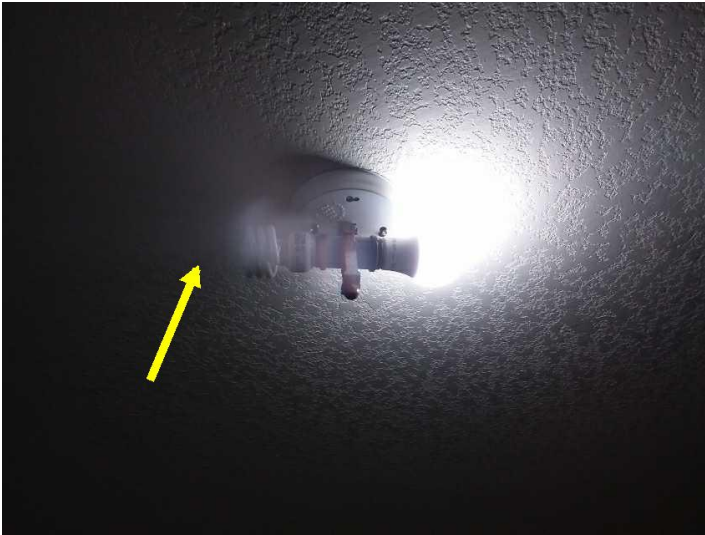
A ceiling light in the bedroom does not respond, and should be serviced.
