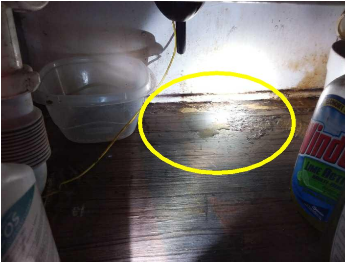
There is a leak below the sink, which should be repaired.
