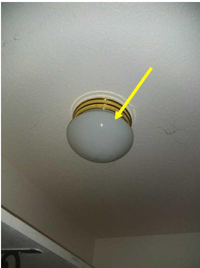
The light in the bedroom closet does not respond and should be serviced.
