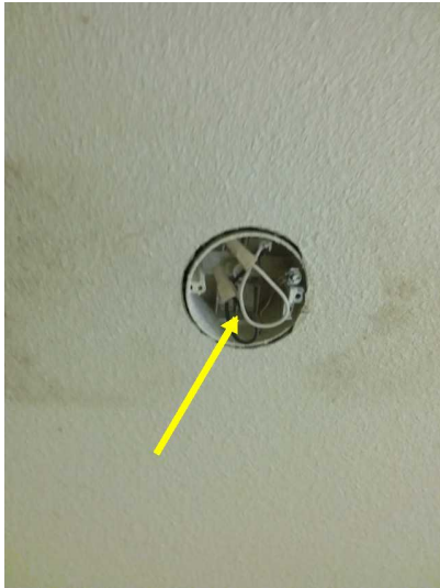
A ceiling light is missing which should be replaced or the electrical box sealed.
