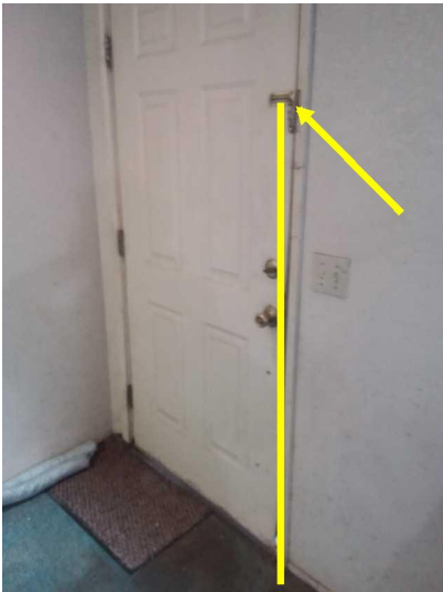
A secondary lock has been installed higher than 48 inches which could impede the exit of a child or short person.
