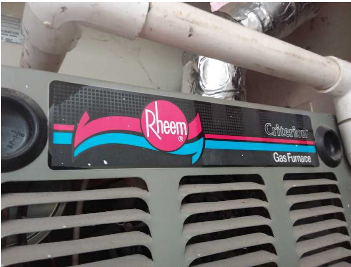
Serial number for furnace in stair closet BR5D302 F1892 6229 - MANUFACTURED 1992
