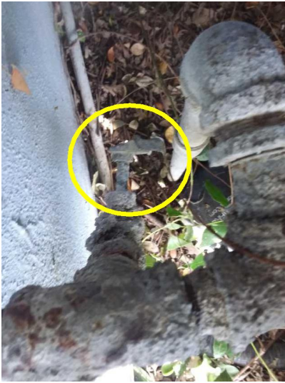
The main water shut off valve handle is missing or broken and it should be repaired.
