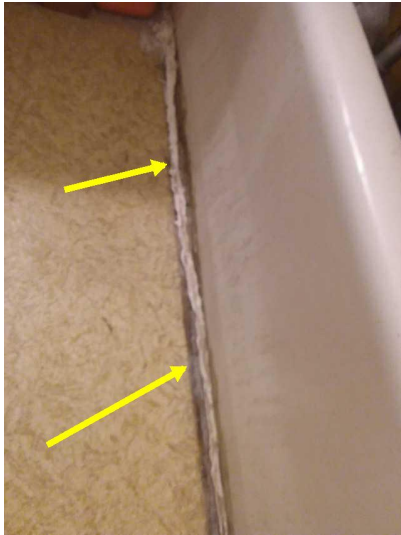
The vinyl floor is lifting where it meets the shower or tub and should be sealed.
