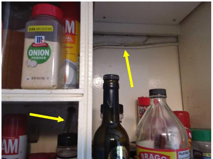
There is exposed romex or electrical cabling that should be protected by installing the romex inside the wall cavity, or properly wired into conduit.
