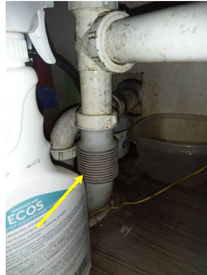
The sink employs an unconventional flexible drainpipe that could contribute to blockages.
