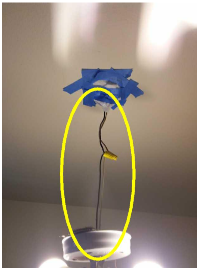
A ceiling light is loose or missing which should be replaced or the electrical box sealed.
