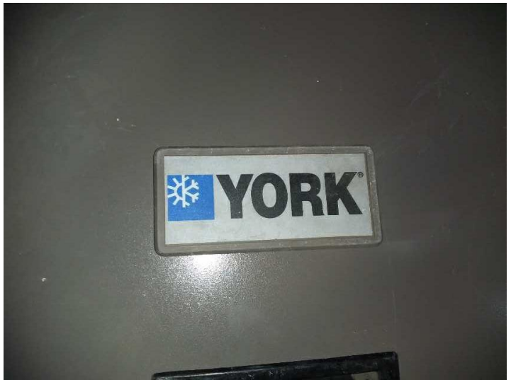
Central heat is provided by 2 forced-air furnaces that are located in crawlspace and stair closet.
