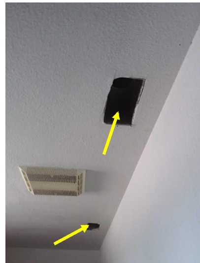
A wall register is missing in bathroom and should be replaced.
