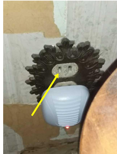
The ungrounded and obsolete outlets in the living room should be upgraded to include more modern and safer ones, which provide a pathway for the current to travel harmlessly to ground.
