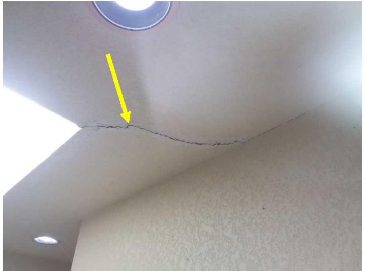
The walls have stress fractures which may have resulted from movement. I can elaborate on this issue, but you should have a specialist comment, and be aware that such cracks can reappear, and typically if they are not repaired correctly.
