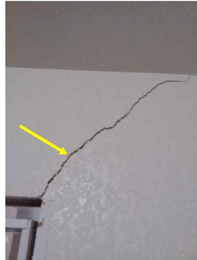
The walls have stress fractures which may have resulted from movement. I can elaborate on this issue, but you should have a specialist comment, and be aware that such cracks can reappear, and typically if they are not repaired correctly.
