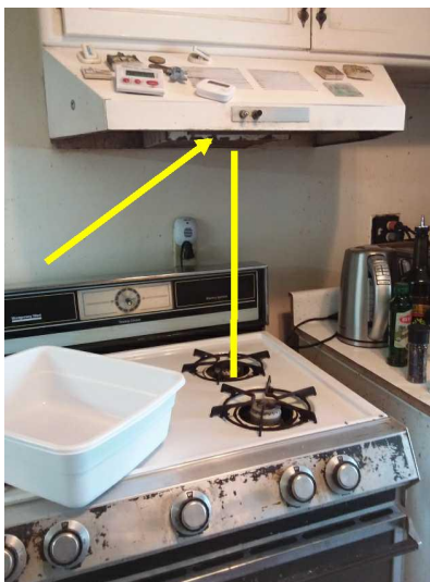
The range hood exhaust-fan is closer than the recommended 24 inches and should be used with caution.
