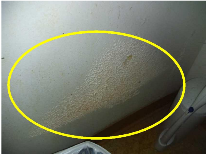
There is a moisture stain on the wall that should be explained by the sellers or further evaluated as to its cause.
