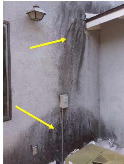
There are separations or nail-pops on the siding that need to be serviced/sealed.
