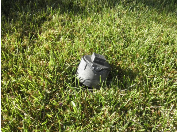
The main clean out cap is broken in the front yard.
