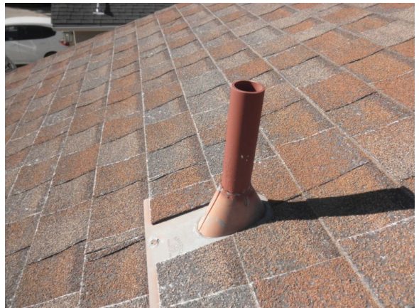
Deteriorated sealant at the vent flashings.
