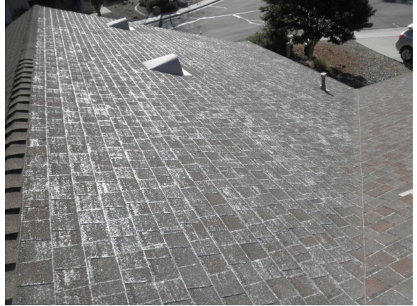
General deterioration of the roof shingles due to age.
