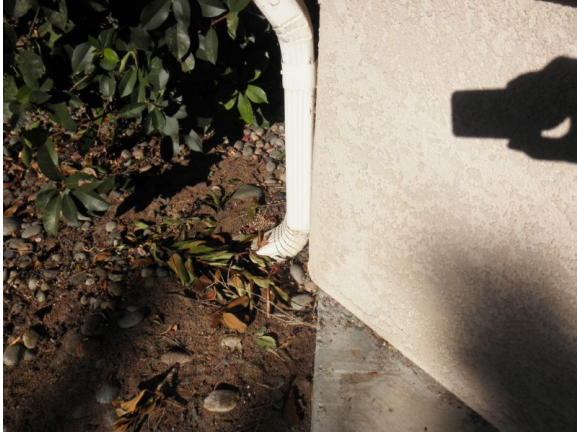
Some of the down spouts need to be directed away from the foundation.
