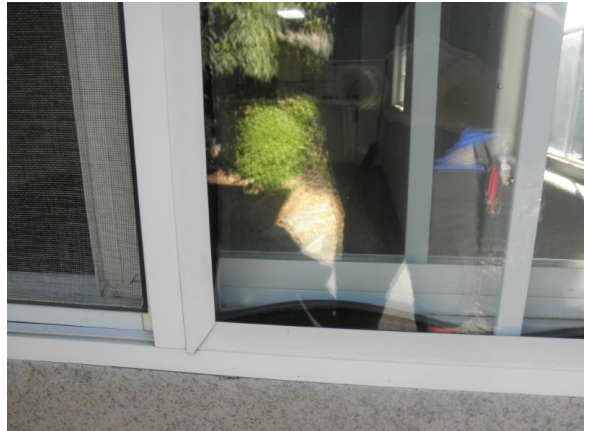
Example of the manufacturing defects at the windows.
