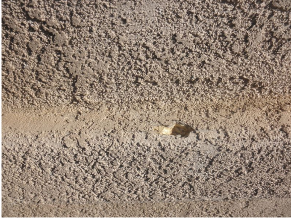
Minor damage to the stucco reveal on the south side of the garage.
