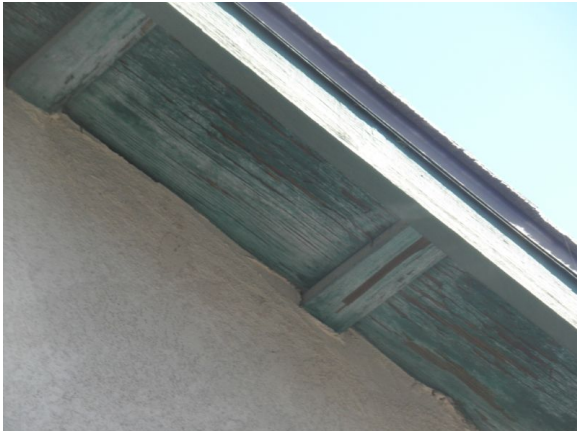
Parts of the eaves are in need of painting.
