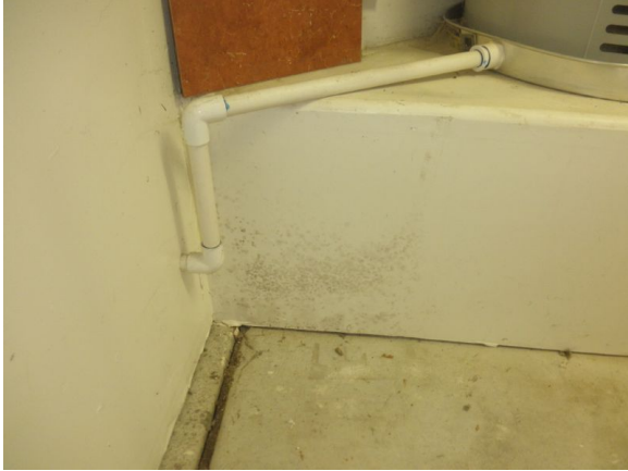
Black mildew like substance on the water heater platform.
