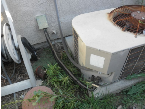
Deteriorated insulation on the low-pressure refrigerant line.
