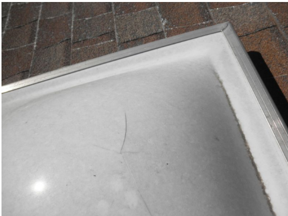
Cracked skylight above the hallway.
