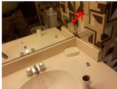
Not GFCI protected - improper
