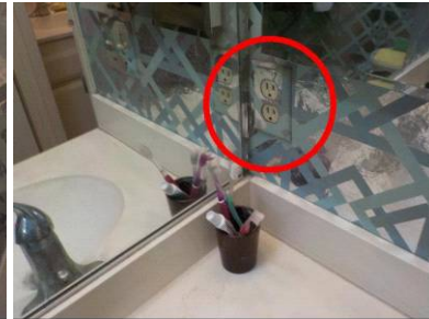
Not GFCI protected - improper
