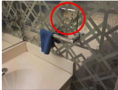
Not GFCI protected - improper
