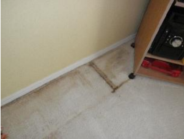
Old leak at the SW bedroom.
