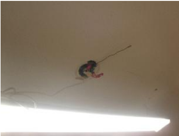
Spliced exposed wires in the garage.
