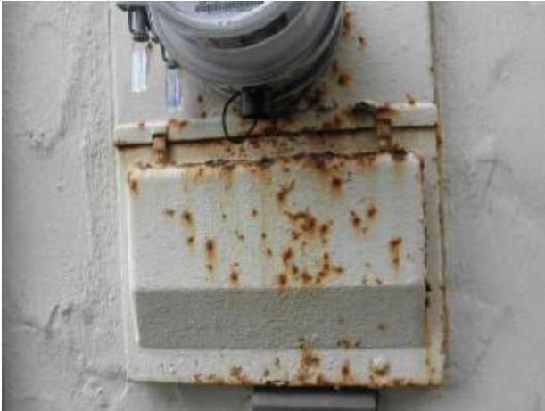
Rust damage at the main electrical panel.
