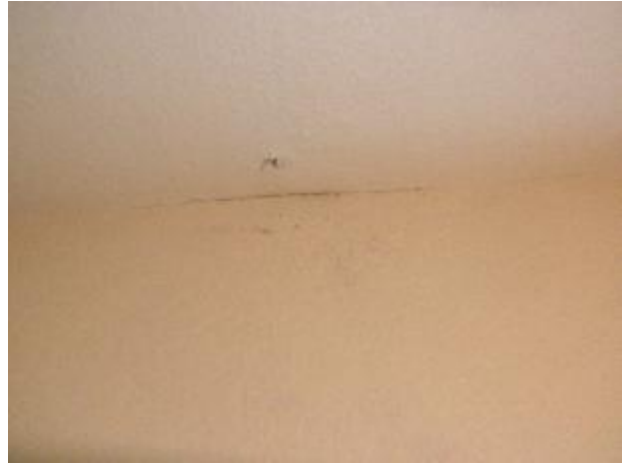
Active leak in the master bathroom above the toilet from the exterior siding.
