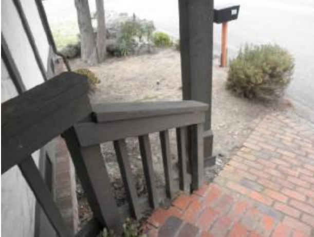
Nongraspable railing at the front entry.
