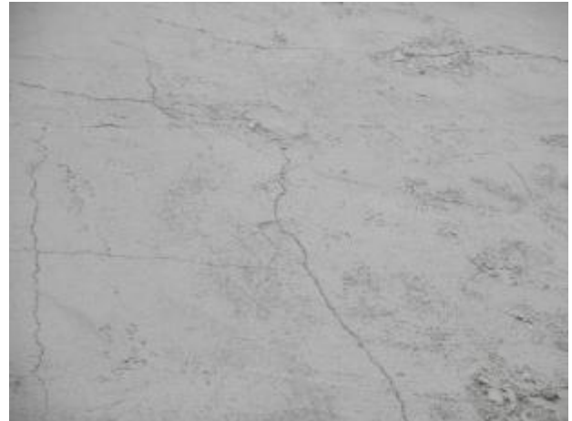
Excessive cracking at the stucco SE wall.
