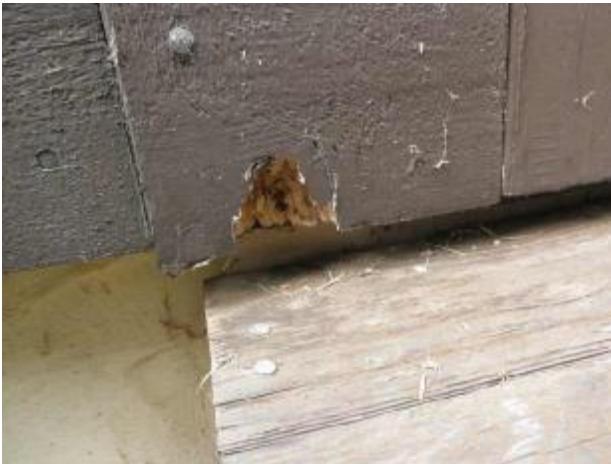
Example of moisture damage at the wood trim.
