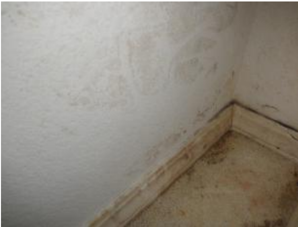
Evidence of a leak at the south bedroom closet with black mildew like substance.
