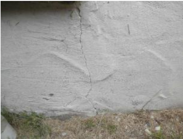
Excessive cracking at the stucco SE wall.
