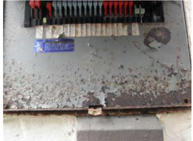
Rust damage at the main electrical panel.
