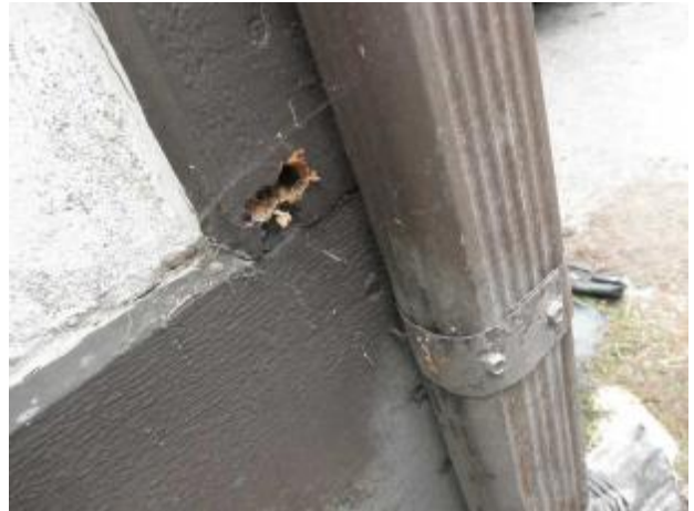
Moisture damage at the wood trim.
