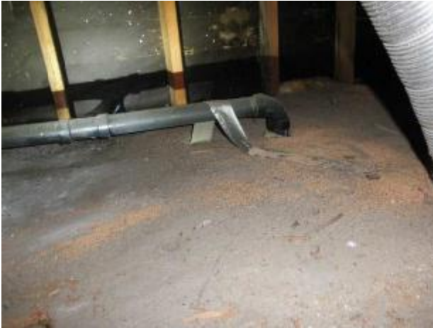
Evidence of termites in the attic space.
