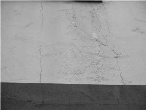
Excessive cracking at the stucco SE wall.
