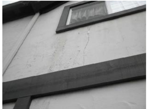
Excessive cracking at the stucco SE wall.
