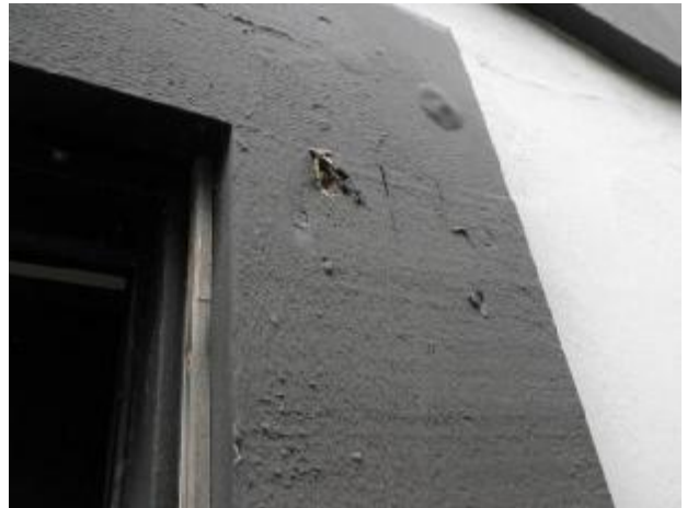
Moisture damage at the garage side door trim.
