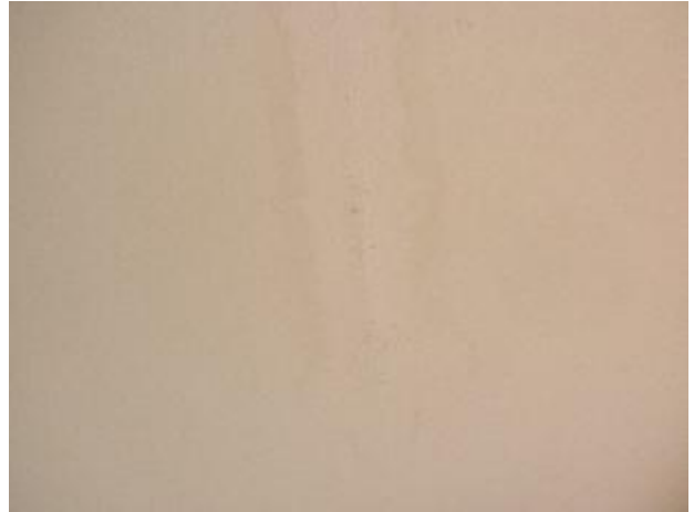
Water stain in the garage.
