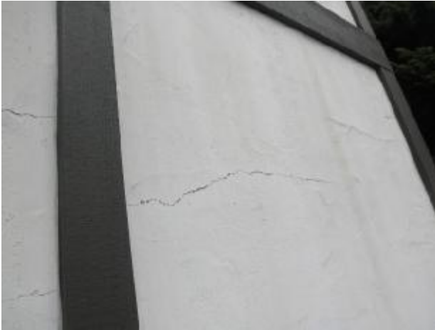
Excessive cracking at the stucco SE wall.
