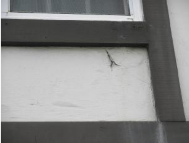
Damage to the stucco siding below the master bedroom window.
