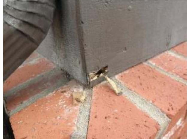
Example of termite damage to the wood trim.
