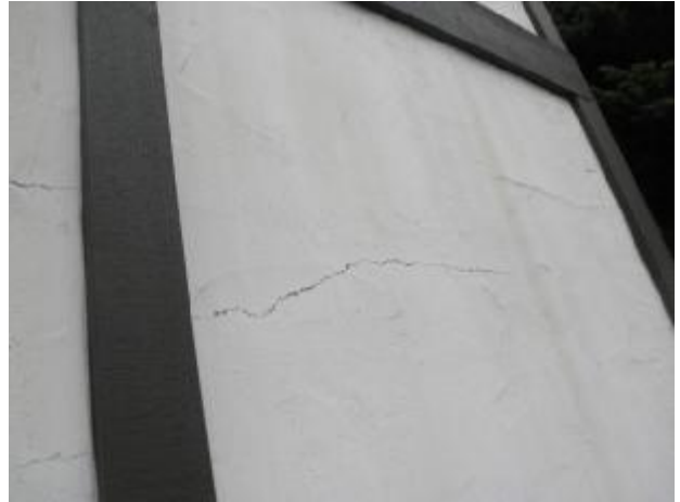
Excessive cracking at the stucco SE wall.
