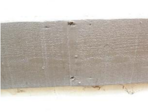
Example of moisture damage to the exterior wood trim.
