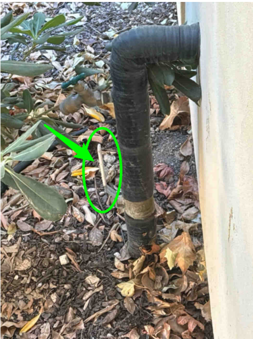
Main water shutoff valve
