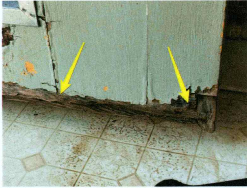
Damaged wood door
