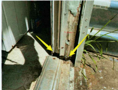
Damaged door jam
