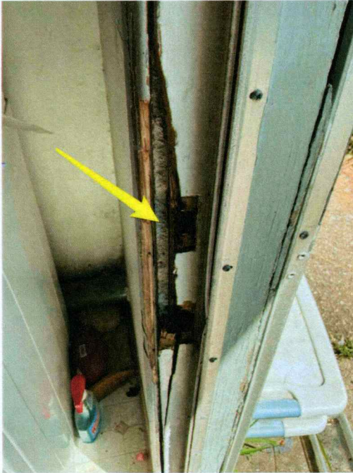
Damaged door frame
