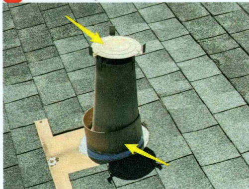
Broken furnace vent cap at roof needs replacement
