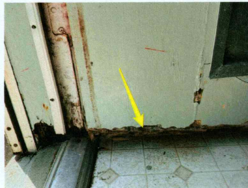
Damaged wood door
