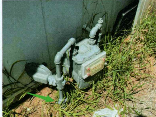
main gas shut off valve
