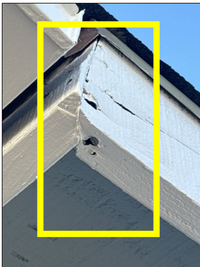
Moisture damage, wood rot, observed.
