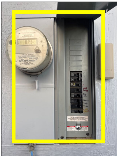
Main electrical service panel to the home.
