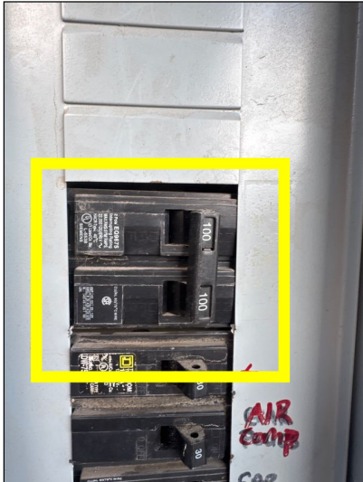
Main electrical shut off to the home
