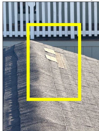
The roof had loose and/or missing shingles.
