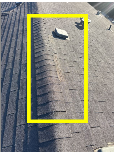
The roof had loose and/or missing shingles.
