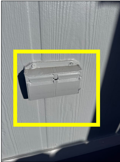
The exterior electrical receptacle was painted shut.
