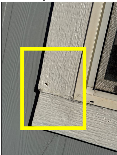
Moisture damage, wood rot, observed.
