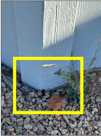
Moisture damage, wood rot, observed.
