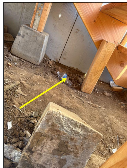
The home had areas of neutral or negative drainage that will route runoff from precipitation toward the foundation.
