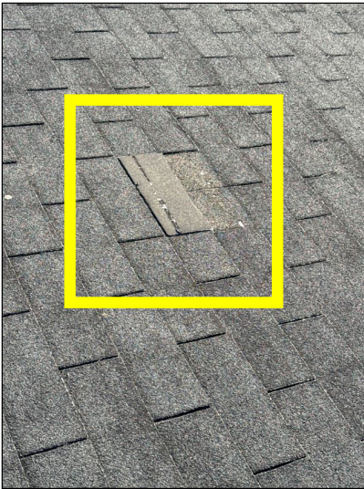
The roof had loose and/or missing shingles.
