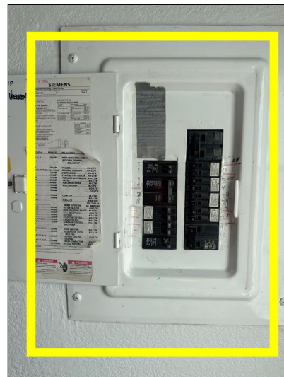
Sub panel to the home
