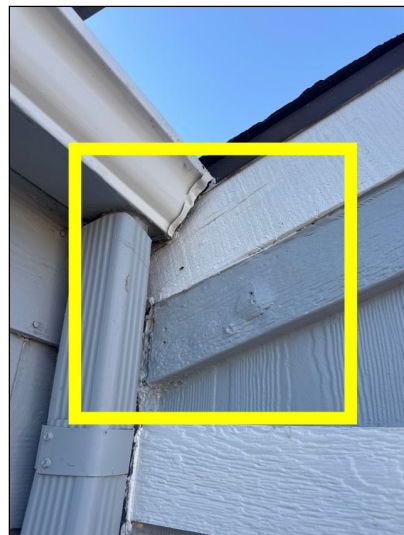
Moisture damage, wood rot, observed.
